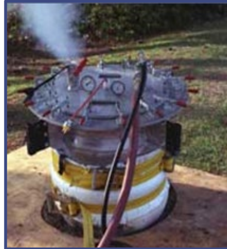
Steam exiting the vent pipe
