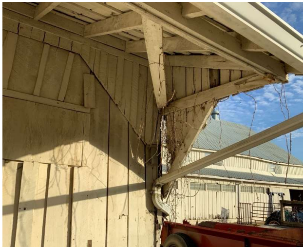
Overhead support diagonal is disconnected at the base and overhang is leaning (REF Photo S140)
