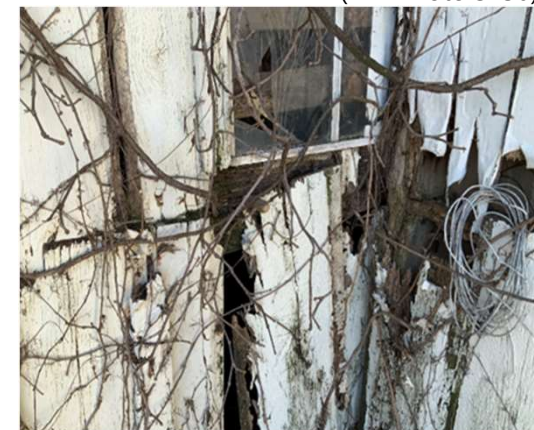
Rot and deterioration and over-growth at grade (REF Photo A16)
