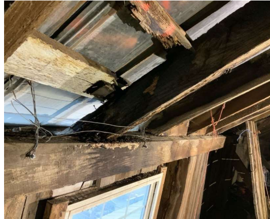
Rotting rafters (REF Photo S10)
