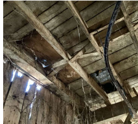
Hayloft from below – typical rotting/broken/missing floorboards – Lean-on structure (REF Photo S68)
