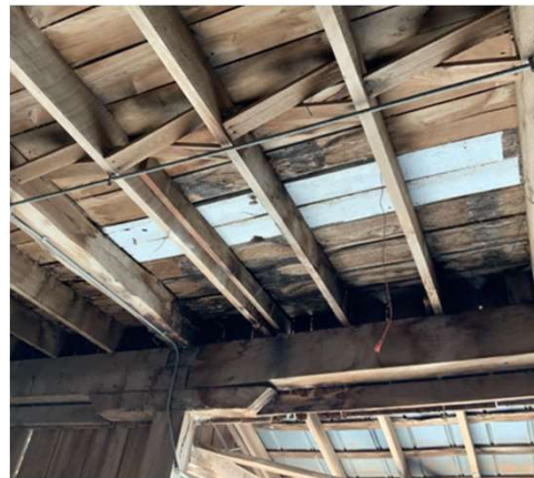
Typical rotting floorboards. East wing near Gridline 4 shown looking south (REF Photo S66).
