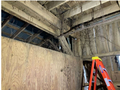
Critical finding at floor beam between Columns B/4 and C/4. West end of beam has approximately 90% section loss (REF Photo S80)
