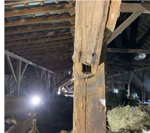
Disconnected and twisted east brace at Column M/3 in hayloft (looking west) REF Photo S47
