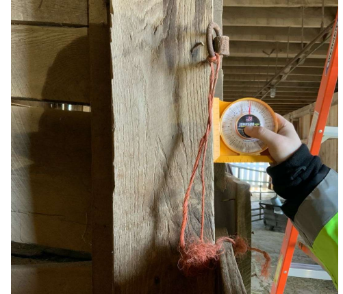
Column E/2 at grade level is leaning up to 6 degrees toward the south (REF Photo S101)
