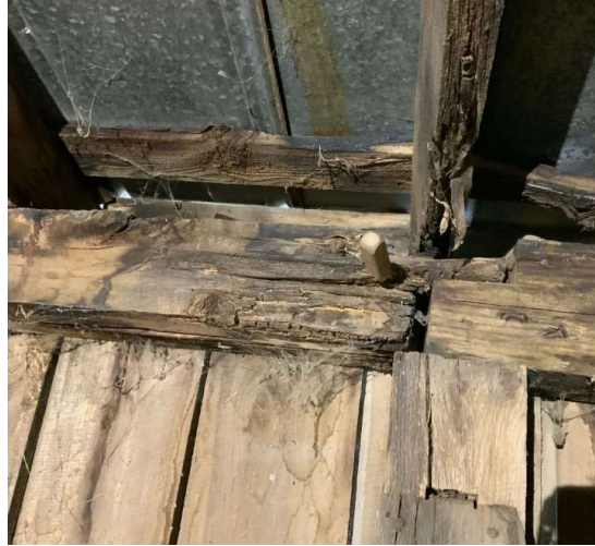
Perimeter roof rot (REF Photo S21)
