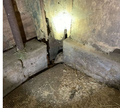
Bearing loss at Column M/2.5 at grade level (looking northwest) (REF Photo S107)
