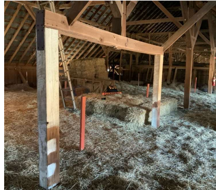
General view of the load spreader beam structures in hayloft (REF Photo G10)
