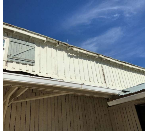
Sections of lifted metal roof panels and missing fascia boards (REF Photo A3)
