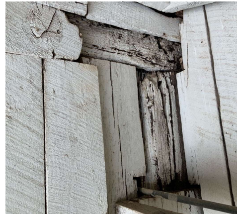
South face of the at-grade column cap at Column K/7 is exposed to exterior and has soft rot (REF Photo S97)
