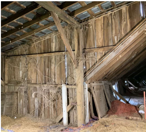
New column and posts supporting wind girt and roof beam at Column H/4 in hayloft (looking southwest). Note the south brace is connected with ineffective strap to new column. REF Photo S40
