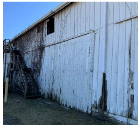
Gutter clogged with vegetation, deteriorated boards and discontinuous rain leader (REF Photo A14)
