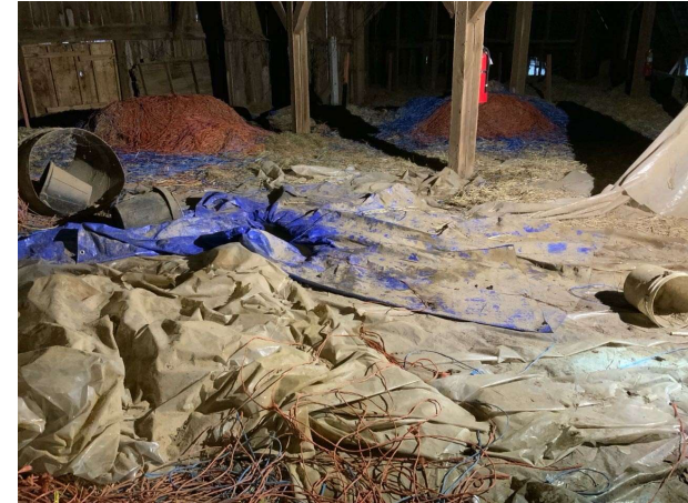
Tarps with standing water on hayloft flooring underneath lean-on region of structure. Floor shown looking northwest along gridline 6. (REF Photo S2)
