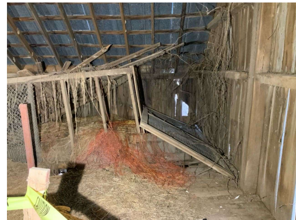
The east brace at Column B/4 in hayloft appears to be missing based on similar geometry in other portions of the building (looking south). REF Photo S51
