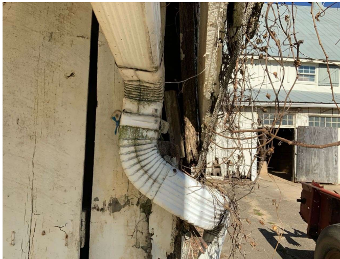
Detail photo of connection separation (REF Photo S141)
