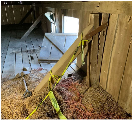
Perimeter roof beam twisting on split column at hayloft Level Near D/1. | REF Photo S15
