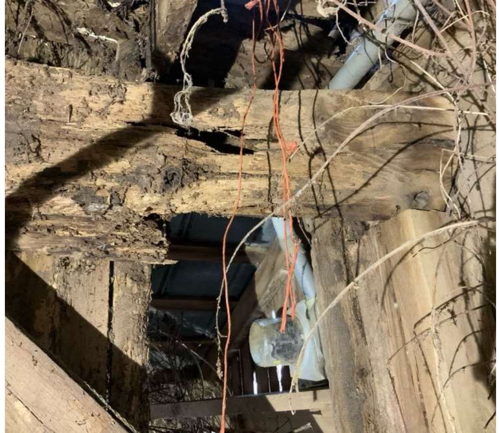
Critical finding at hayloft floor beam – west end of beam has approximately 90% section loss (REF Photo S81)
