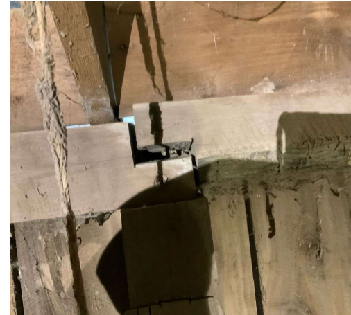
Perimeter roof beam between Column C/4 and D/4 is twisting 9 degrees south at east bearing and has minimal to no bearing remaining. REF Photo S16
