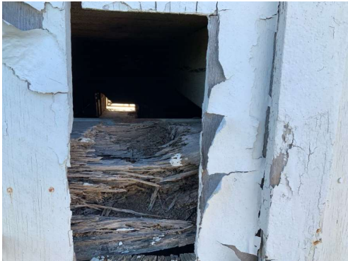
Severe rot at floor beam – west end has significant section loss (REF Photo S82)
