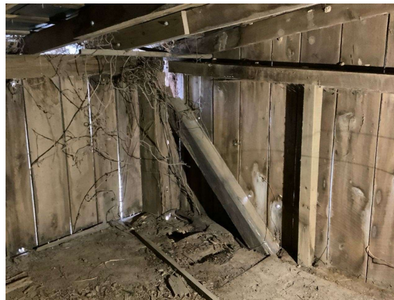
Severe rot at top of original Column H/7 in hayloft (looking southwest). A new post has been installed to the east of the existing column. The north brace and wind girt are not connected to the new post and east brace is missing. The floorboards adjacent to column are rotting. REF Photo S42
