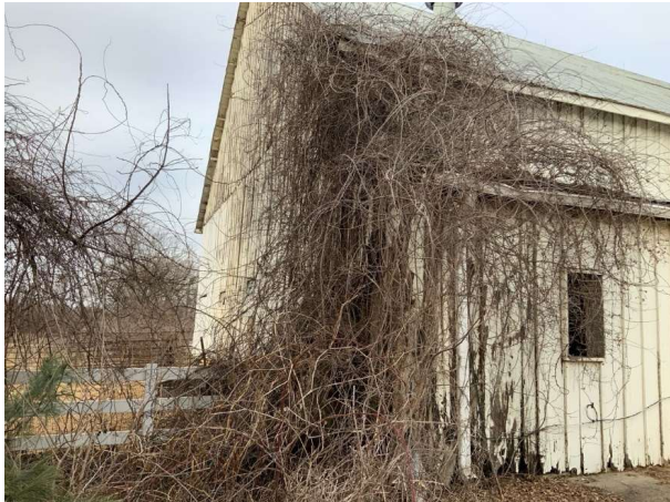
Heavy vegetation pushing up roof deck along southwest corner (REF Photo S113)
