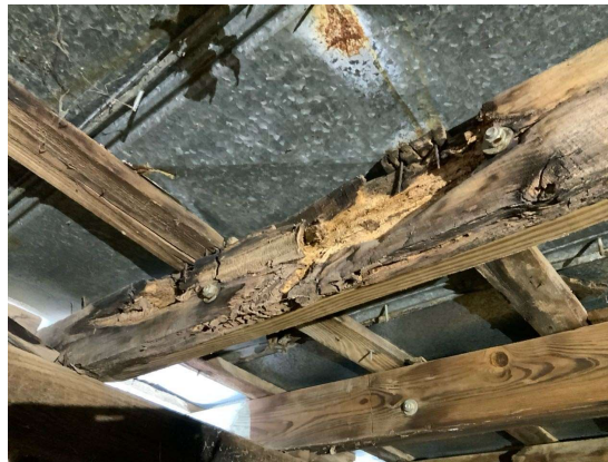
Previously sistered roof rafter along Gridline 7 between Gridlines I and J. Note the bolts are only through the rotted portion of the rafter. (REF Photo S12)
