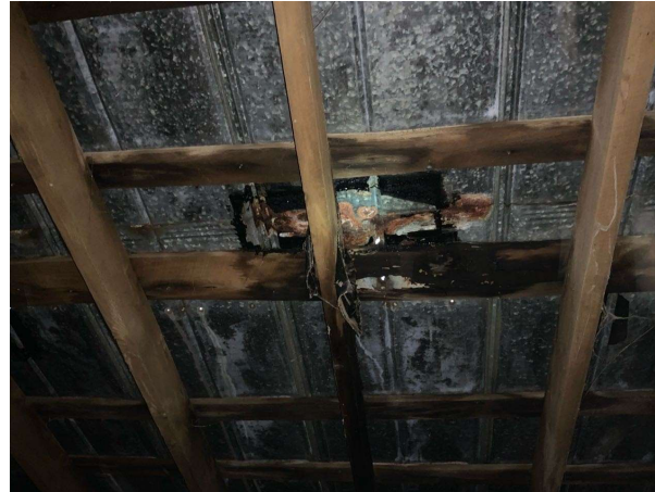
Typical area of rusted roof deck and failing patch (REF Photo S2)
