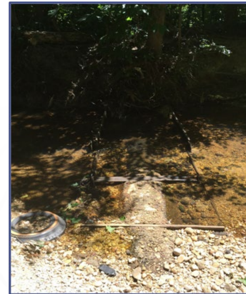
Exposed sewer pipes
