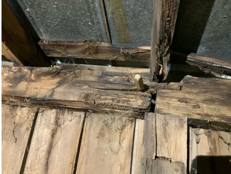
ES Photo 4 – Perimeter Roof Rot (REF Photo S21 – Appendix B2)
