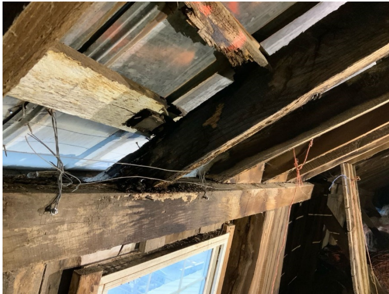
ES Photo 3 Rotting rafters (REF Photo S10 – Appendix B2)
