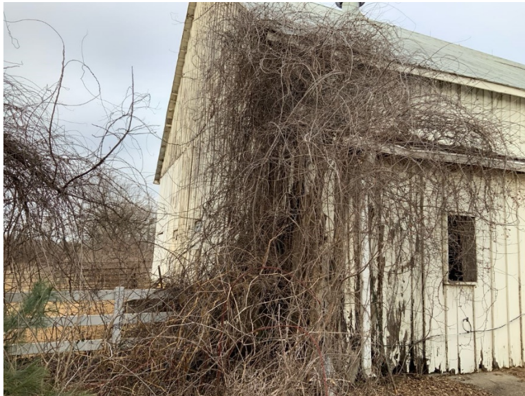
ES Photo 2: Heavy Vegetation pushing up roof deck along southwest corner (REF Photo S113)
