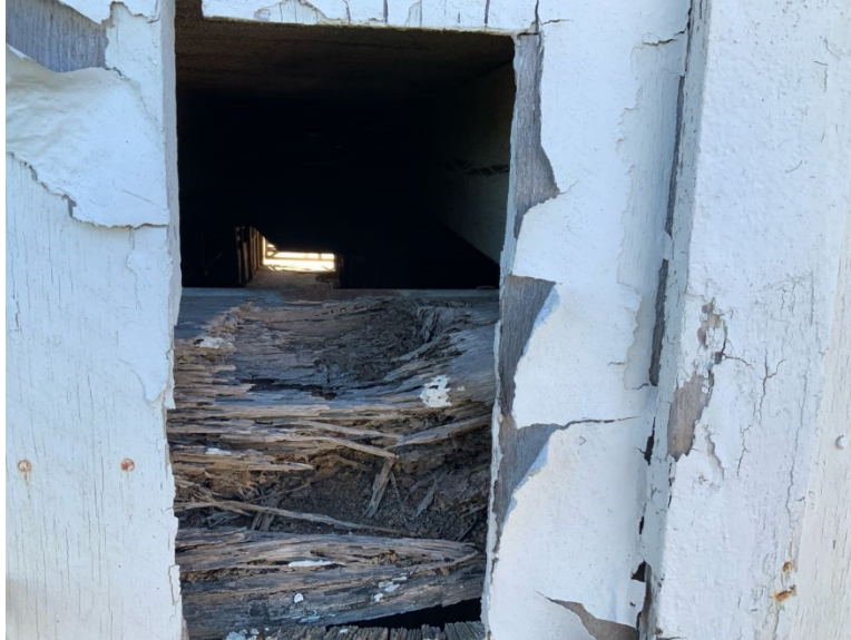
ES Photo 9 – Severe rot at floor beam – west end has significant section loss – (REF Photo S82 – Appendix B2)
