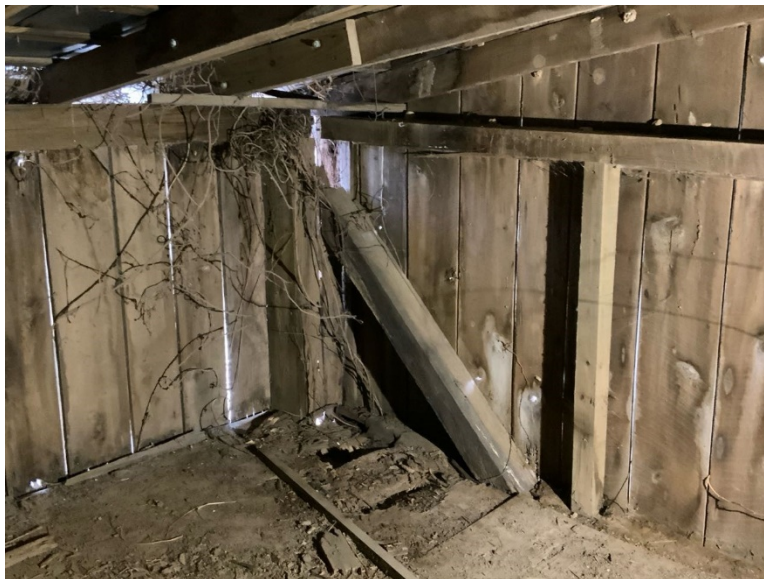
ES Photo 6 – Hayloft looking southwest – post has been added to east existing column., north brace and wind girt are not connected to the post and the east brace is missing. The floorboards adjacent to the column are rotting. (REF Photo S42- Appendix B2)
