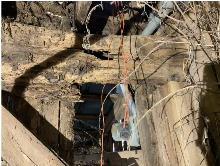
ES Photo 8 – Critical finding at hayloft floor beam – west end of beam has approximately 90% section loss – (REF Photo S81 – Appendix B2)
