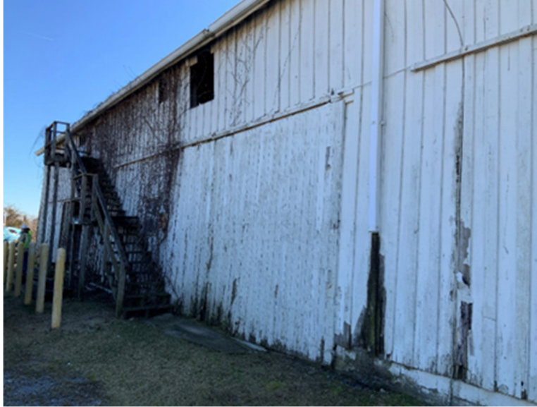
ES Photo 14 – Gutter clogged with vegetation, deteriorated boards and discontinuous rain leader (REF Photo A14 – Appendix B3)
