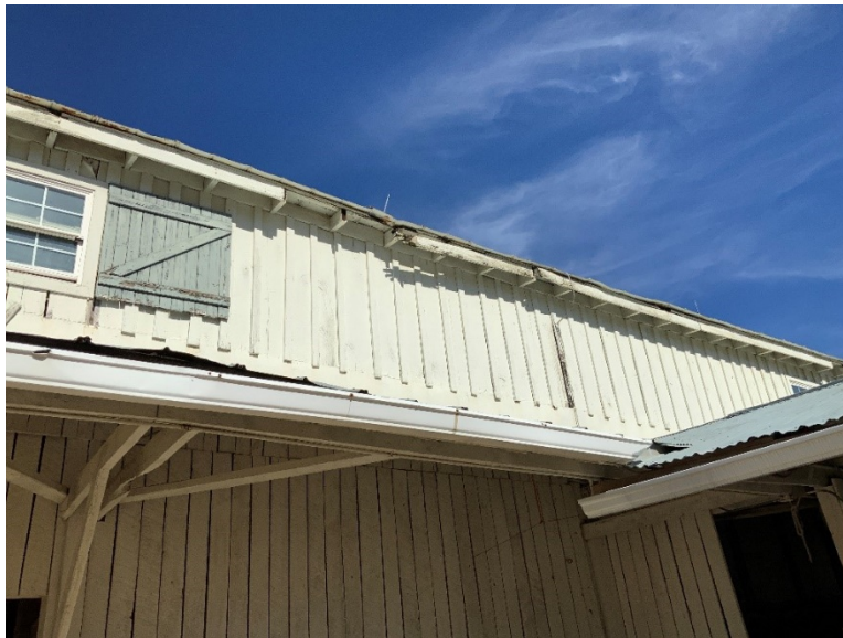
ES Photo 13 – Sections of lifted metal roof panels and missing fascia boards (REF Photo A3- Appendix B3)
