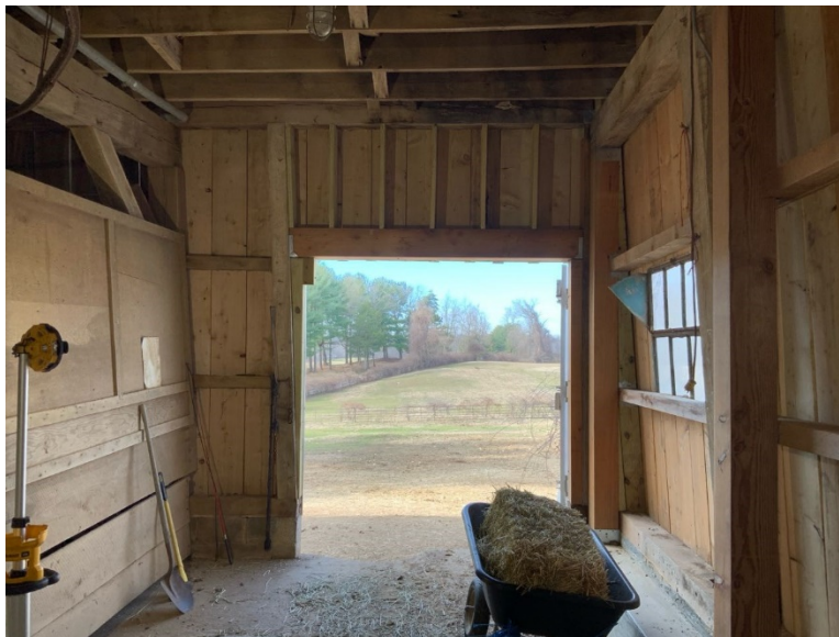
ES Photo 11 – New repairs on Northwest corner (REF Photo S100 - Appendix B2)
