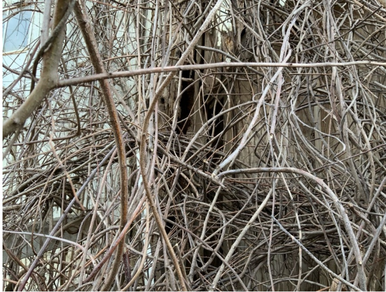
ES Photo 10 – Siding at southwest corner has holes – column appears to be rotting throughout its height – heavy vegetation (REF Photo S114 – Appendix B2).
