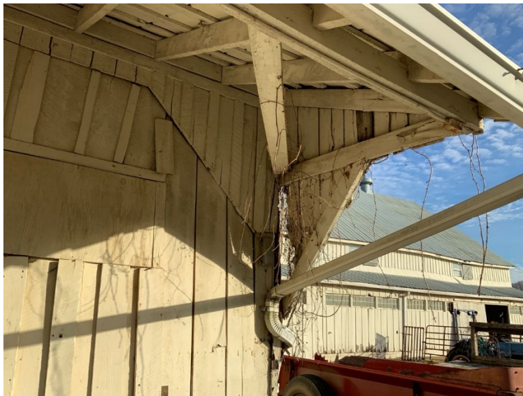
ES Photo 12 – Overhead support diagonal is disconnected at the base and overhang is leaning (REF Photo S140 Appendix B2)
