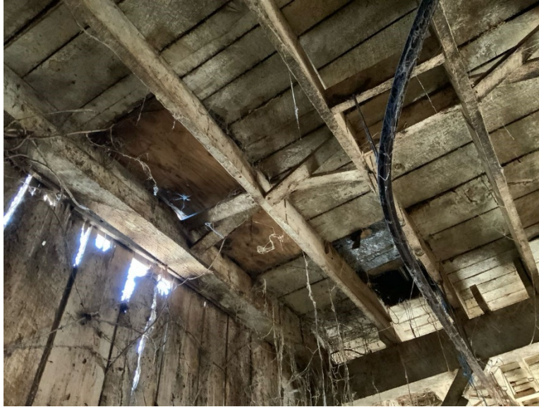
ES Photo 7 – Hayloft from below – typical rotting/broken/missing floorboards – Lean on structure (REF Photo S68 – Appendix B2)
