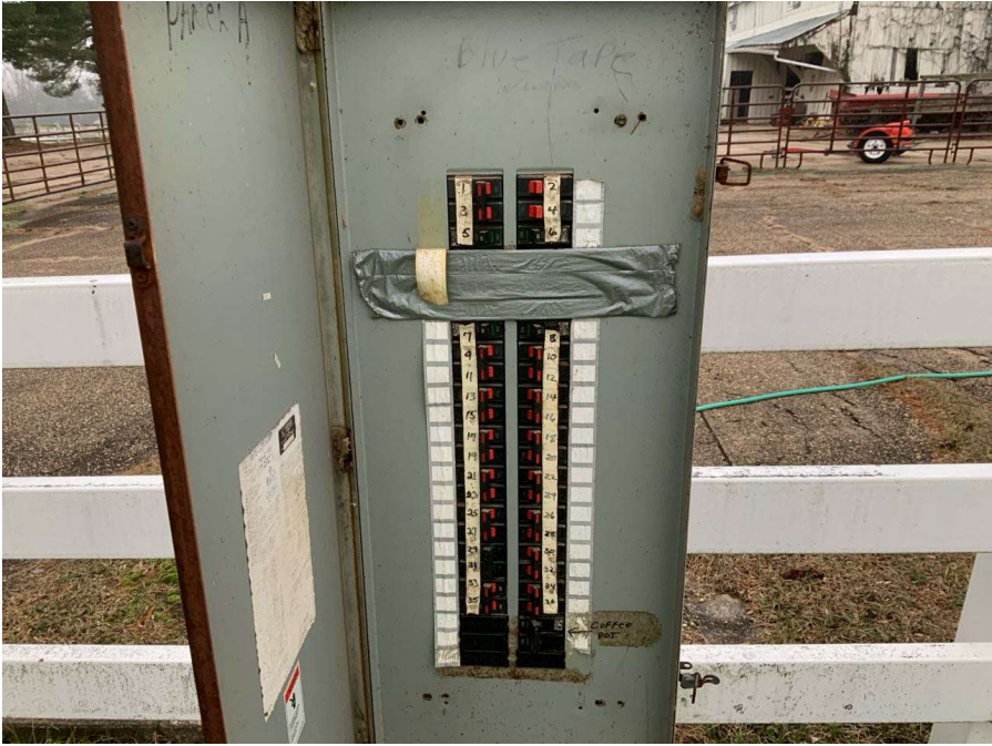
Photo EL-2: Site mounted panelboards are missing circuit breaker knockouts.
