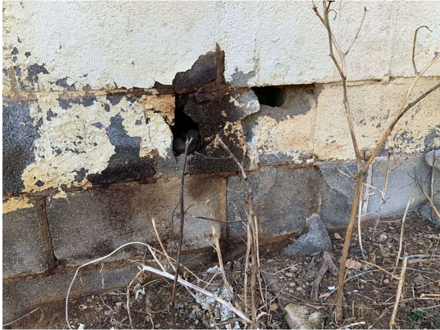
Photo S-155: Typical chips in exterior faces of the cells of the CMU foundation wall blocks at the west elevation.
