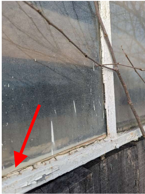
Photo E-1: Tan/white caulk associated with the barn's exterior windows. Identified as potential ACM. Windows are present in all exterior walls.
