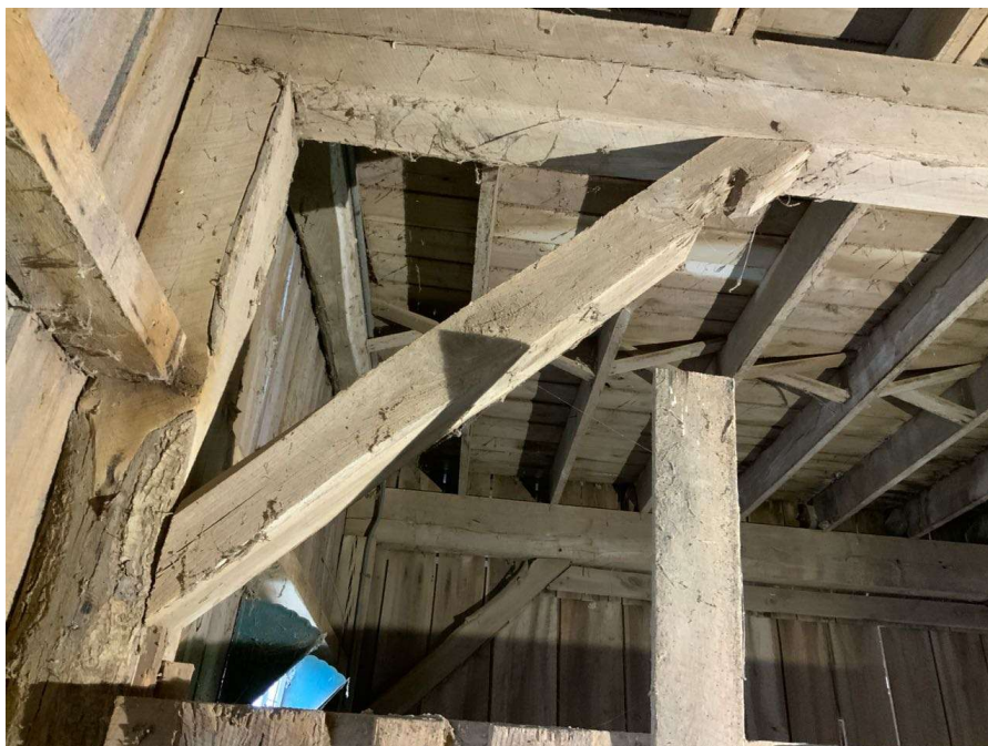
Photo S-130: West brace at Column T/3 at grade level has a notch cut out of the bottom face (looking south).
