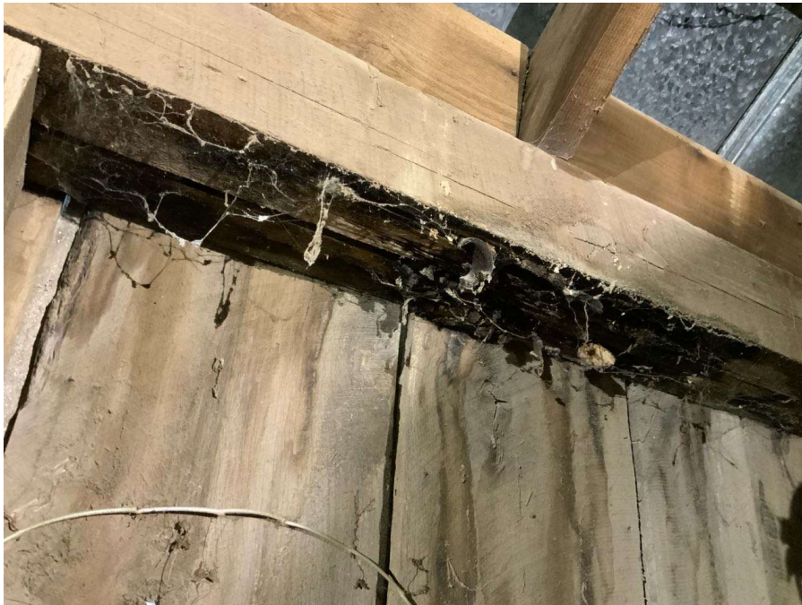
Photo S-20: Roof beam between Columns D/4 and E/4 exhibits rot with full icepick penetration.
