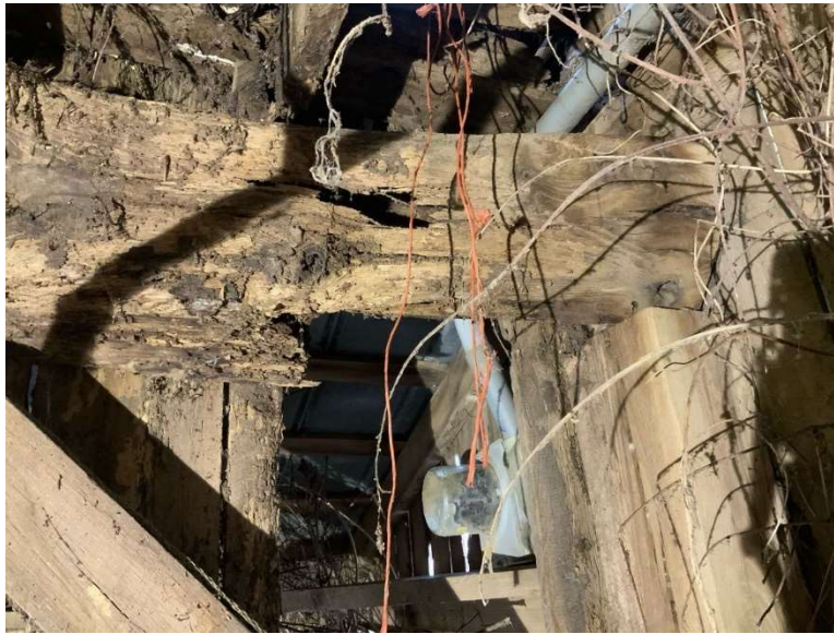
ES Photo 8 – Critical finding at hayloft floor beam – west end of beam has approximately 90% section loss – (REF Photo S81 – Appendix B2)
