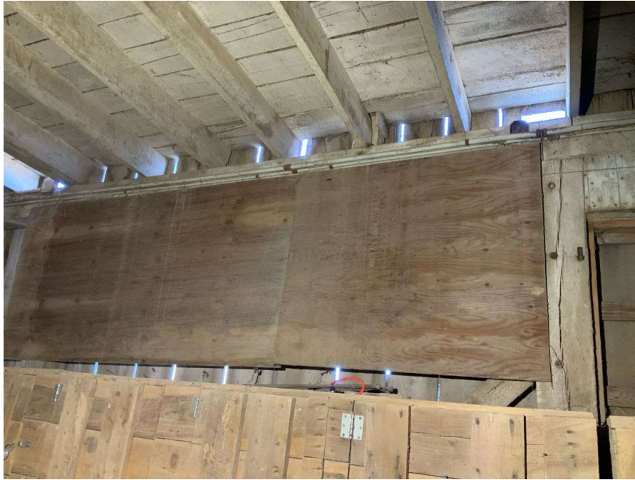
Photo S-87: Rotted floor beam between Column J/1 and K/1 could not be observed from the interior due to plywood obscuring the view (looking north).
