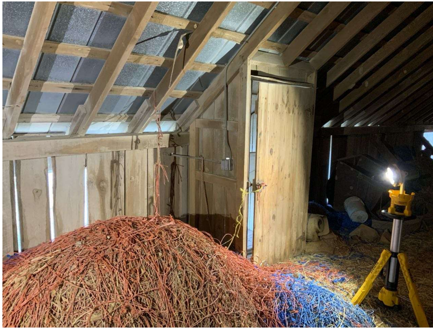
Photo S-63: There is a door entryway at Gridline K/1 instead of a column with brace. It is unknown whether this was designed as part of the original construction or installed as a renovation.
