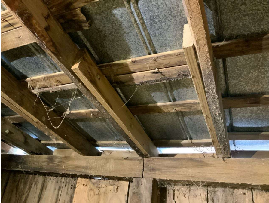
Photo S-11: Previously sistered roof rafters along Gridline 7 between Gridlines H and I.
