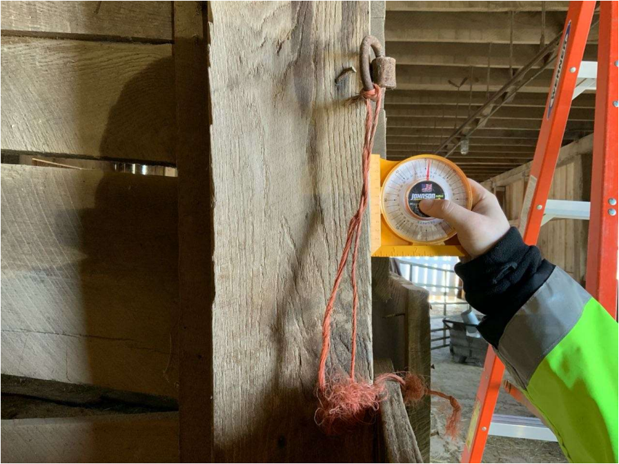
Photo S-101: Column E/2 at grade level is leaning up to 6 degrees towards the south.
