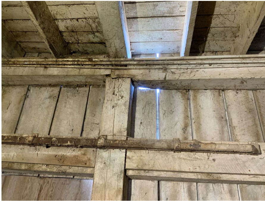
Photo S-83: Severe rot at floor beam between Columns I/1 and J/1. The west end of the beam has approximately 75% section loss. Beam crushing is observed at the bearing location.
