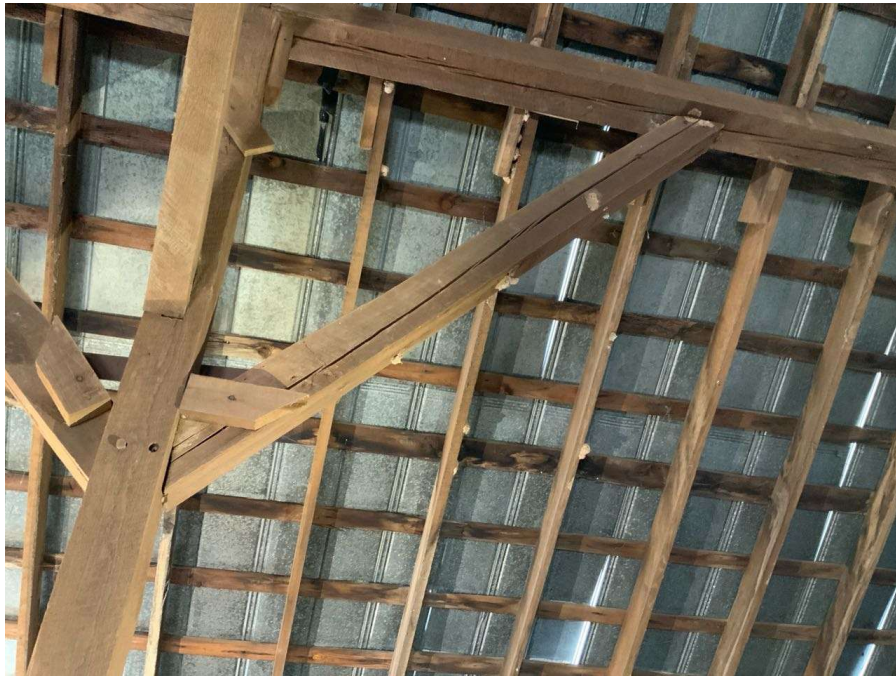
Photo S-43: Typical check in the east/west knee braces in hayloft. West brace at Column C/3 shown looking south.
