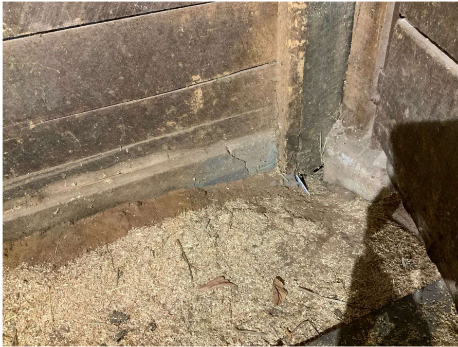
Photo S-103: Bearing loss at Column I/2 at grade level. Note stick rule is poking through from the other side.
