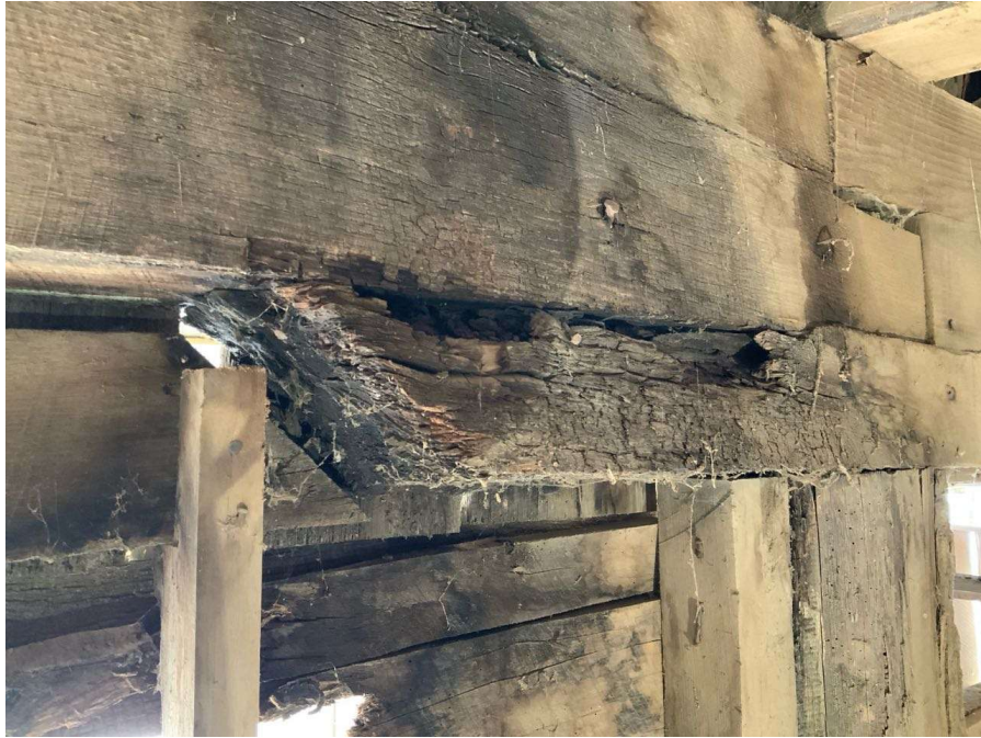
Photo S-85: Water damage and rot at west end of floor beam between Columns F/4 and G/4 (looking south). Supporting column cap at Column F/4 has severe rot.
