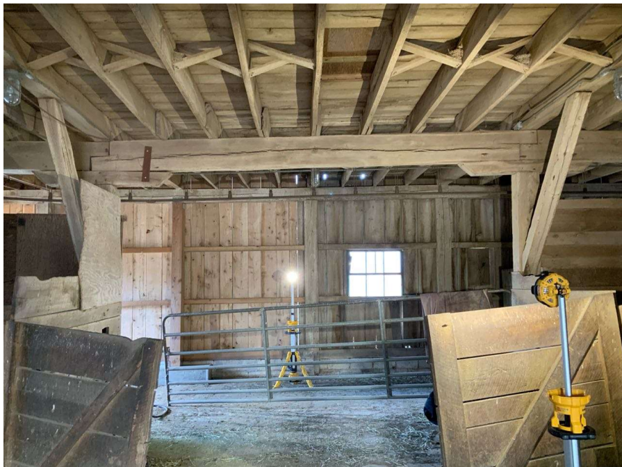
Photo S-72: Typical check in the floor beams spanning east/west. Beam between Columns C/2 and D/2 shown looking north.
