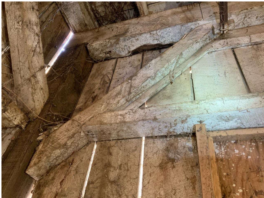
Photo S-128: The west brace at Column N/7 at grade level is not connected to the column at the base connection (looking south). Note the wind girt is connected to the brace and cannot efficiently transfer loads to the column.
