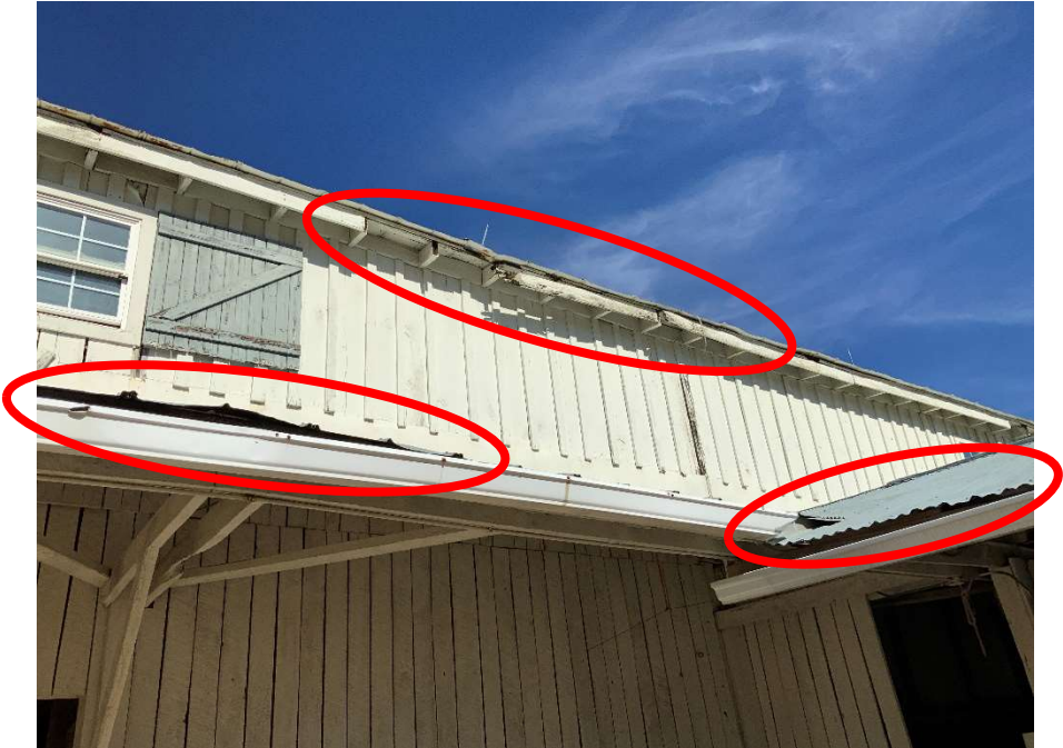
Photo A-3: Sections of lifted metal roof panels and deteriorated/missing fascia boards.
