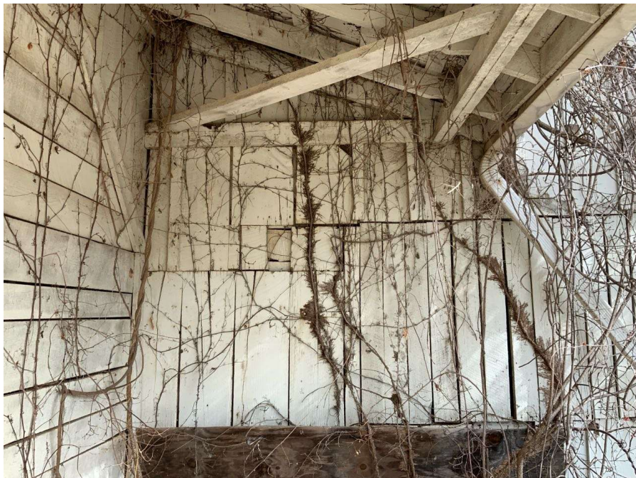
Photo S-136: The overhang at Column H/4 does not have any diagonal support but the wall of the lean-on structure appears to be supporting the overhang instead.
