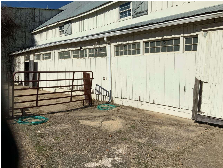
Photo G-19: General view of non-bearing curtain wall bump out under the cantilevered overhang along the south elevation. Bump out at the east wing shown looking north. Note the bump out is sitting on a CMU wall.
