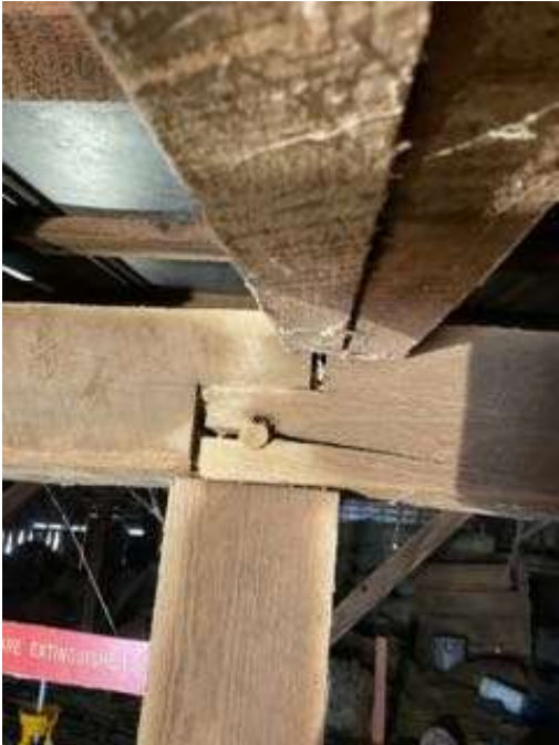
Photo S-26: Split in the east/west face of the roof beam spanning between Columns L/6 and M/6 at the west bearing.
