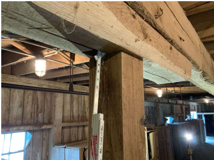
Photo S-116: Replaced column at Column O/2 at grade level has no positive connection to the cap at the top.
