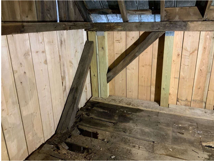
Photo S-61: South brace at Column B/1 in hayloft exhibits rot at base connection to the floor beam. The wind girt and roof beam also exhibit signs of rot at the connection interface. Note broken floorboards in the region preventing hands-on access.
