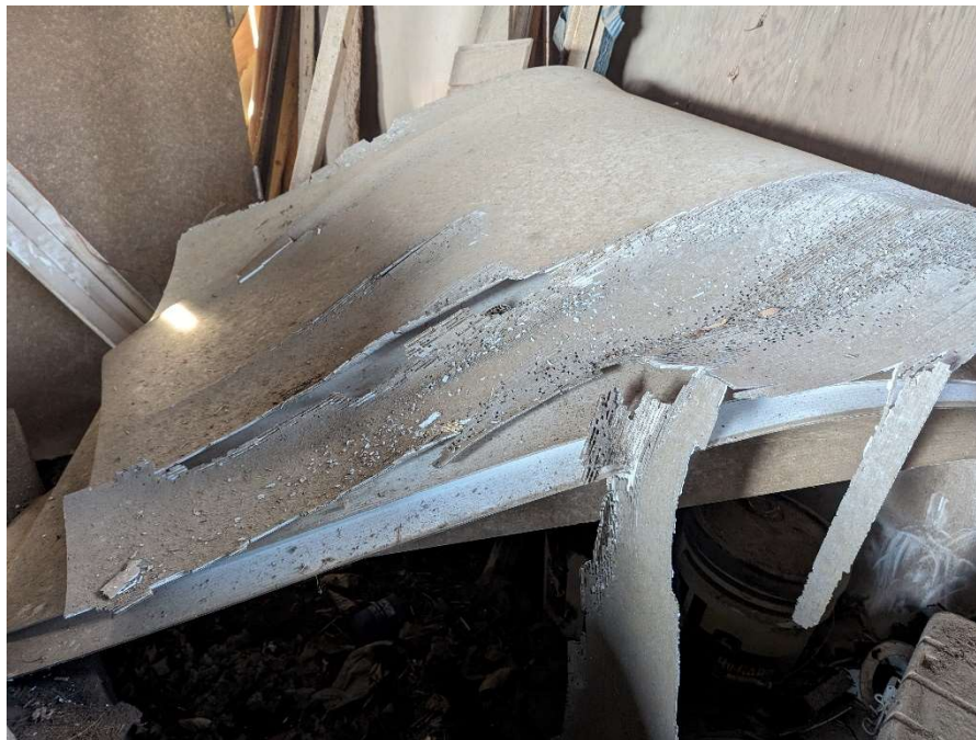
Photo E-2: Corrugated sheets in the garage/outbuilding south of the barn. Identified as potential ACM.
