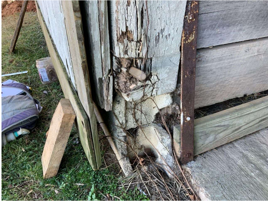
Photo S-149: Rot with full icepick penetration in the sill plate below Column S/1. Note the CMU wall is chipped out at this location indicating that this door is likely not part of the original construction.
