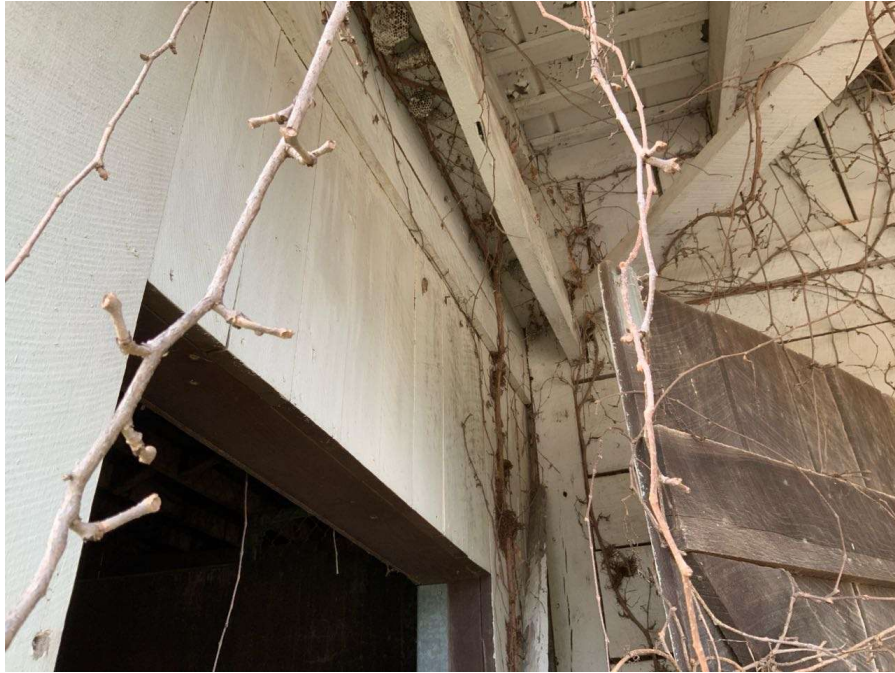
Photo S-135: Missing overhang diagonal supports at Column C/4.
