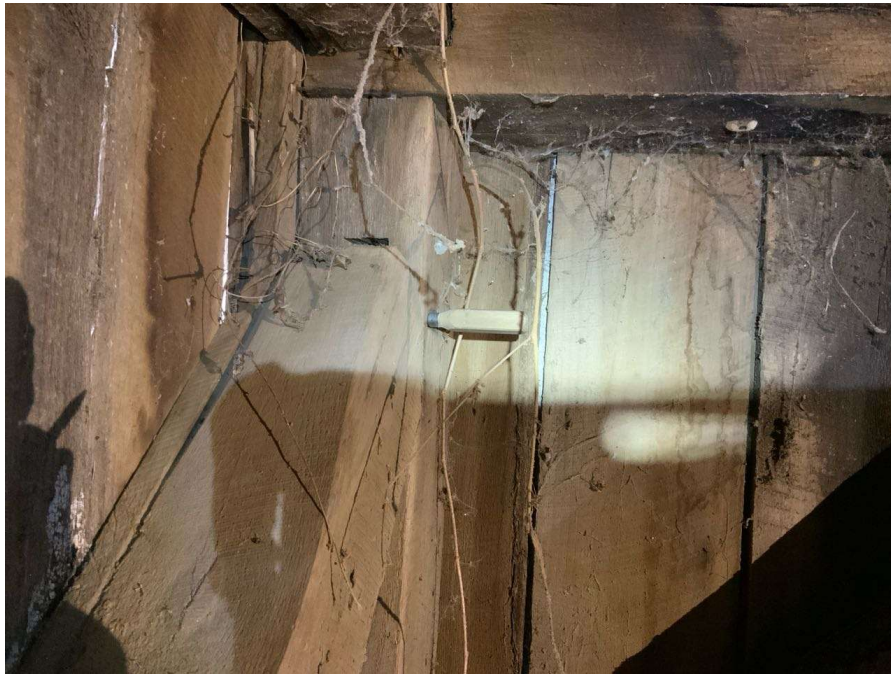
Photo S-59: North brace at Column N/7 in hayloft has no dowel at the top connection.
