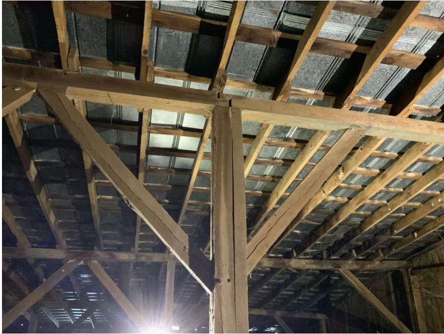
Photo S-27: Gap between roof beams at Column 1/4 bearing location (looking south). Note the extra post added to west side of column to support the beam.
