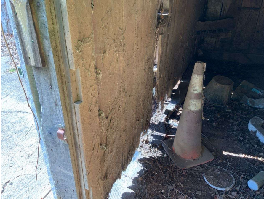
Photo S-163: The curtain wall between Gridline N and O has rotting siding and sill plate near the base. The wall moves when pushed.
