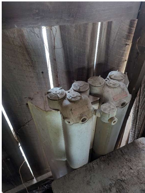
Photo E-14: Fluorescent light fixture in garage/outbuilding south of the barn. Fixture could not be opened to allow inspection of the ballast due to its location. Identified as potentially containing PCBs.
