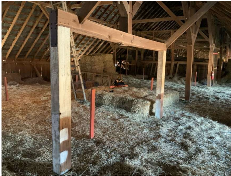
ES Photo 5 – General view of the load spreader beam structures in hayloft (REF Photo G10 – Appendix B1)
