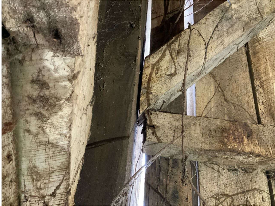
Photo S-133: Typical brace separation at base column connection. Column H/7 shown at grade level. Note the wind girt is disconnected at this location.
