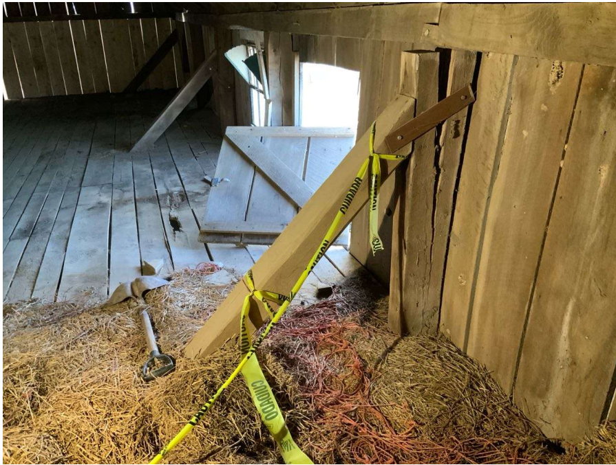
Photo S-15: Perimeter roof beam twisting on split column at hayloft level. Bearing at Column D/1 shown.
