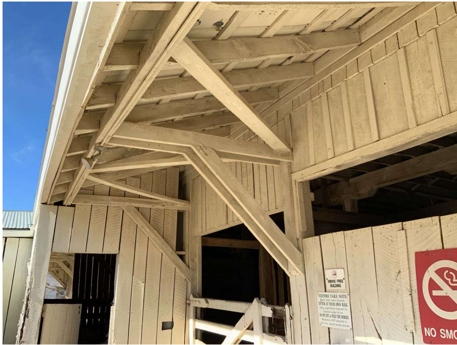
Photo G-17: General view of the cantilevered overhang supported by the perimeter columns along the south elevation. Overhang supports at Column M/7 shown looking northwest.
