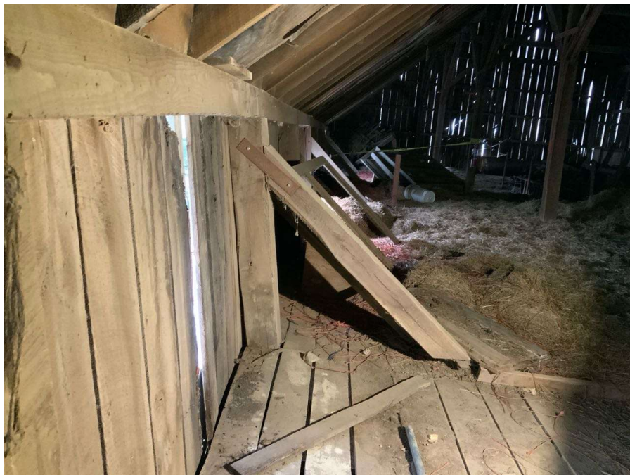
Photo S-38: Hayloft wall is pushed out up to 18 inches along Gridline 4 in the west wing and Column F/4 is leaning up to 7 degrees towards the south (looking west). The lateral brace is disconnected at the base connection to floor beam.
