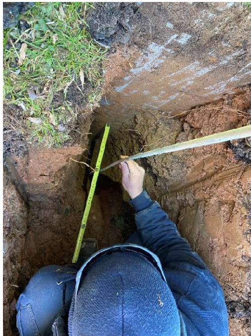
Photo GT-8: Sounding rod used at TP-2 to locate edge of spread footing foundation. Foundation protrudes 1.0 foot from exterior foundation wall.
