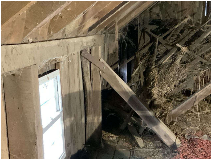
Photo S-37: Split in the east/west faces at Column C/4 in the hayloft (looking west).
