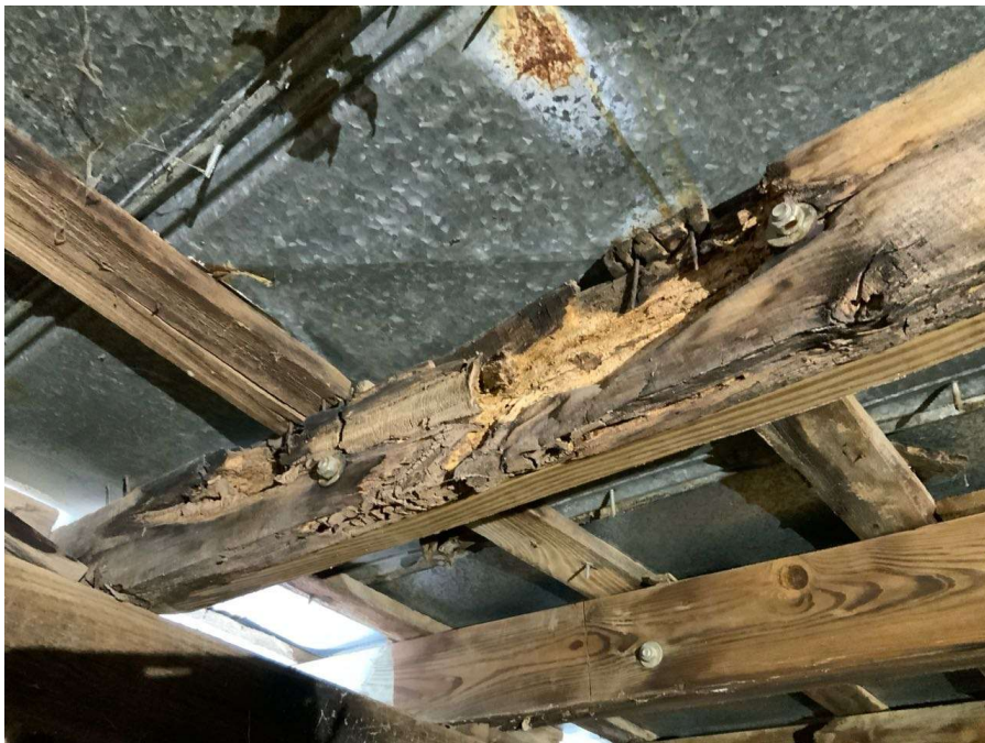
Photo S-12: Previously sistered roof rafter along Gridline 7 between Gridlines I and J. Note the bolts are only through the rotted portion of the rafter.
