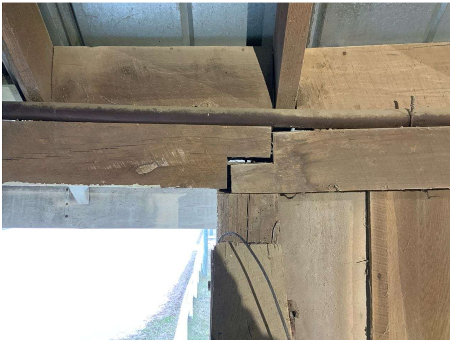
Photo S-18: Column I/1 at hayloft level has 1/2" gap at bearing between west beam and east beam with minimal bearing remaining.
