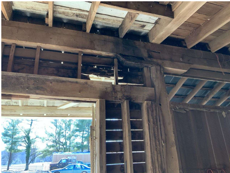
Photo S-170: A new member has been sistered to the original rotting header at the door between Columns F/4 and G/4.
