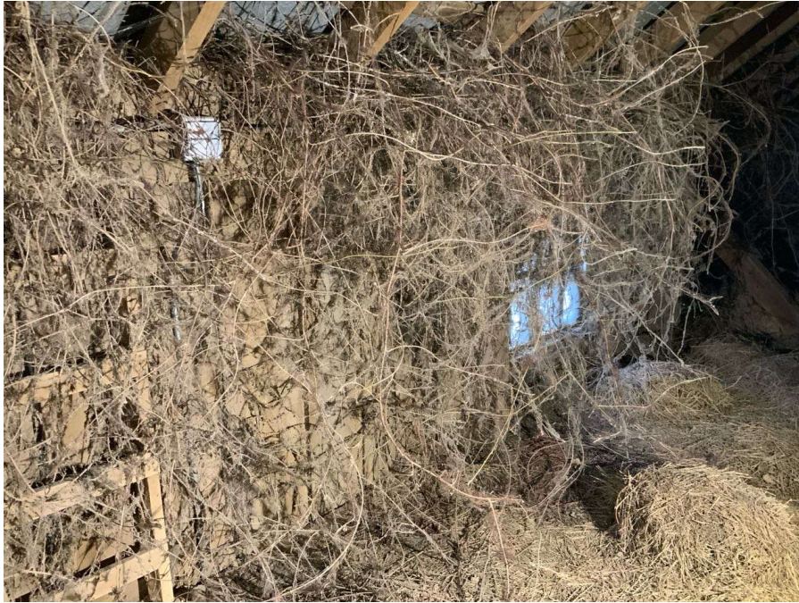
Photo S-7: Heavy vegetation inside the building along the north wall between Gridlines D and H at the hayloft level (looking northeast).
