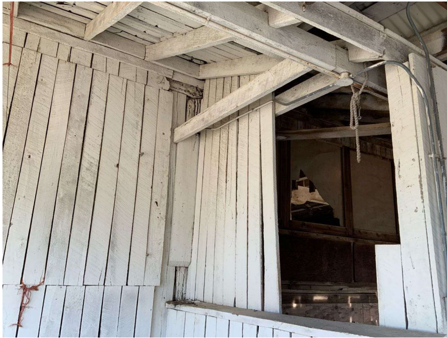
Photo S-139: The west overhang support diagonal is missing at Column K/7.
