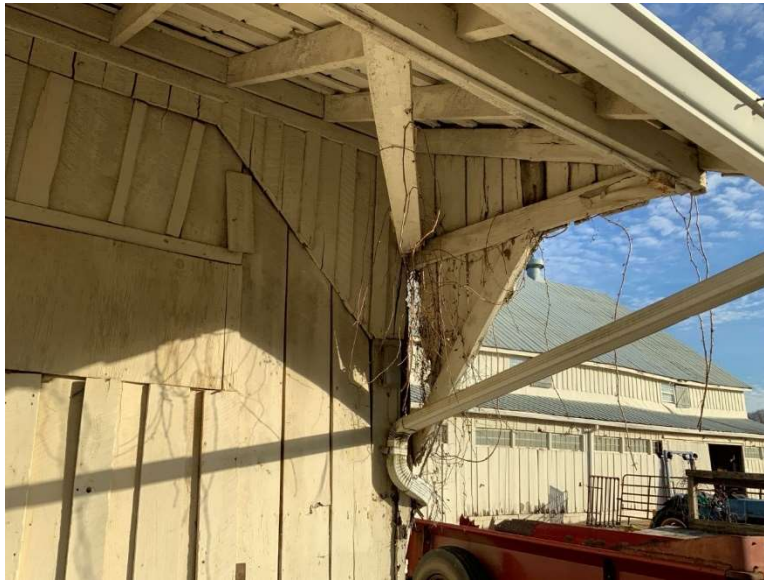
ES Photo 12 – Overhead support diagonal is disconnected at the base and overhang is leaning (REF Photo S140 Appendix B2)
