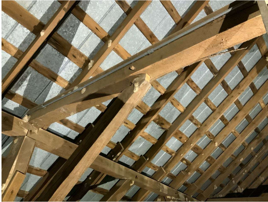
Photo S-57: South brace at Column Q/2 in hayloft is slipping out of the mortise slot at the top connection to the horizontal frame member. The connecting dowel is projecting outwards from the member.
