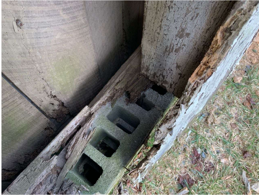
Photo S-111: Bearing loss at Column J/1 at grade level. The column has approximately 30% section loss. The sill plate is completely deteriorated under and to east of column and the column is sitting directly on the CMU foundation wall.
