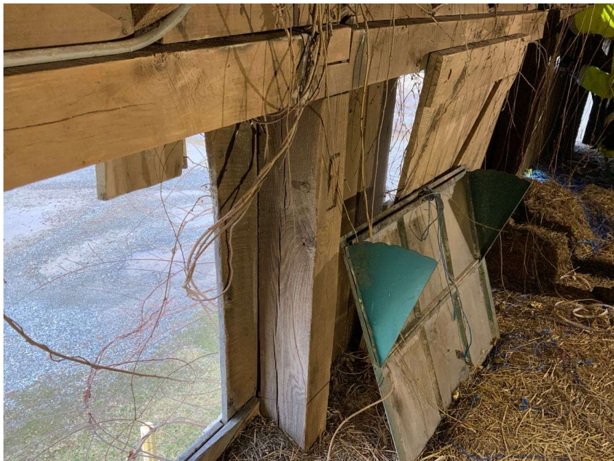
Photo S-62: South brace at Column Q/1 in the hayloft appears to have been cut off and removed, likely at the same time that the load transfer spreader structures were installed.
