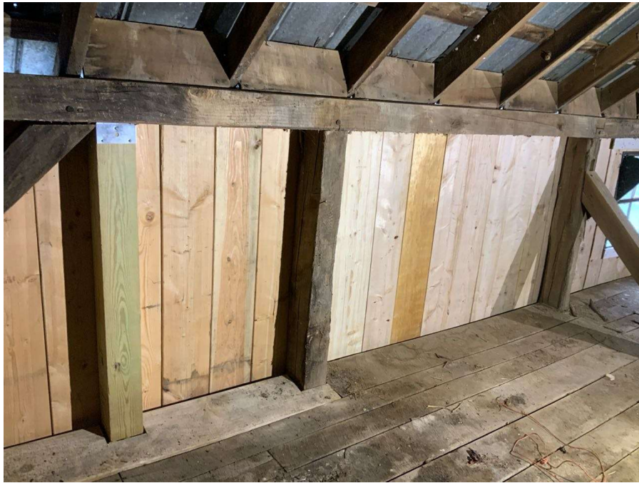
Photo G-9: General view of an intermediate column supporting a roof beam along the perimeter in the hayloft. Intermediate column between Columns B/1 and C/1 shown looking northeast. Note an additional intermediate column was added at this location during a previous repair.
