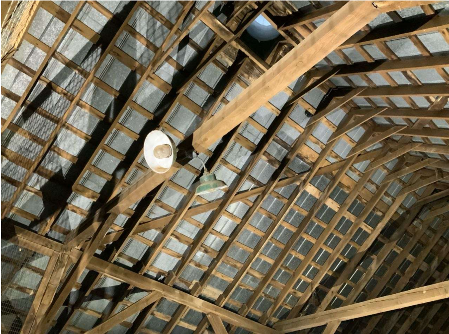
Photo EL-1: Ceiling mounted lights in hayloft do not have protection guard over the light fixture bulb.
