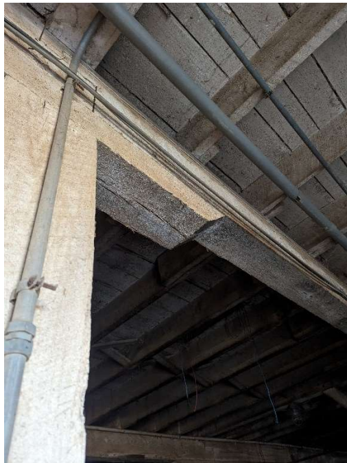
Photo E-8: Flaking white paint on interior walls and timbers. Identified as potential lead-based paint.
