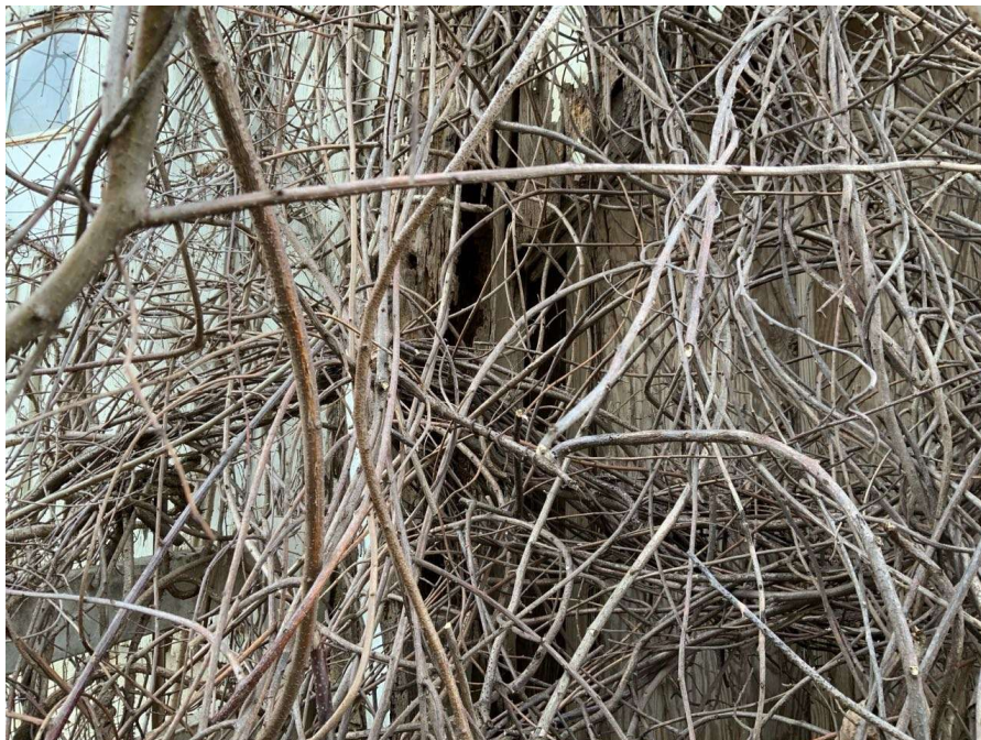
Photo S-114: Siding at Column B/4 has holes and column appears to be rotting throughout its height. Access to column was limited due to heavy vegetation and the critical finding in the floor beam at this location.
