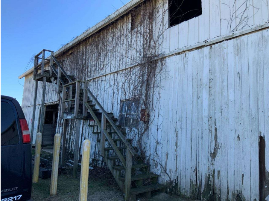
Photo G-6: General view of the exterior stairs at the east end of the north elevation.
