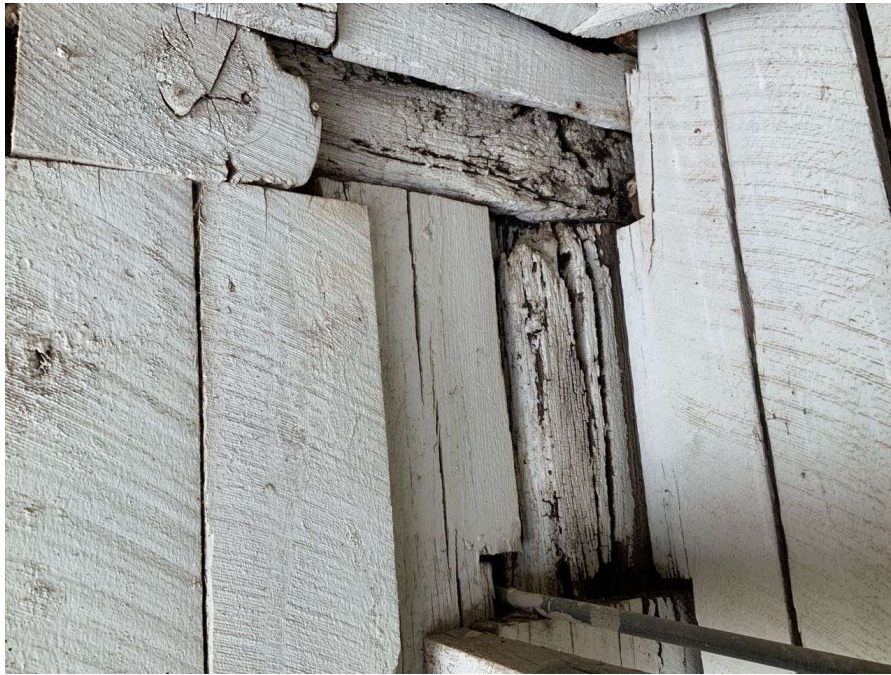
Photo S-97: South face of the at-grade column cap at Column K/7 is exposed to exterior and has soft rot with up to 1.5" icepick penetration.
