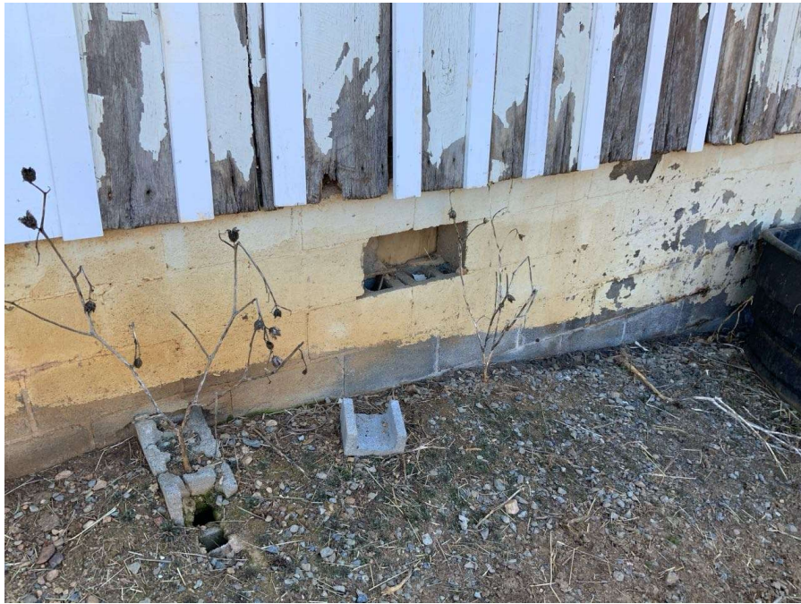
Photo S-153: Missing block in CMU foundation wall at the west elevation (looking southeast).
