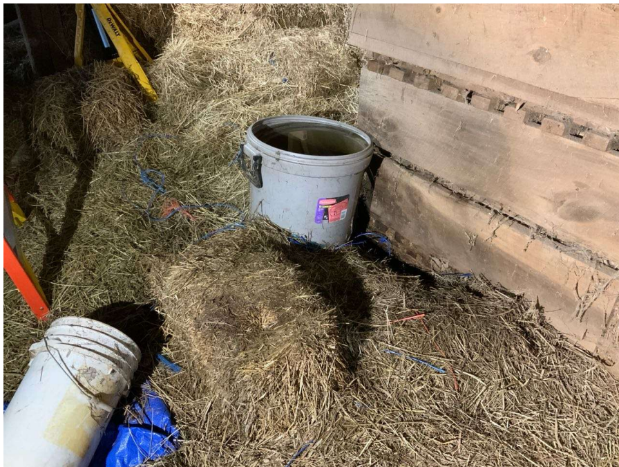
Photo S-4: 32-gallon bucket near Column M/4 full of water under previous roof patch.
