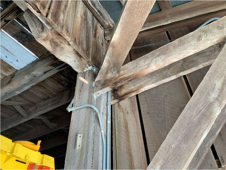
Photo S-143: Rot at the overhang support horizontal member connection to Column S/4.
