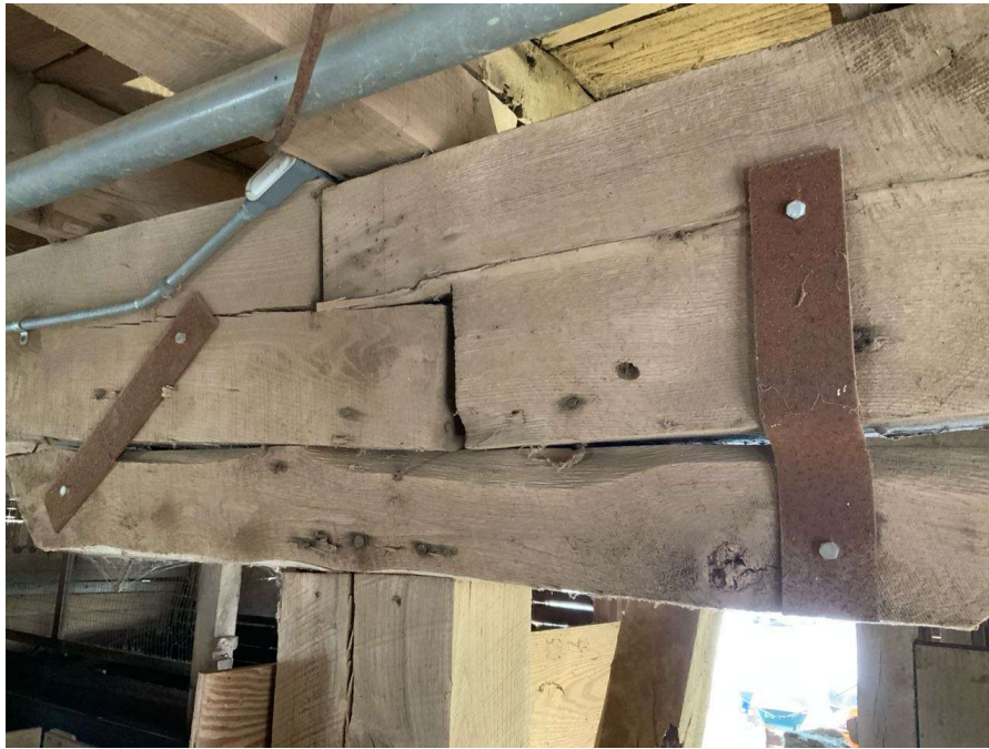
Photo S-75: Retrofit straps at the grade level Column C/2 cap. Note gaps in bearing surface of beam to column cap.
