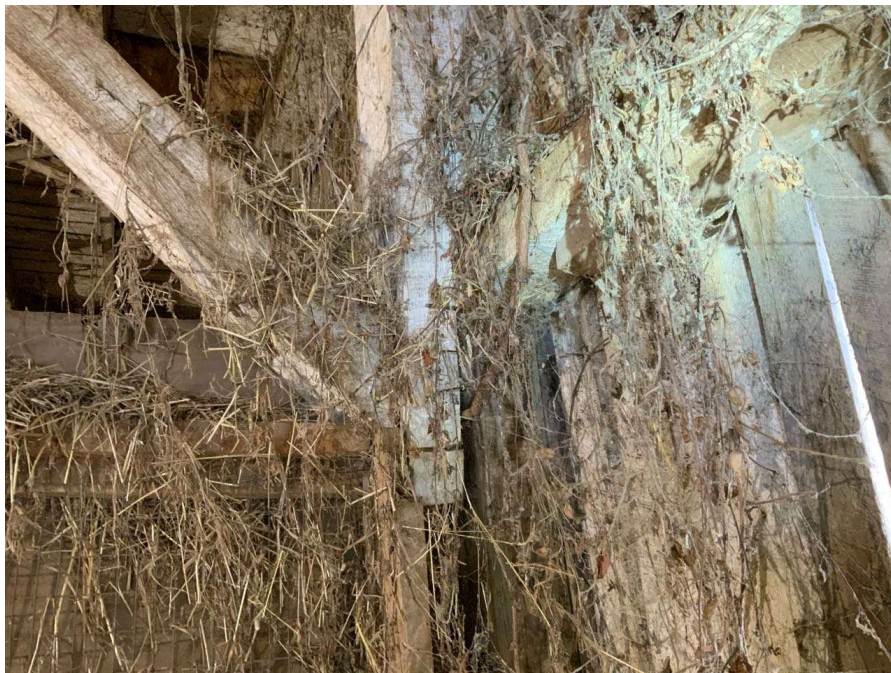
Photo S-120: The bottom portion of Column N/6 at grade level consists of a 5.75" x 5.75" post supporting the original column above.
