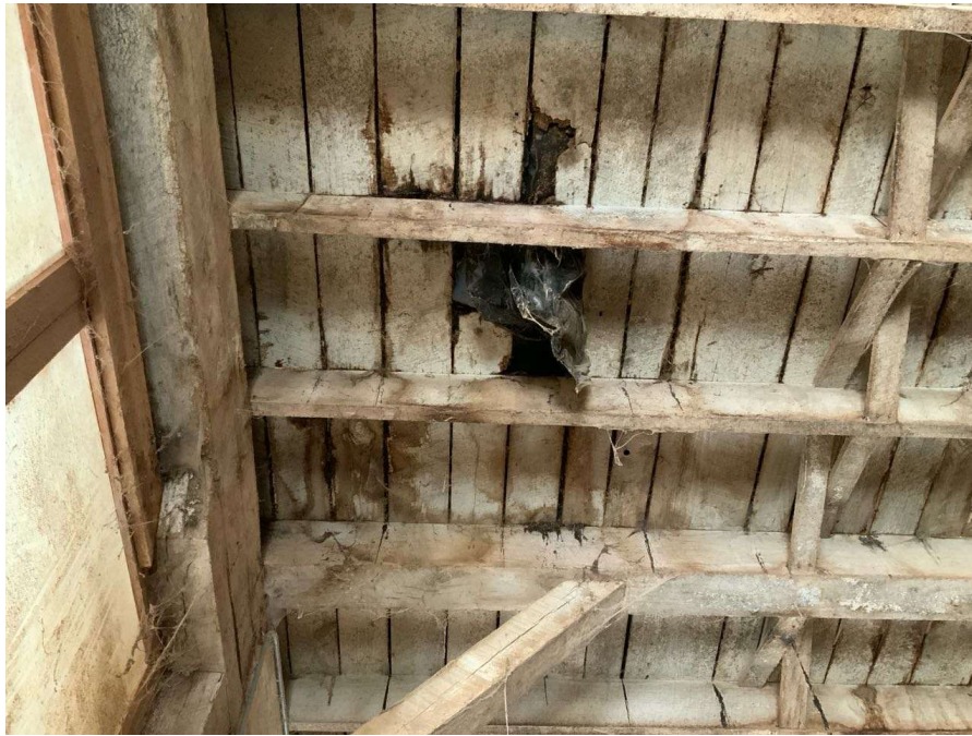
Photo S-67: Typical rotting/broken/missing floorboards. Lean-on portion of structure near Gridline 7 shown looking west.
