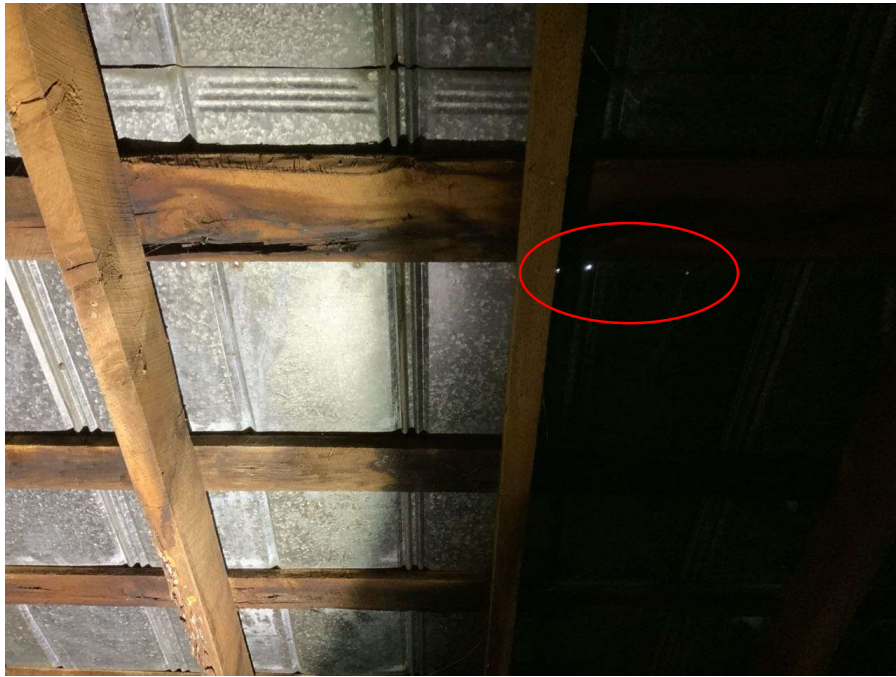
Photo S-1: Typical pinhole leak in roof metal deck. Deck near Column L/6 shown.
