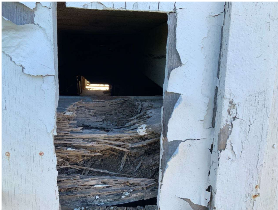
Photo S-82: Severe rot at floor beam between Columns I/1 and J/1. The west end of the beam has approximately 75% section loss.
