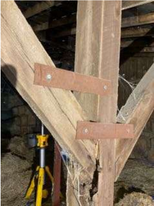
Photo S-48: Disconnected west brace at Column M/5 in hayloft (looking northeast).
