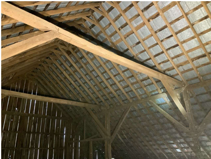
Photo G-8: General view of a knee braced frame at the hayloft level spanning between Gridlines 2 and 3. Frame between Columns D/2 and D/3 shown looking northwest.
