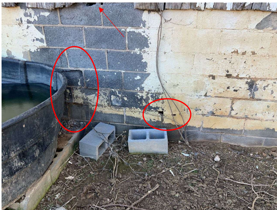
Photo S-154: Typical chips in exterior faces of the cells of the CMU foundation wall blocks at the west elevation.
