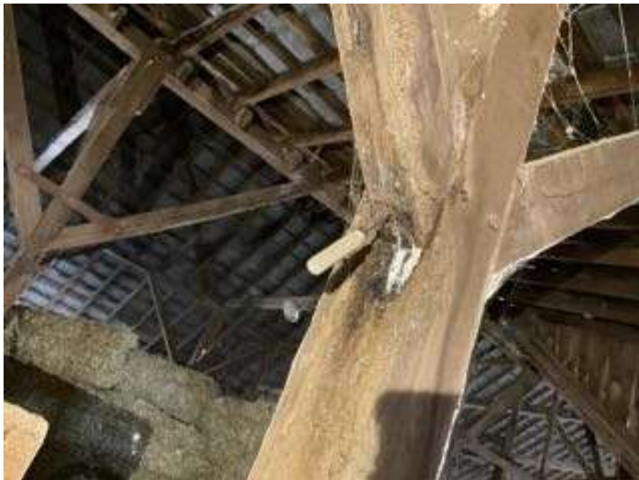
Photo S-52: The west brace at Column M/4 in hayloft exhibits rot at the base connection to the column (looking north).
