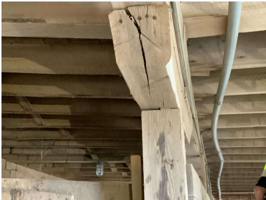
Photo S-96: At-grade column cap at Column E/2 is split and not sitting correctly on top of column. There is a small gap between the top of column and base of cap with approximately 50% bearing remaining.
