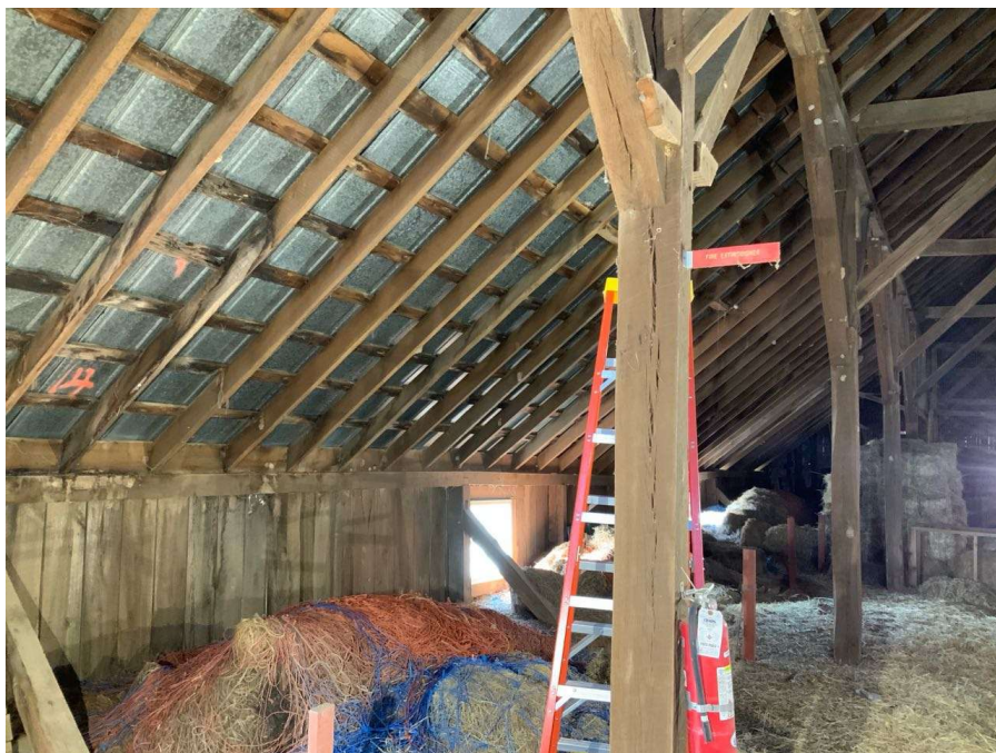
Photo S-34: Split in east/west face of Column R/3 in hayloft (looking west)
