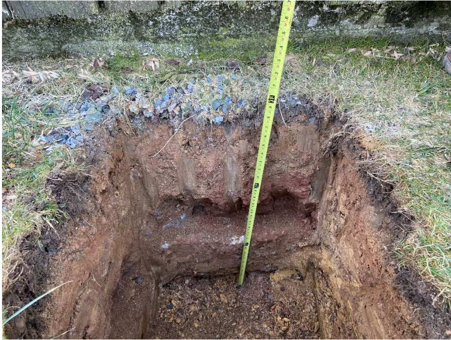
Photo GT-5: Exposed foundation at TP-1 with top of footing measuring 1.9 feet BGS and bottom of footing at 2.8 feet BGS.
