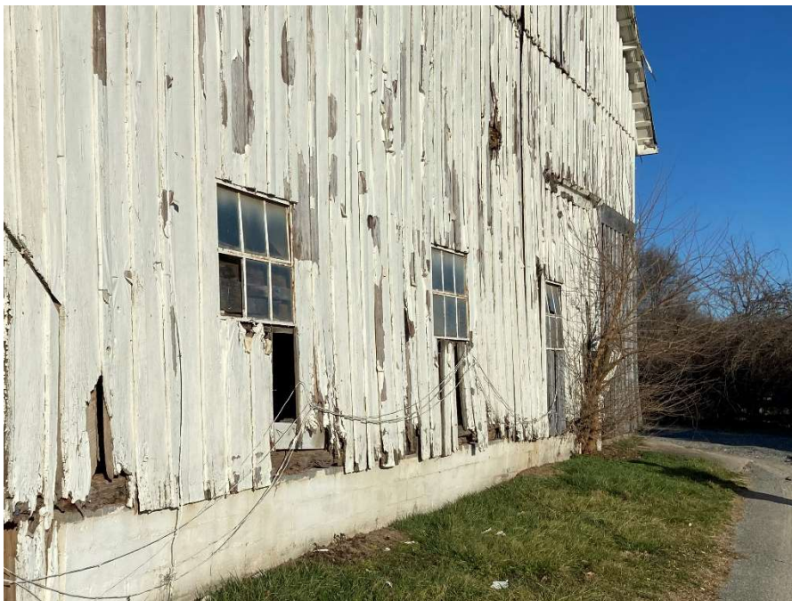
Photo A-18: General exterior photo of window damage and localized deterioration.
