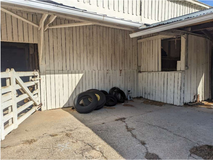
Photo E-21: Tires stacked adjacent to barn’s south exterior wall.
