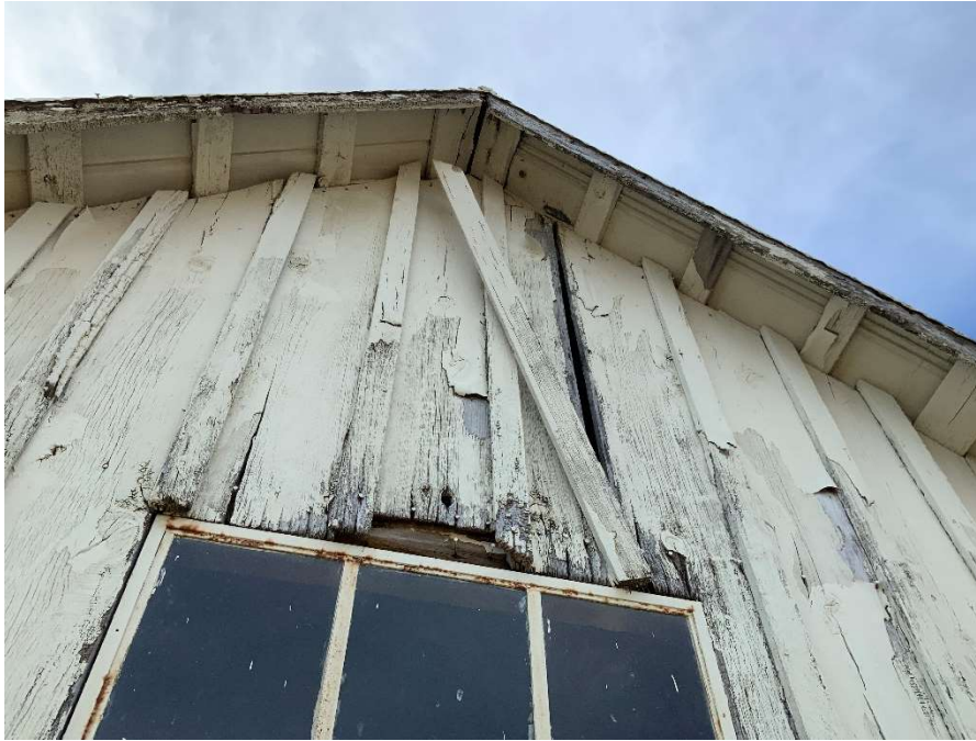
Photo A-21: Window damage and deterioration at head.
