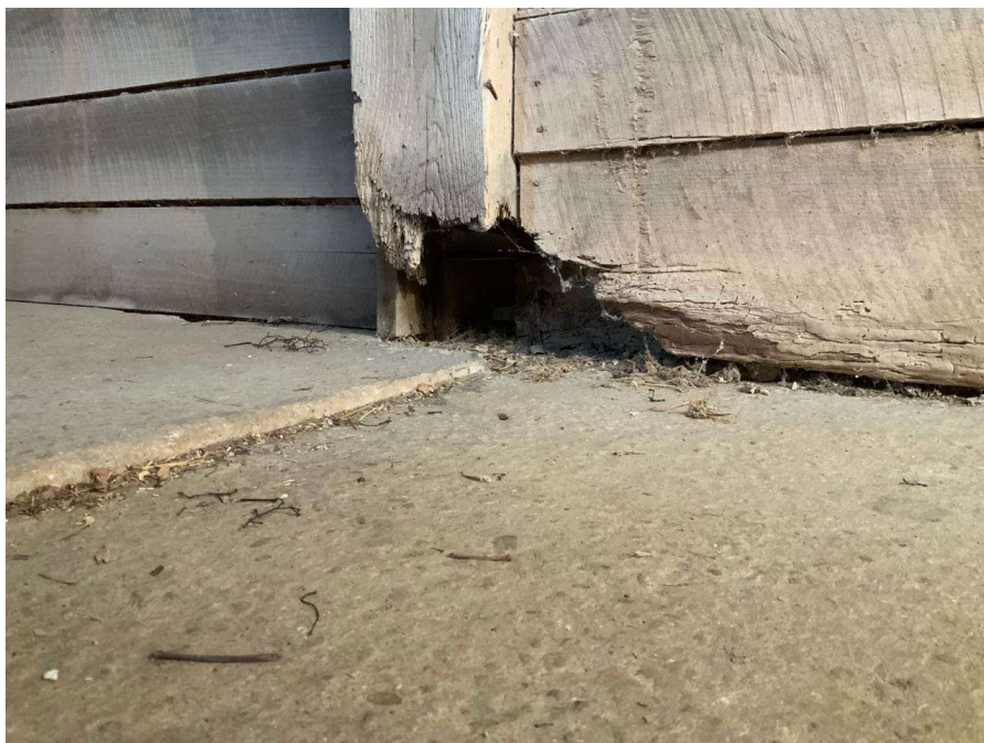
Photo S-110: Bearing loss at Column P/4 at grade level.
