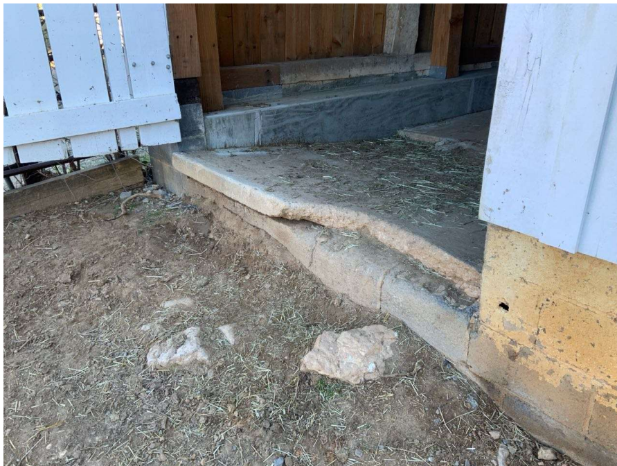
Photo S-158: Settled walkway slab at northwest corner of building.
