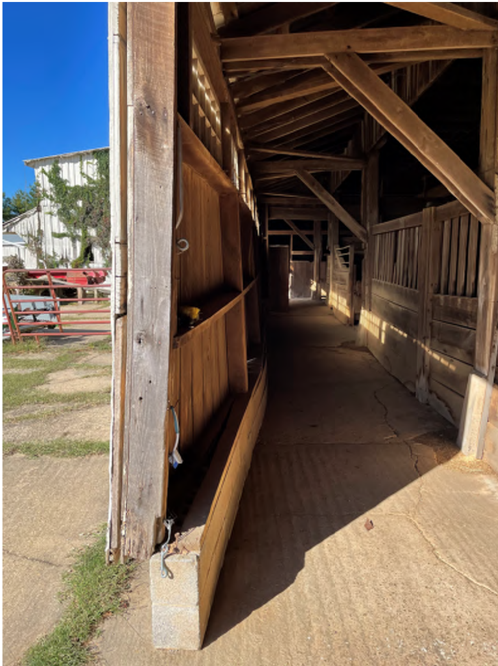
South west foundation wall out of place.
