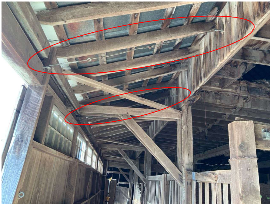
Photo S-166: The eyehooks in curtain wall between Gridline N and T where the golf course allegedly attached tents during large events are attached back to main framing at the top of wall using steel rods.
