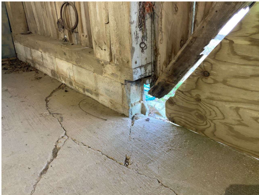
Photo S-122: Chipped out masonry foundation wall indicating door was likely installed or widened after the original construction. Door between Columns E/1 and F/1 shown.
