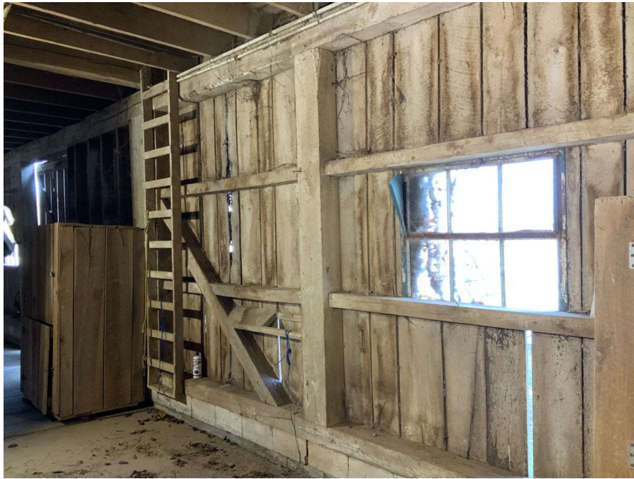
Photo G-13: General view of an intermediate column supporting the perimeter floor beam along the north wall. Intermediate Column Between Columns F/1 and G/1 shown. Note the wind girts span between the columns and also act as the header and sill for the window.
