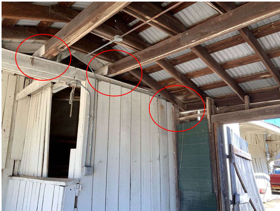
Photo S-160: The wall bump out between Gridlines K and L supports the gravity load from the roof of the out-of-scope outbuilding structures to the south of the main barn.
