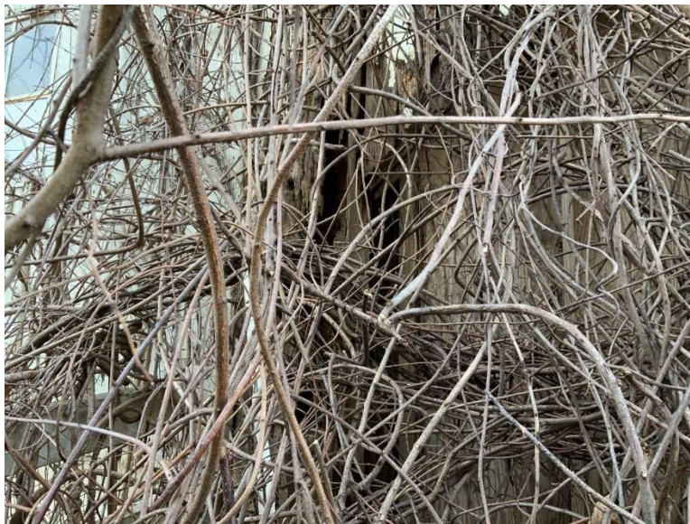
ES Photo 10 – Siding at southwest corner has holes – column appears to be rotting throughout its height – heavy vegetation (REF Photo S114 – Appendix B2).
