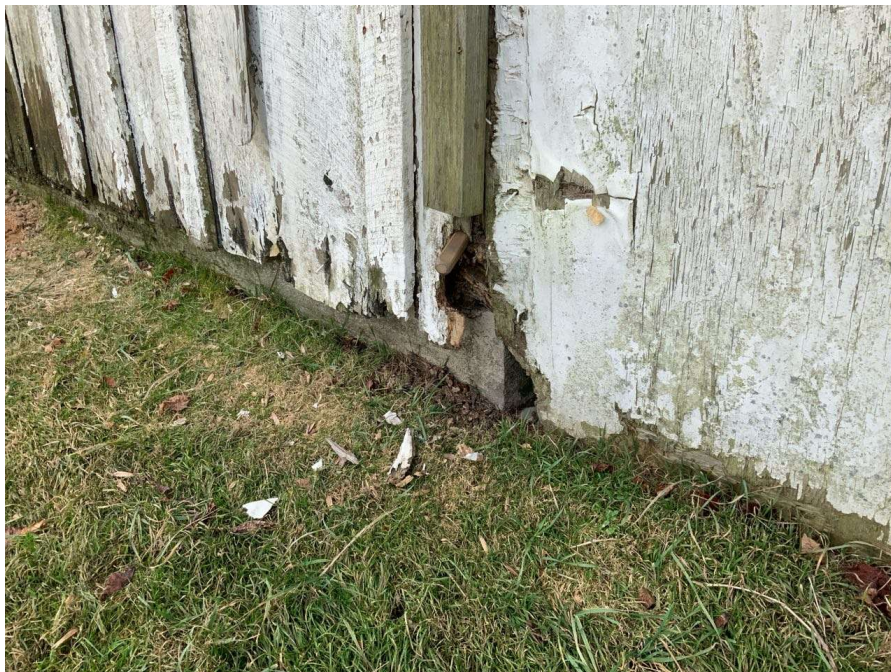
Photo S-146: Rot with full icepick penetration in the sill plate below Column I/1 at grade level.
