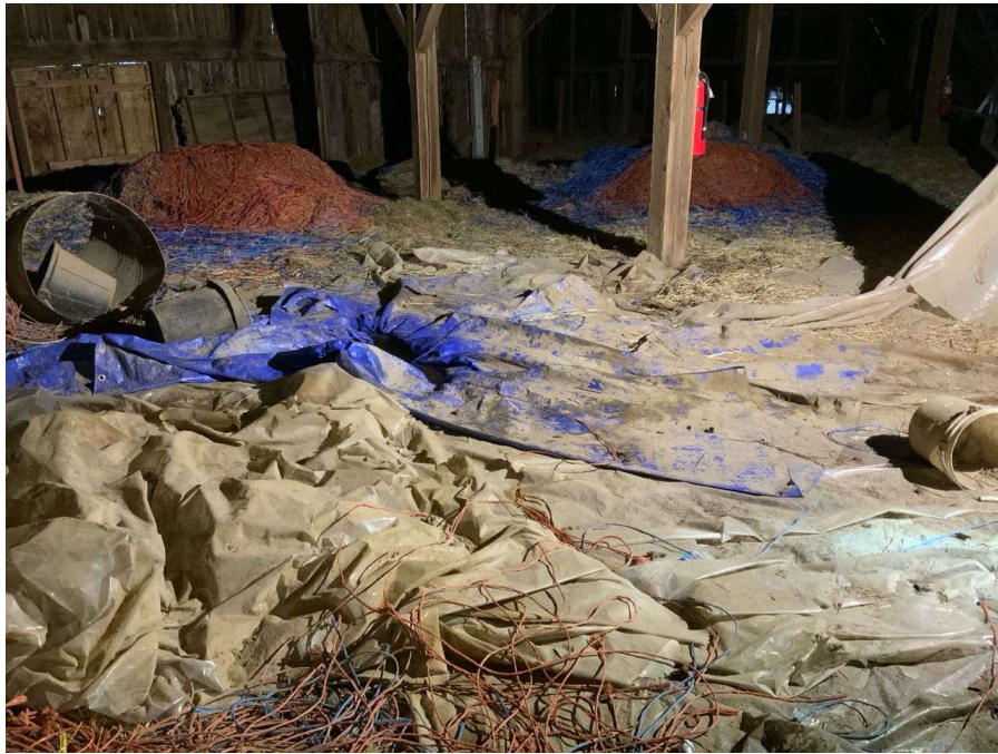
Photo S-3: Tarps with standing water on the hayloft flooring underneath the lean-on region of the structure. Floor shown looking northwest along Gridline 6.
