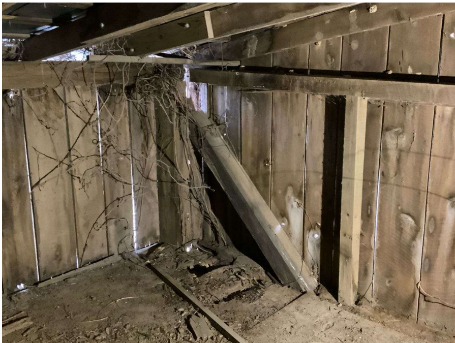
Photo S-42: Severe rot at top of original Column H/7 in hayloft (looking southwest). A new post has been installed to the east of the existing column. The north brace and wind girt are not connected to the new post and the east brace is missing. The floorboards adjacent to the column are rotting.
