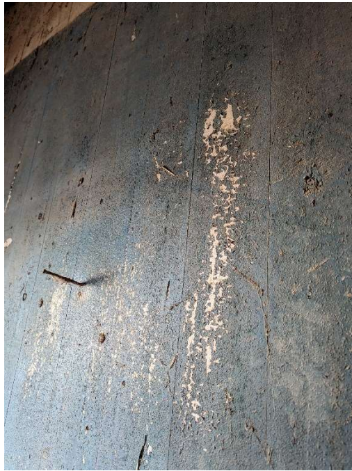
Photo E-7: "Alligator texture" cracking on green interior paint located throughout barn. Identified as potential lead-based paint.
