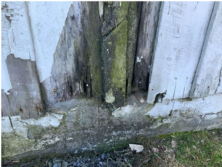
Photo S-148: Rot with full icepick penetration in the sill plate adjacent to Column P/1 at grade level.
