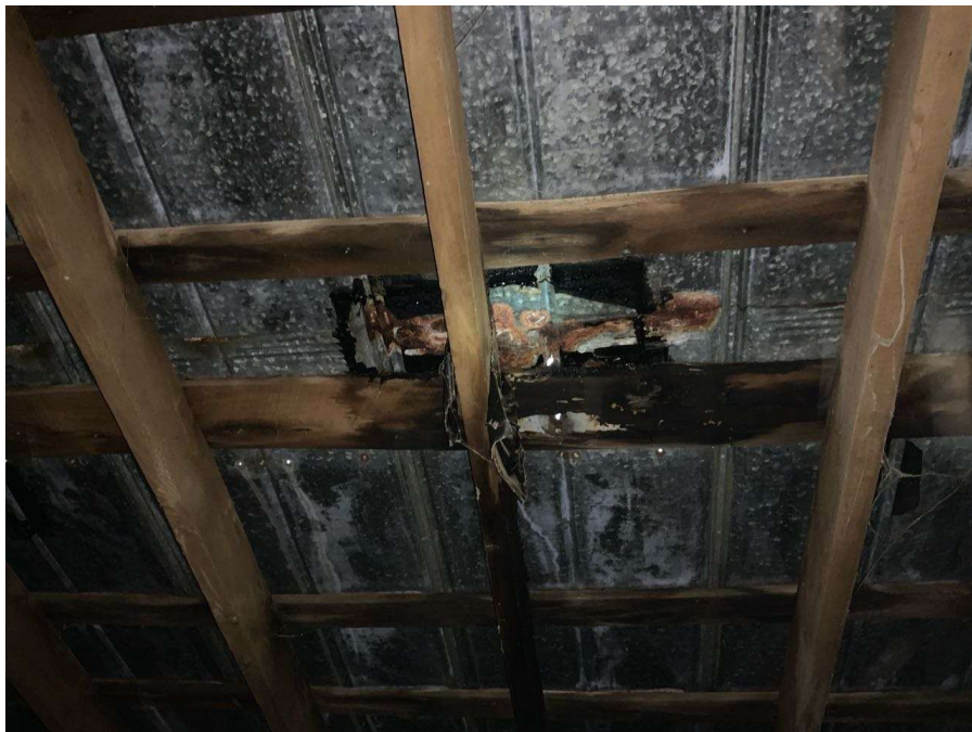
Photo S-2: Typical area of rusted roof deck and failing patch. Deck near Column L/6 shown.
