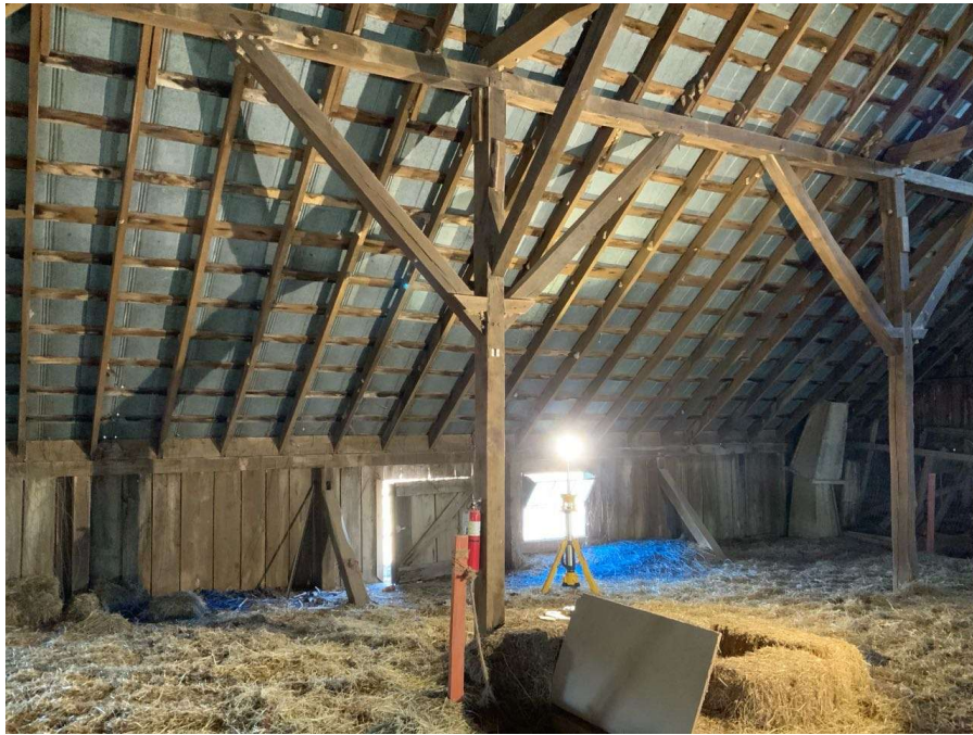
Photo G-7: General view of a typical hayloft braced column. Column R/2 shown looking northeast.
