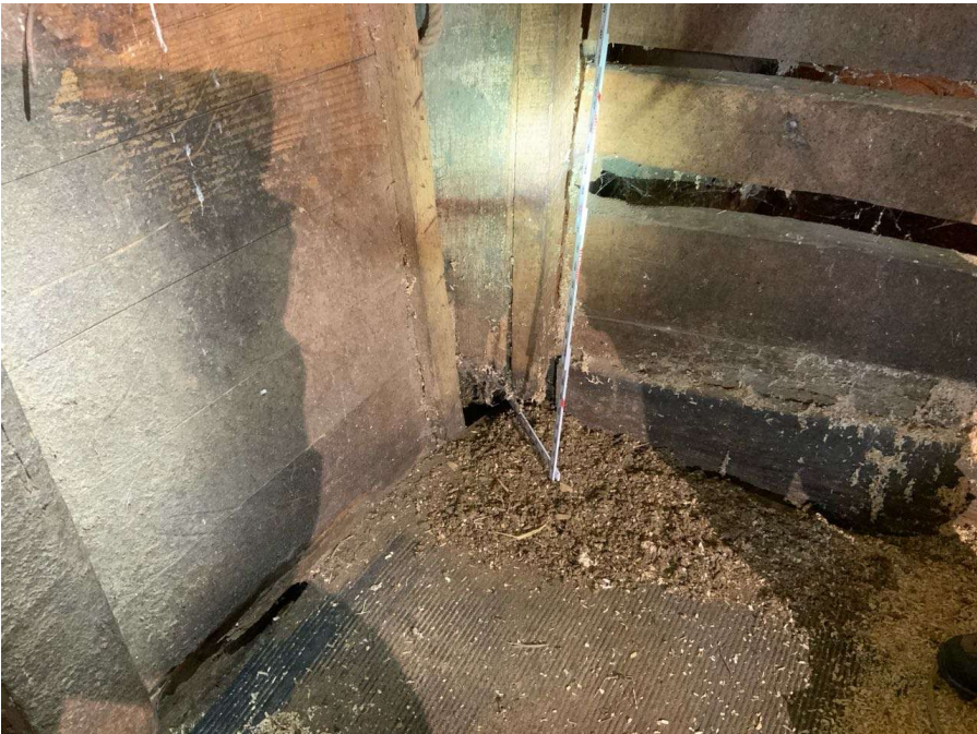
Photo S-106: Bearing loss at Column L/2.5 at grade level.
