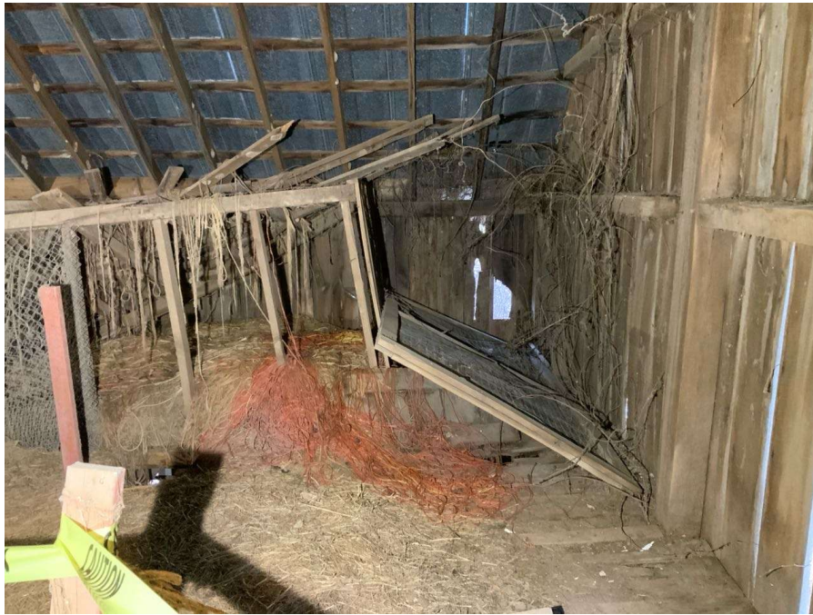
Photo S-51: The east brace at Column B/4 in hayloft appears to be missing based on similar geometry in other portions of the building (looking south).
