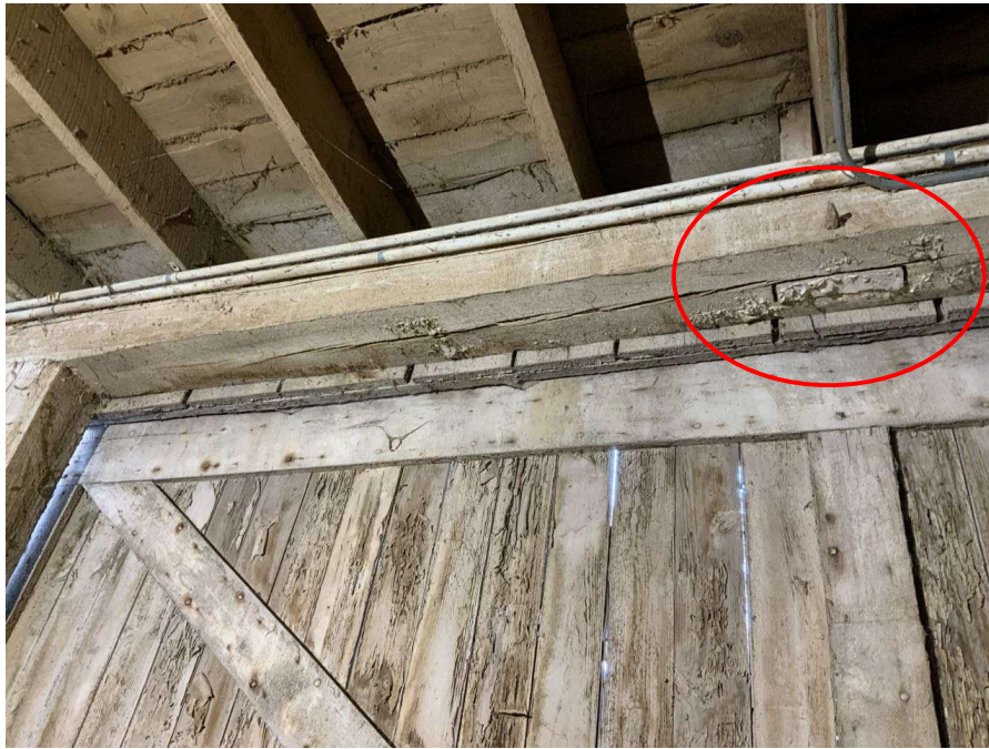
Photo S-123: Cut portion of intermediate column still in mortise slot with dowel. Door between Columns G/1 and H/1 shown.
