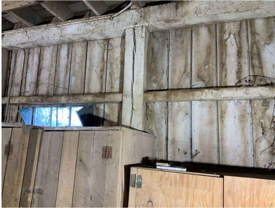
Photo S-121: Typical check on south face of intermediate column at grade level along Gridline 1. Column Q.5/1 shown looking north.
