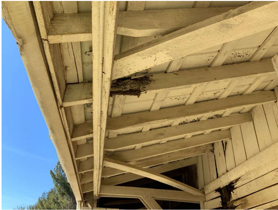
Photo S-13: Rotting overhang roof rafter between Gridlines F and G at south bearing (looking west).
