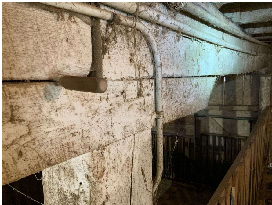
Photo S-78: Both floor beams at Column M/2.5 have limited contact with column cap and are only bearing directly over the column (looking southwest)
