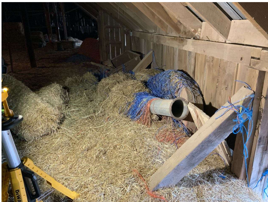
Photo S-84: Haybales and debris directly above severely rotted beam between Columns I/1 and J/1 in hayloft (looking northwest).
