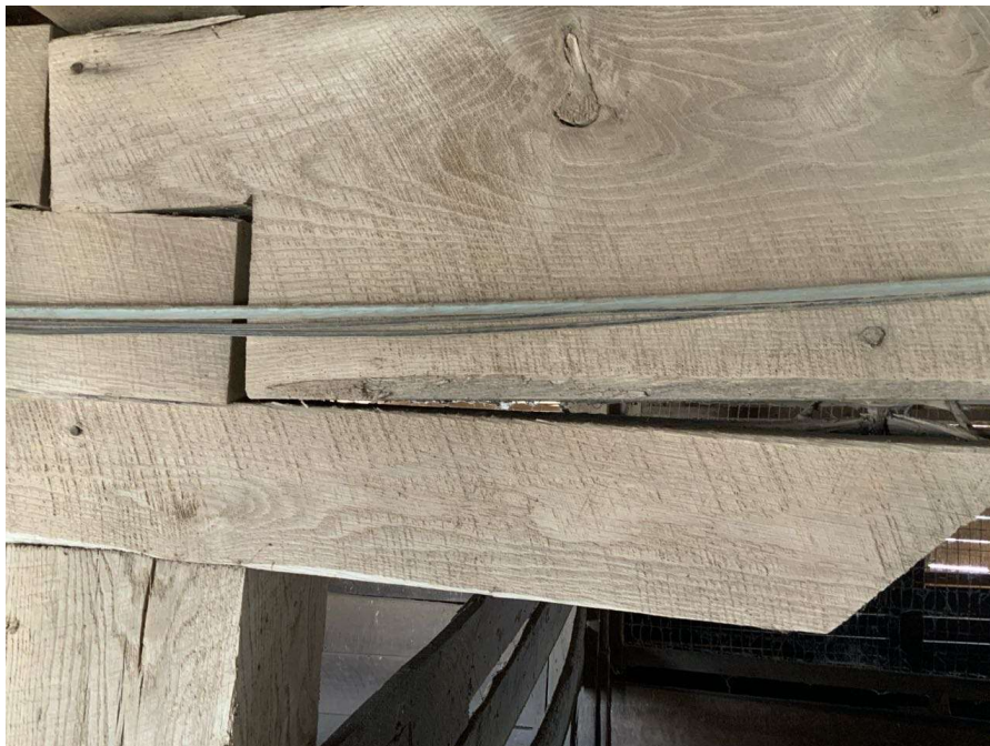
Photo S-76: Uneven floor beam at Column E/2 (looking south). The west beam is not bearing on the cap and only has approximately 2" bearing on the east beam at notch.
