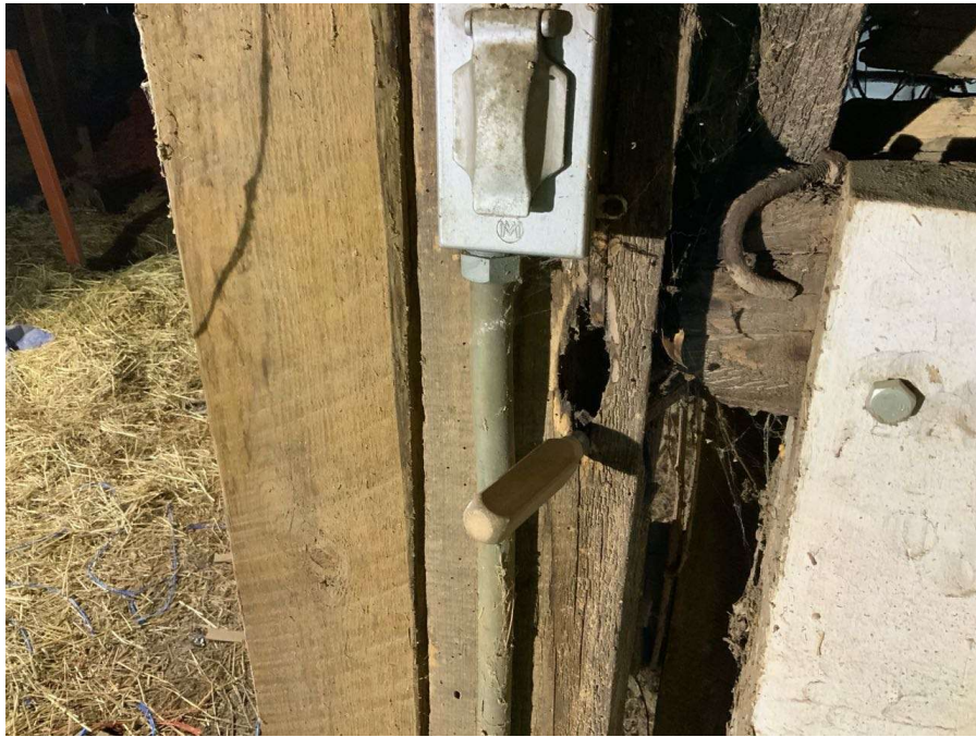
Photo S-39: Severe rot at original Column H/4 in hayloft (looking south). Note a newer column has been installed to the east of the existing column.
