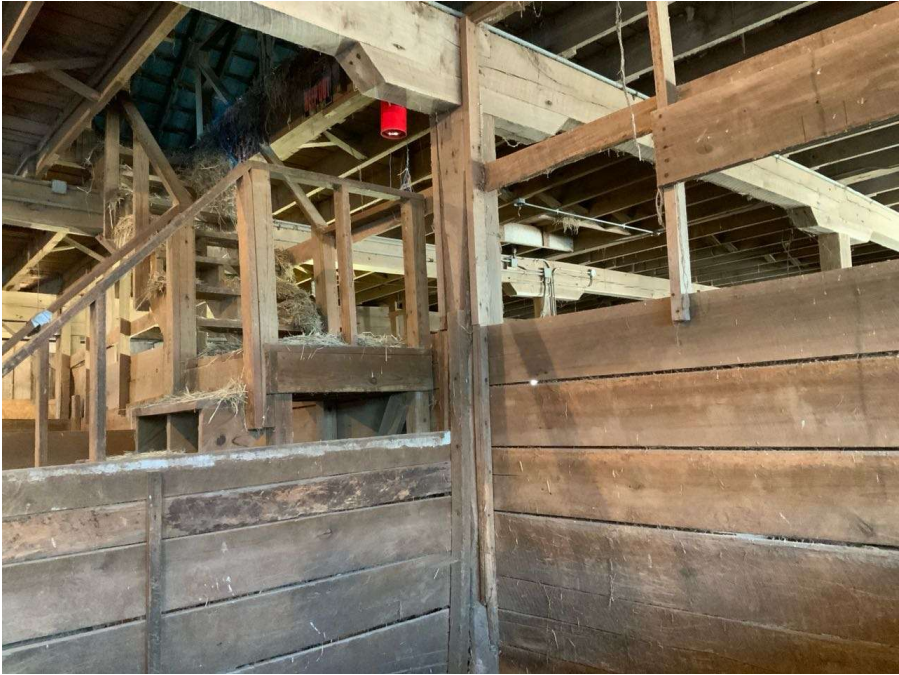
Photo G-4: General view of the stairs to hayloft in the east wing.
