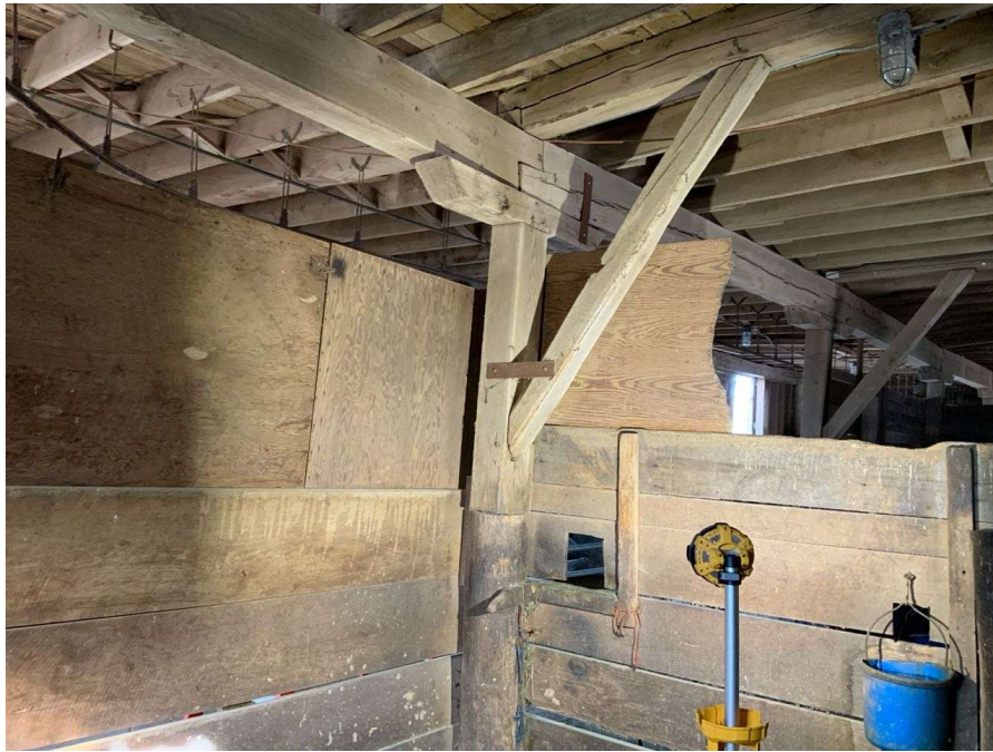
Photo S-131: The south brace at Column C/2 at grade level has a retrofit strap at the base connection to keep the brace attached (looking northeast).
