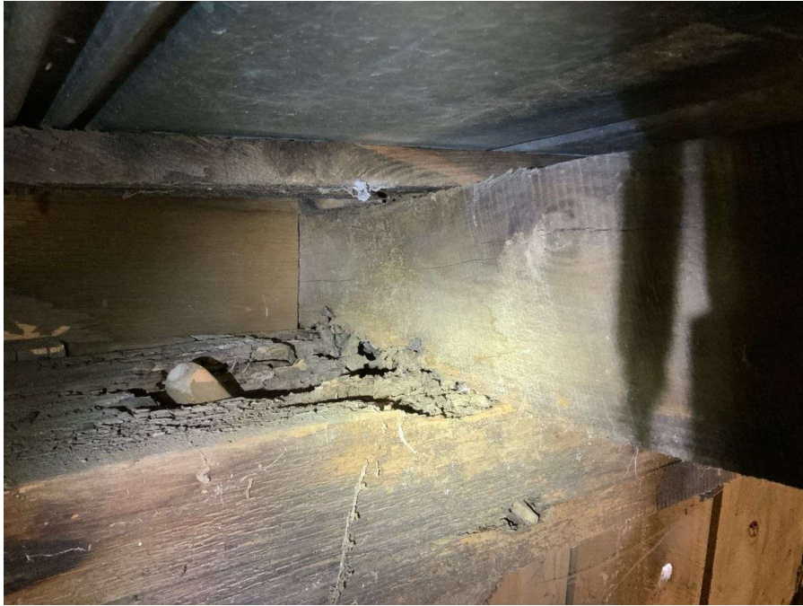
Photo S-23: Roof beam between Columns M/7 and N/7 exhibits rot with significant section loss under roof stringer. Note the icepick is fully inserted in top of beam.
