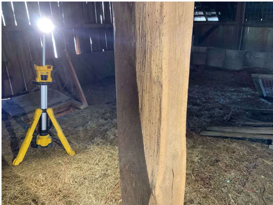
Photo S-36: Small holes at the base of the columns in the hayloft likely from insects or animals. Column C/3 looking northwest shown.
