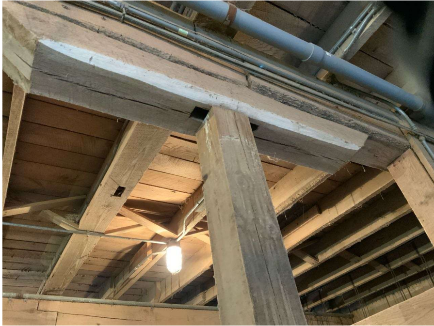
Photo S-115: Replaced column at Column O/2 at grade level has no positive connection to the cap at the top. Note the empty mortise slot in the floor beam indicating that the brace for this column is missing.
