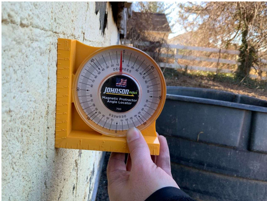
Photo S-152: Tilt in west elevation CMU foundation wall (looking south).
