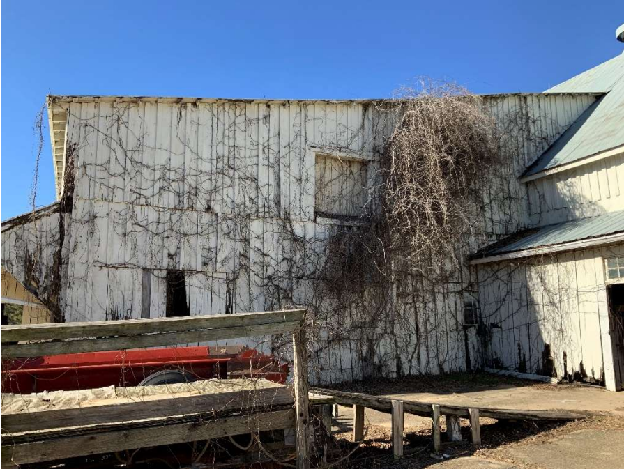
Photo A-10: General exterior photo of wood decay and overgrowth.
