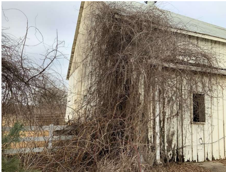
ES Photo 2: Heavy Vegetation pushing up roof deck along southwest corner (REF Photo S113)
