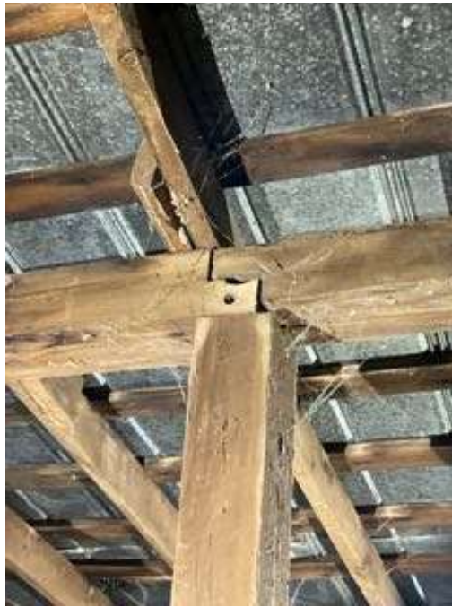
Photo S-29: Roof beam dowel is deteriorated/missing at Column M/5 (looking south).
