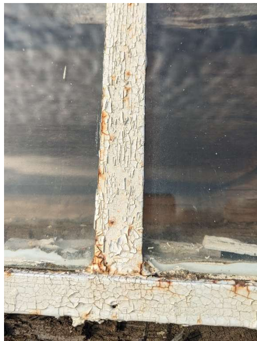
Photo E-6: "Alligator texture" cracking observed on white paint on exterior window frames. Identified as potential lead-based paint.
