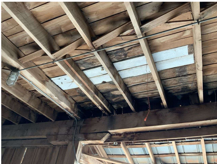
Photo S-66: Typical rotting floorboards. East wing near Gridline 4 shown looking south.
