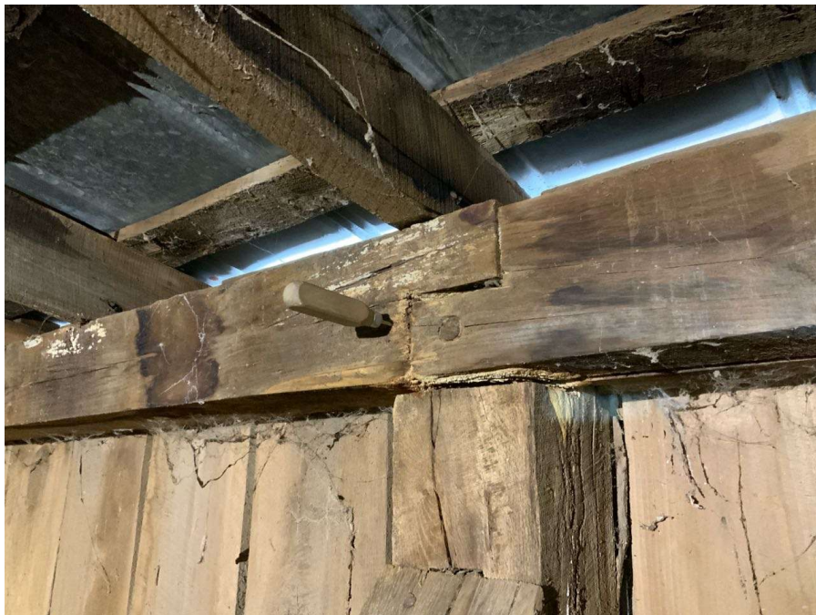
Photo S-22: Roof beam between Columns K/7 and L/7 exhibits rot with up to 4" deep ice pick penetration at west bearing.
