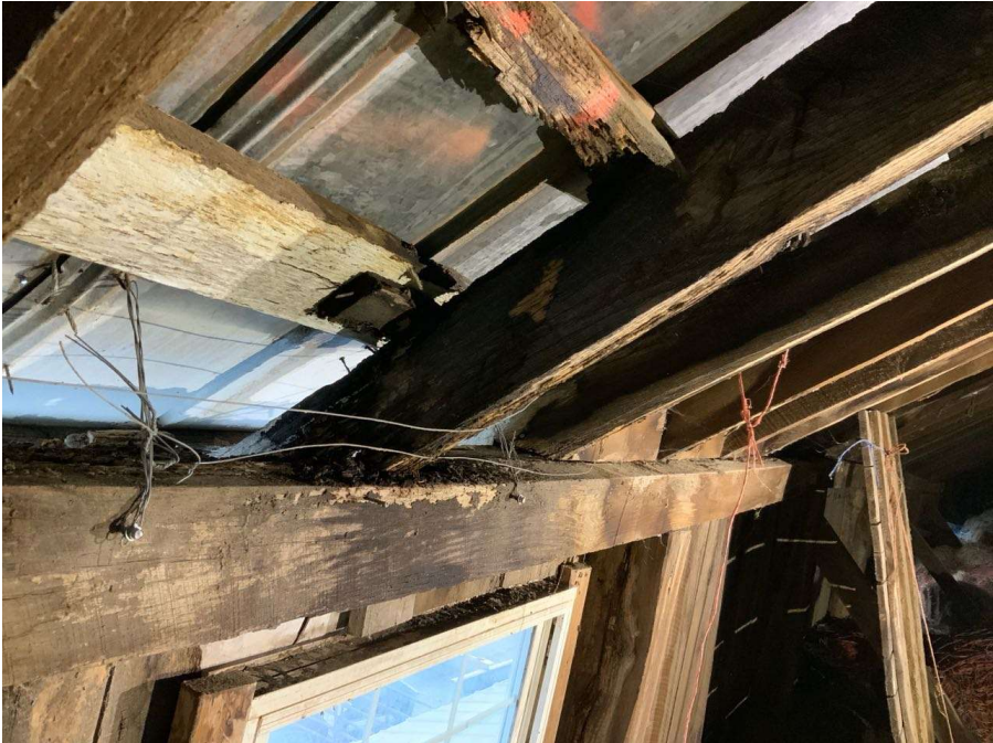
Photo S-10: Rotted rafters with full icepick penetration along Gridline 4 between Gridlines R and S.
