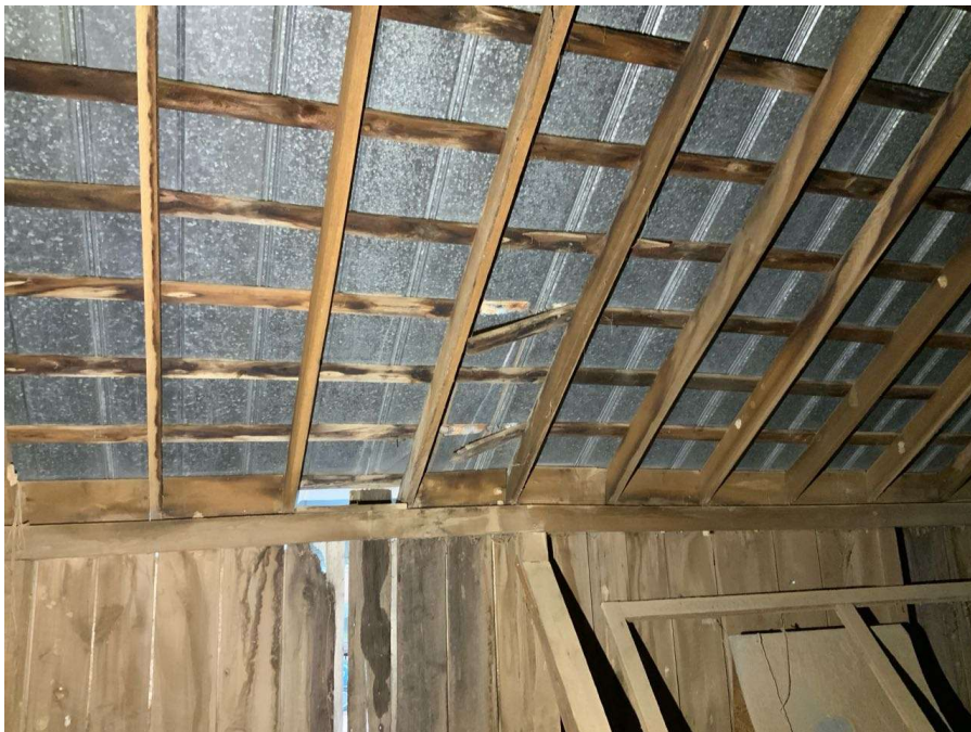
Photo S-8: Typical water saturated and broken roof purlins. Roof near Column F/4 shown looking southwest.
