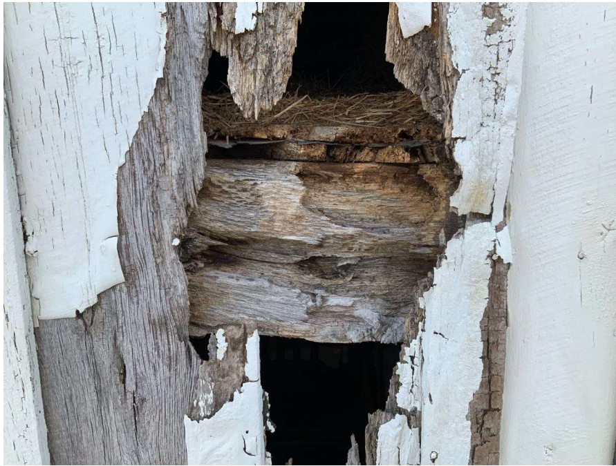
Photo S-93: Area of water damage and rot with approximately 25% section loss near north end of floor beam. Beam between Columns T/2.5 and T/3 shown looking west.
