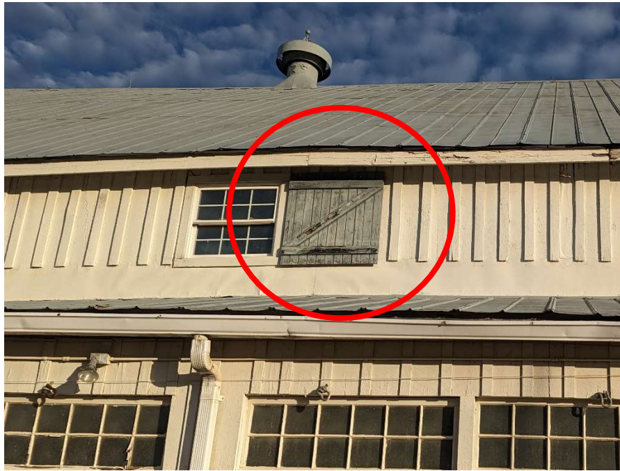
Photo E-5: Faded/peeling gray paint on wooden exterior window shutters. Identified as potential lead-based paint.
