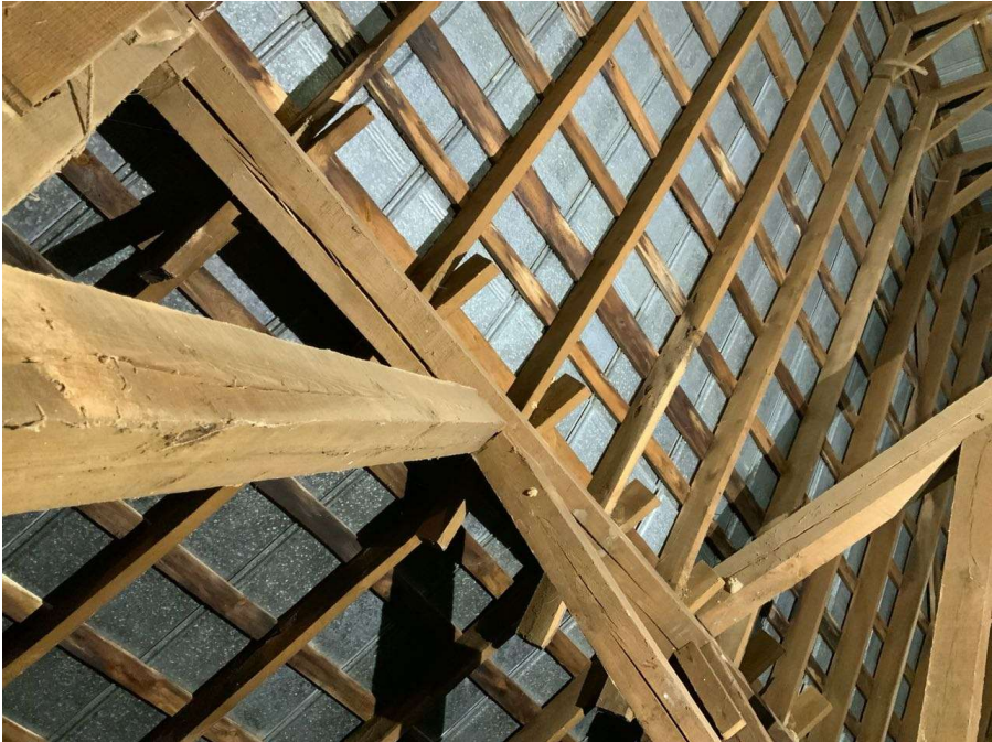
Photo S-25: Typical check on bottom face of interior roof beam. Roofbeam between Columns I/3 and J/3 shown.
