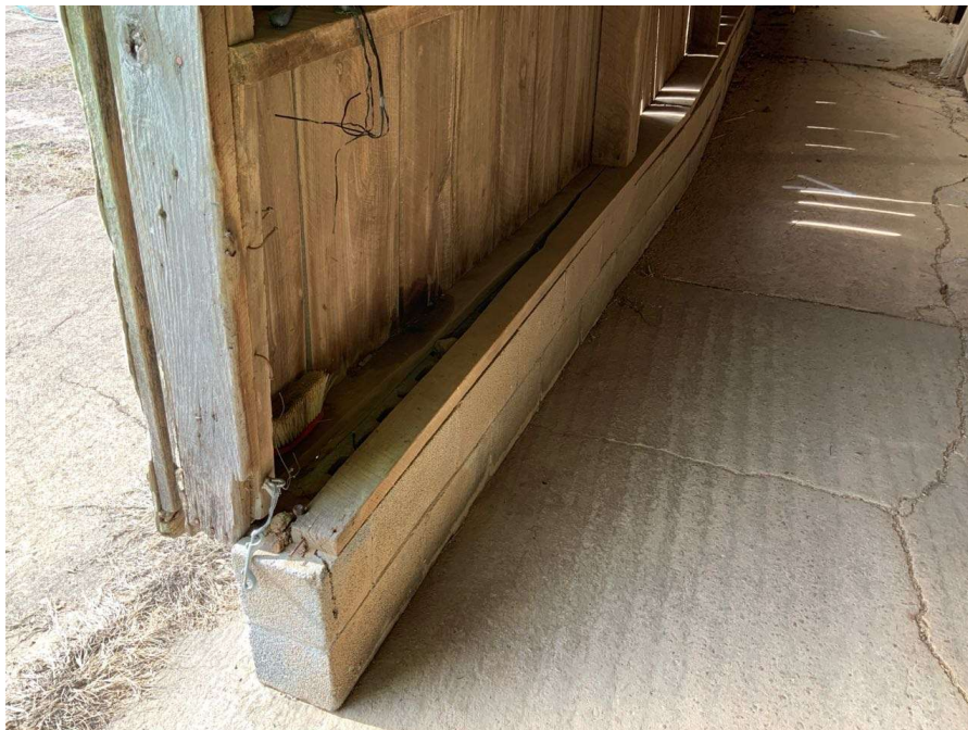
Photo S-164: The curtain wall between Gridline Q and R is pulled outwards and has misaligned CMU wall and split sill plate (looking west).
