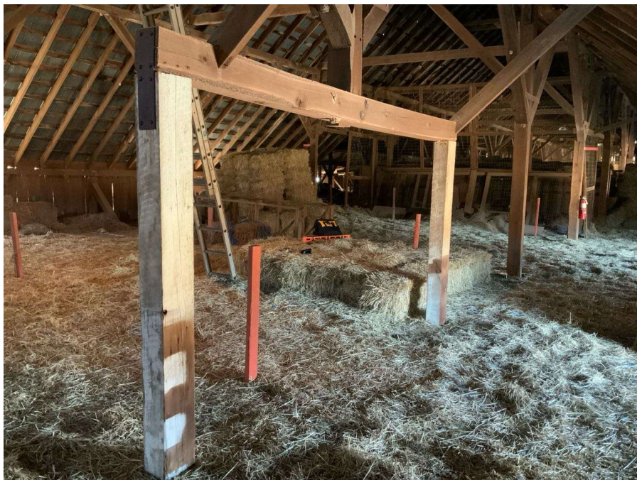
Photo G-10: General view of a load transfer spreader beam structures in the hayloft. Structure at Column Q/2 shown looking southwest.
