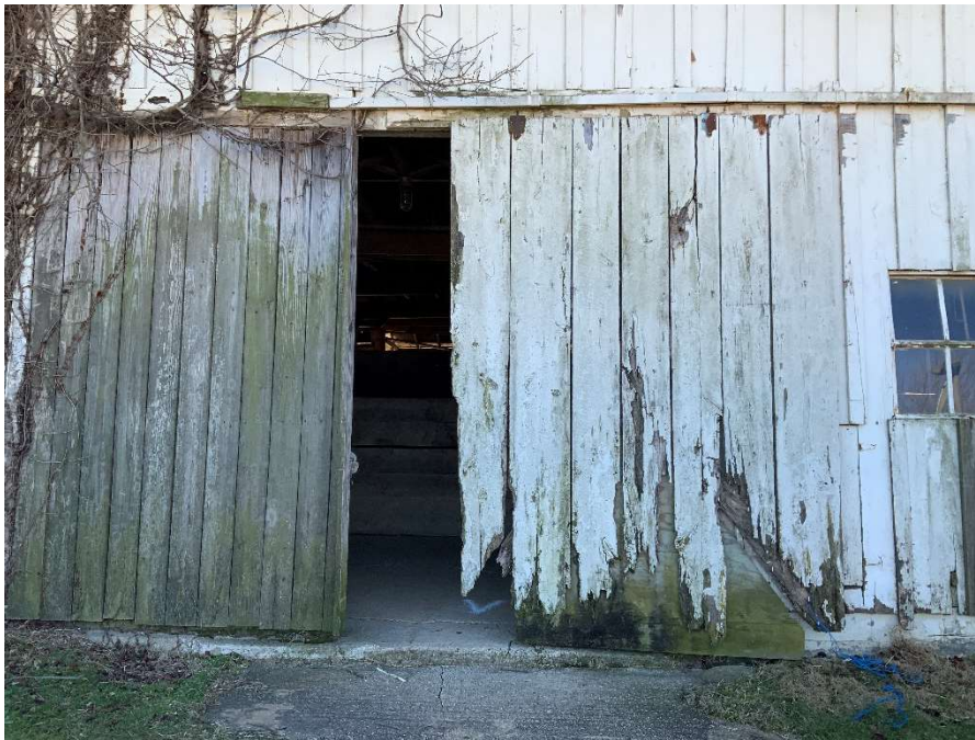
Photo A-22: General exterior photo of sliding door deterioration and decay.
