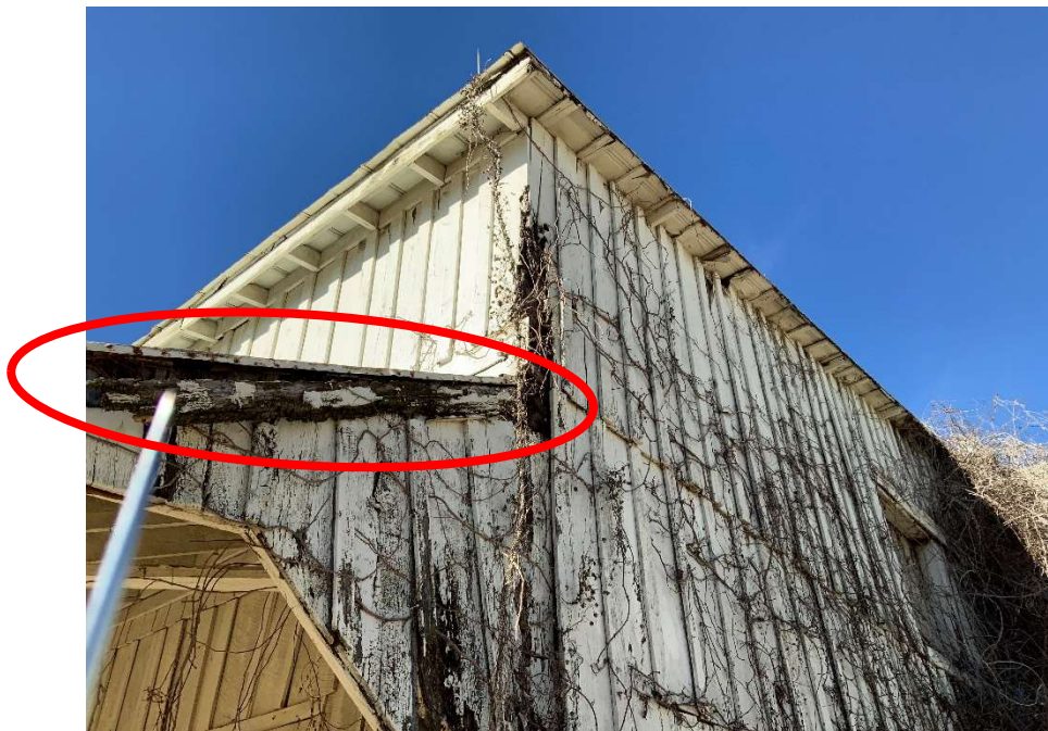
Photo A-6: Lack of edge coverage and wood deterioration.
