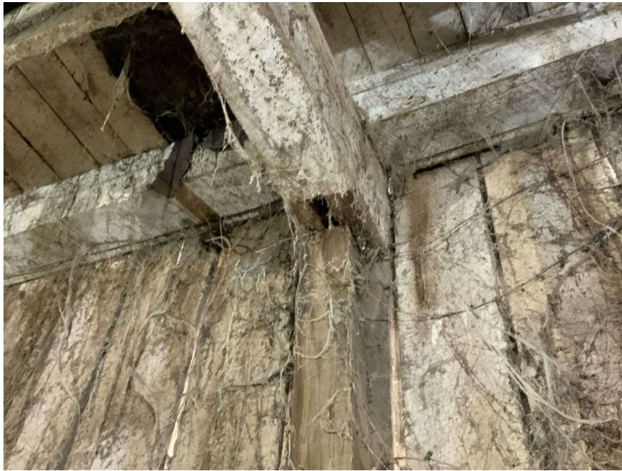
Photo S-117: The replaced column at Column N/5 at grade level has no positive connection to the cap at the top. Note the west brace is missing.
