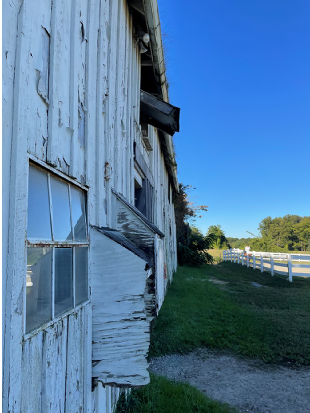
Leaning to left in photo (south). Note vegetation.
