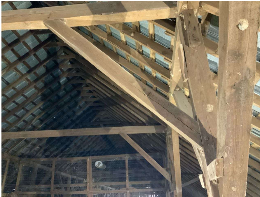
Photo S-53: Split in the south brace of Column P/2 in hayloft (looking west)
