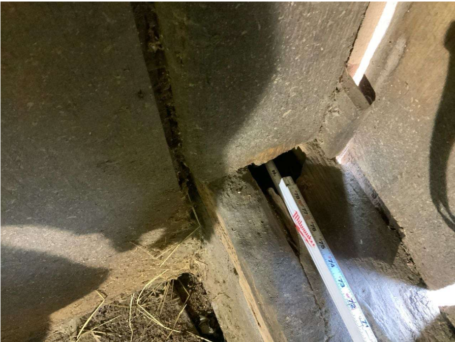
Photo S-144: Rot with section loss in the sill plate below Column B/2.5 at grade level.
