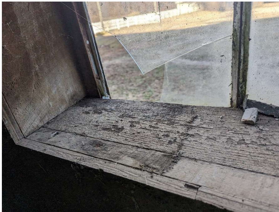
Photo E-10: Cracking/flaking white paint on interior wooden window sills throughout barn. Identified as potential lead-based paint.
