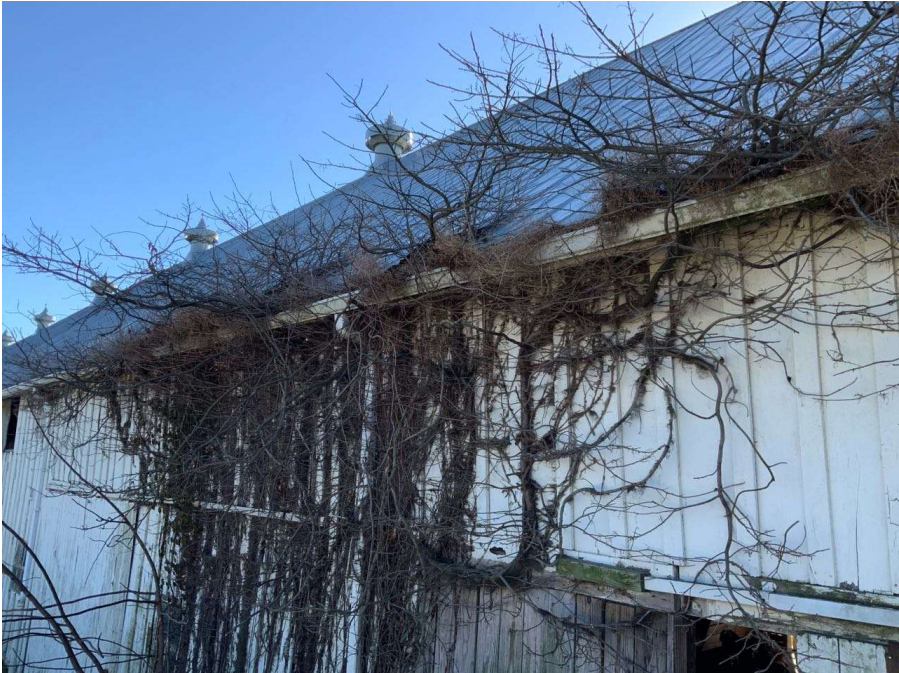
Photo S-5: Heavy vegetation pushing up roof deck along north elevation between Gridlines D and H (looking southeast).
