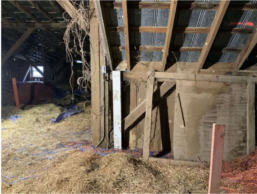
Photo S-41: New column and posts supporting wind girt and roof beam at Column H/4 in hayloft (looking south). Note the west brace is connected to the base of the original column.
