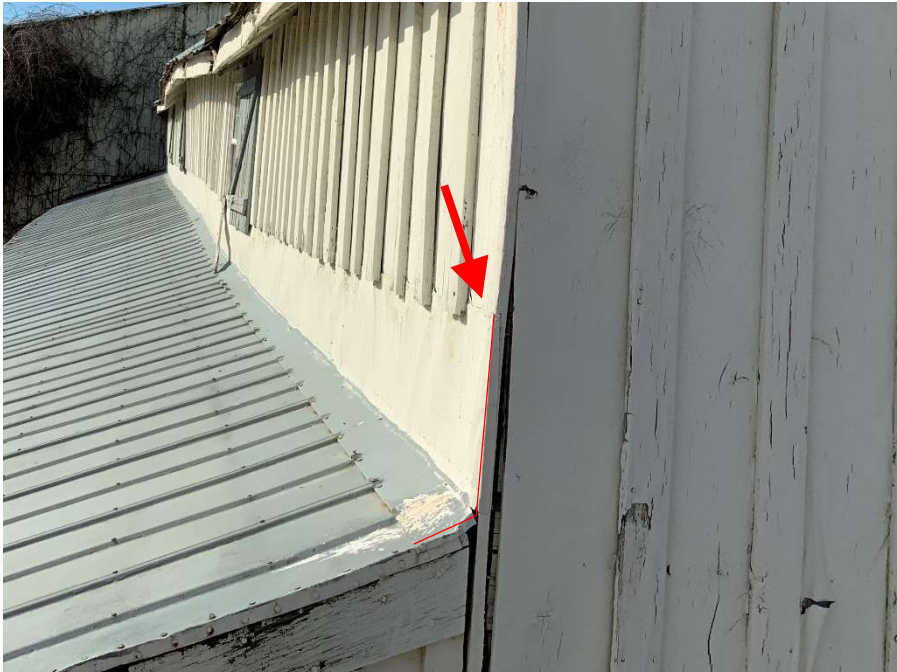
Photo A-8: Metal trim between the roof and wall connection lacking adequate sealing properties.
