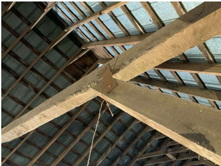
Photo S-56: South brace at Column F/2 in the hayloft is disconnected at the top connection to the horizontal frame member. The brace is no longer within the slot and held up by a single steel strap (looking west).
