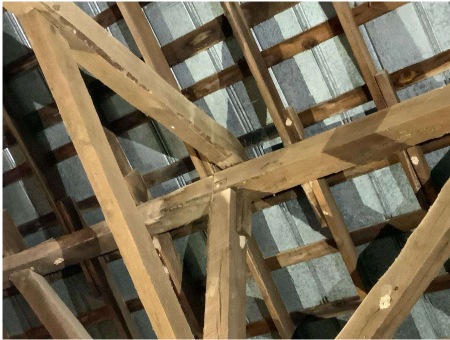
Photo S-33: Horizontal framing member south end is lifted up and not fully bearing at support in hayloft. Member at Gridline P looking southeast shown.
