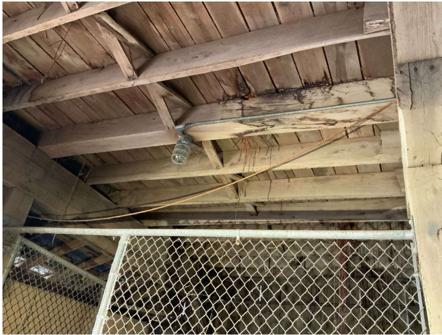
Photo S-91: Area of water damage and rot near north end of floor beam. Beam between Columns C/3 and C/4 shown looking west.
