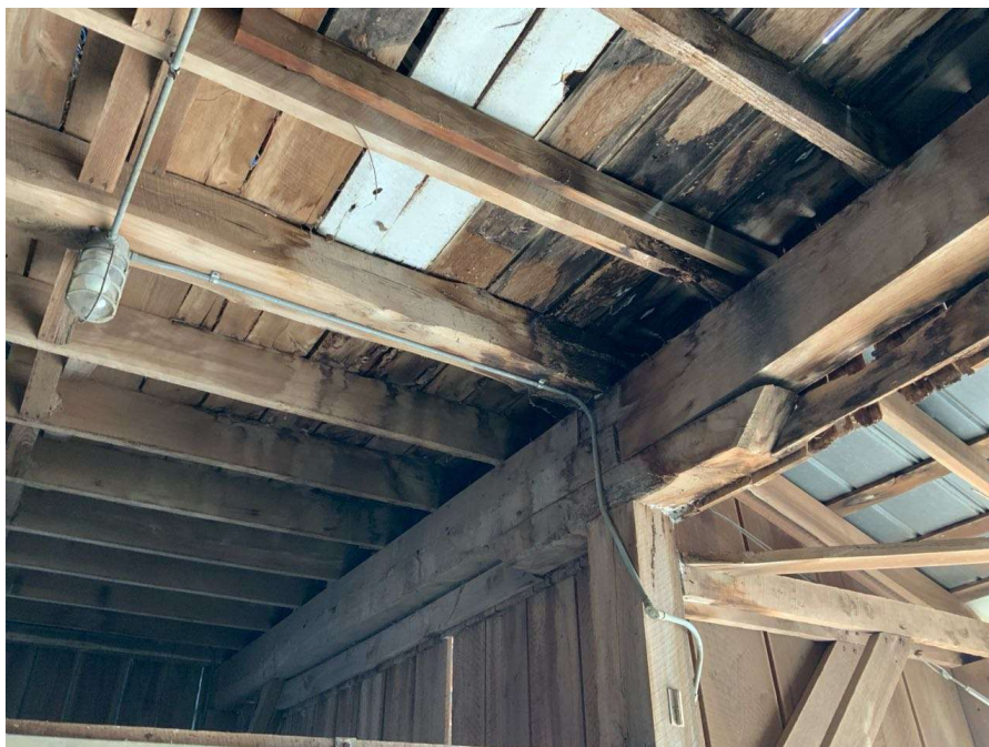
Photo S-70: Rotting floor stringer bearing on floor beam spanning between Column R/4 and S/4 (looking east). Note a sistered member has been added to this stringer.
