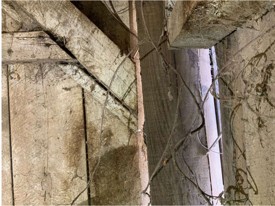
Photo S-127: The east brace at Column H/7 at grade level is not positively connected to the column at the base connection (looking south).
