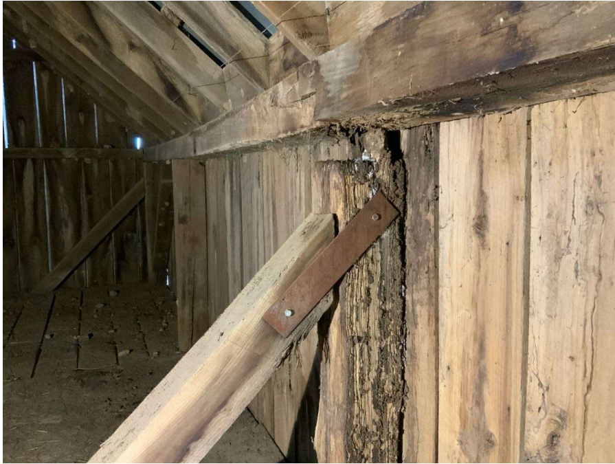
Photo S-19: Column S/4 at hayloft level has 3" gap at bearing between beam and column with minimal to no bearing remaining. The column is rotted and is dropping out of the mortise slot in the roof beam.
