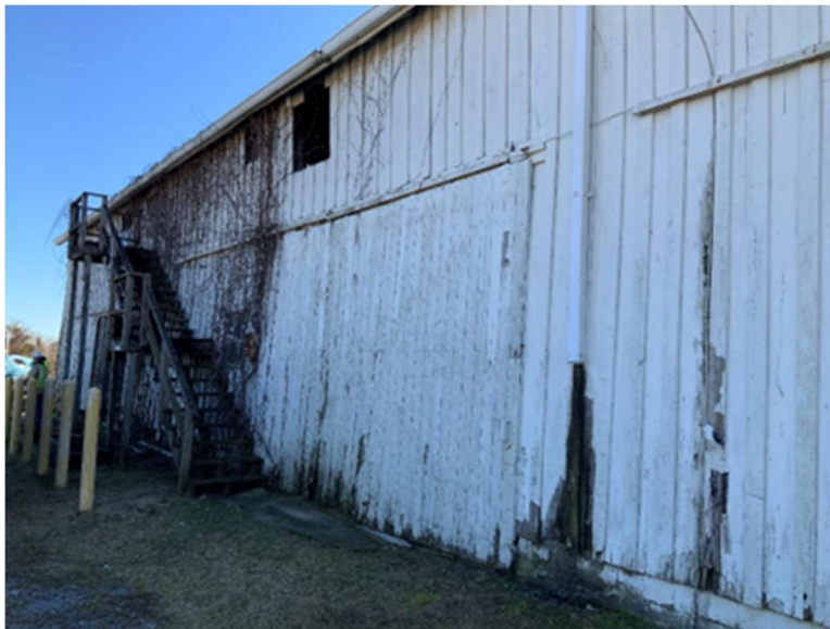
ES Photo 14 – Gutter clogged with vegetation, deteriorated boards and discontinuous rain leader (REF Photo A14 – Appendix B3)
