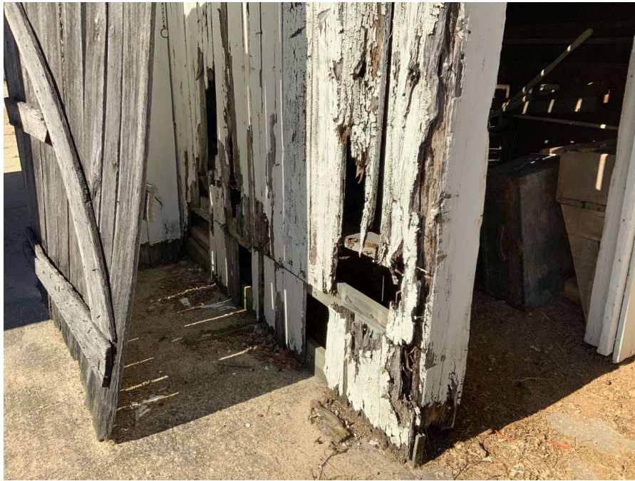
Photo S-161: The wall bump out between Gridlines K and L has rotting siding near the base and a rotting east end post.
