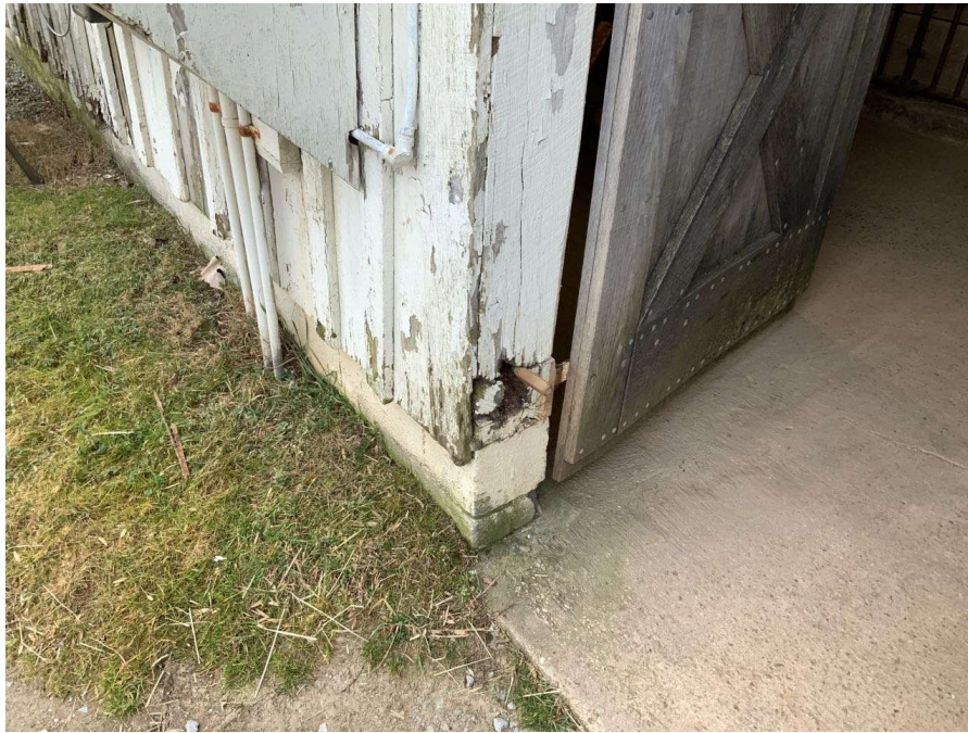
Photo S-147: Rot with full icepick penetration in the sill plate below east jamb near Gridline K/1 at grade level.
