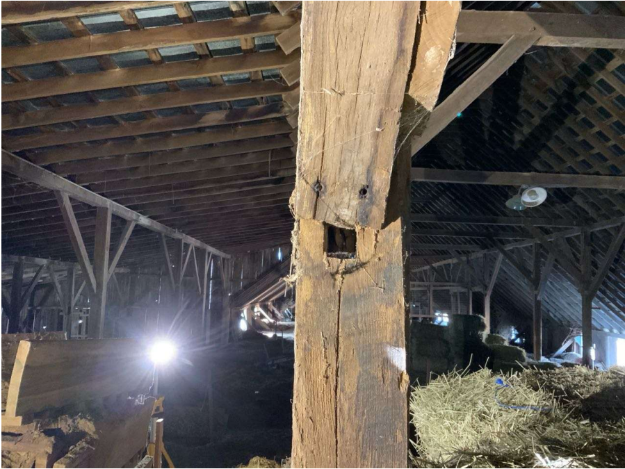
Photo S-47: Disconnected and twisted east brace at Column M/3 in hayloft (looking west).
