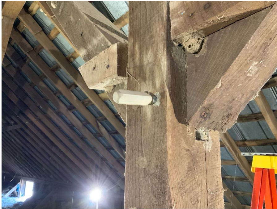
Photo S-45: Typical empty dowel hole in brace to column connection in hayloft. Column P/2 shown looking northwest. Note the icepick can fully penetrate the opening with no resistance.
