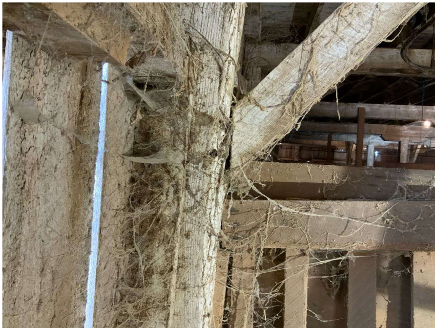
Photo S-126: The east brace at Column H/6 at grade level has a gap at the base connection to the column (looking north).
