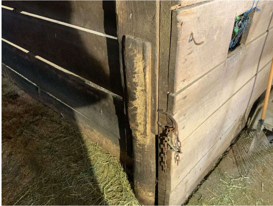
Photo S-119: The bottom portion of Column D/2.5 at grade level consists of a round post spliced to the original column using timber boards.
