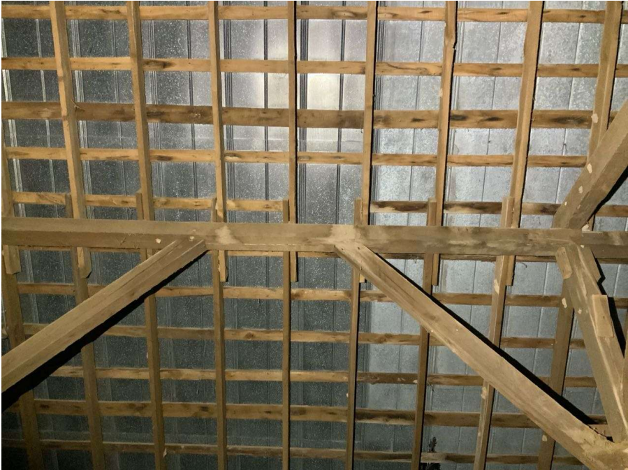
Photo S-9: Broken/missing roof purlin. Roof deck near Column L/2 shown looking north.
