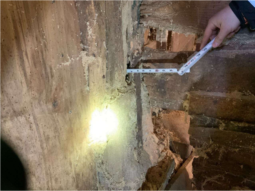
Photo S-105: Bearing loss at Column K/2.5 at grade level. Note this column is sitting on a pedestal.
