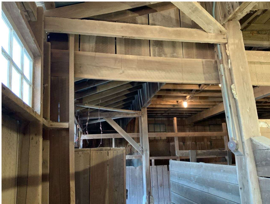
Photo S-142: Both overhang support diagonals and the west horizontal member is missing at Column P/4.
