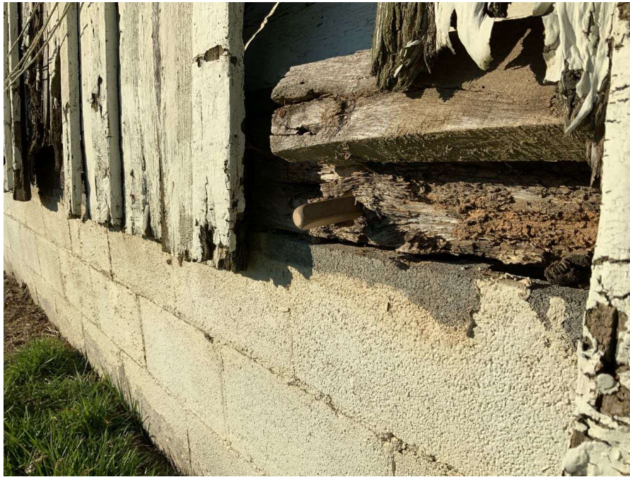
Photo S-151: The sill plate along Gridline T is rotting with up to full icepick penetration.
