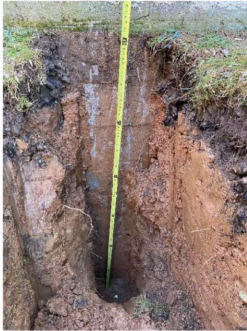
Photo GT-7: Top of concrete footing at TP-2 measuring 6.0 feet BGS with CMU foundation wall extending full depth and resting on top of spread footing.
