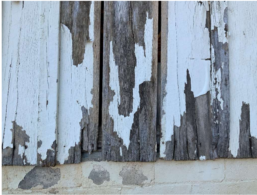
Photo A-11: Paint peel, missing battens, and exposed wood joints.
