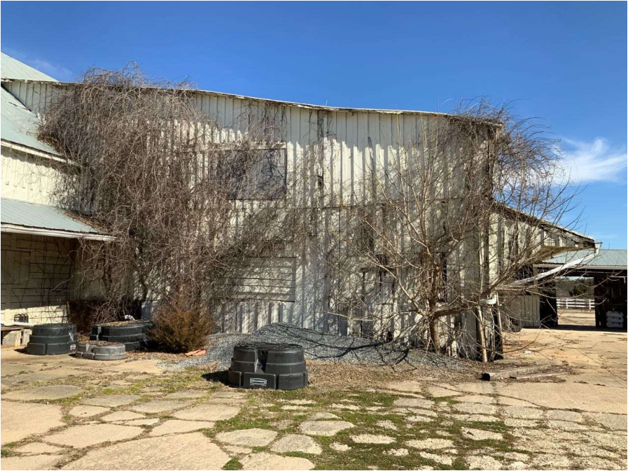
Photo S-171: Heavy vegetation growth on west elevation of lean-on structure.
