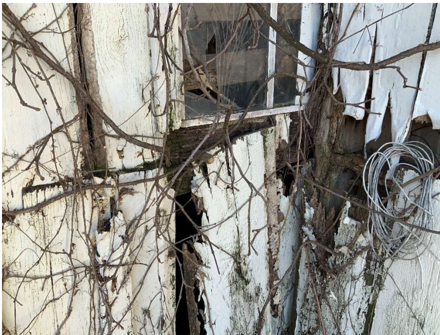
Photo A-16: Close-up photo of wood deterioration and overgrowth.
