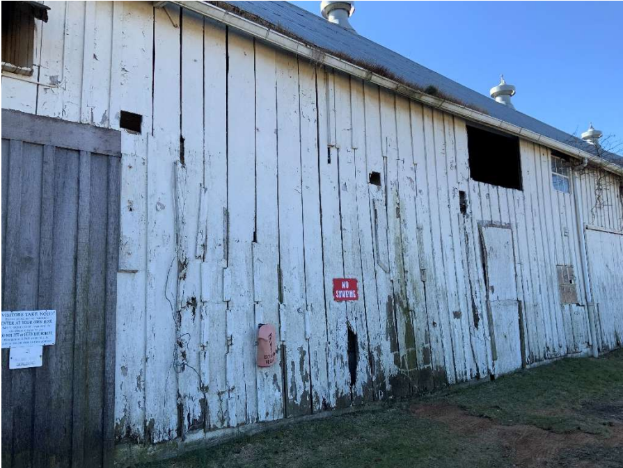
Photo A-13: General exterior photo of deteriorated and decaying boards.
