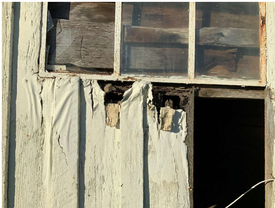
Photo A-20: Window damage and deterioration at sill.
