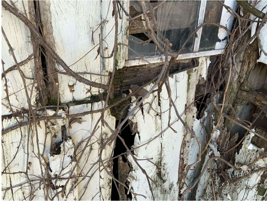
Photo S-169: Typical area of rot in the wind girt under the window opening. Wind girt between Columns N/4 and N/5 at grade level shown. There is up to full icepick penetration at this location.
