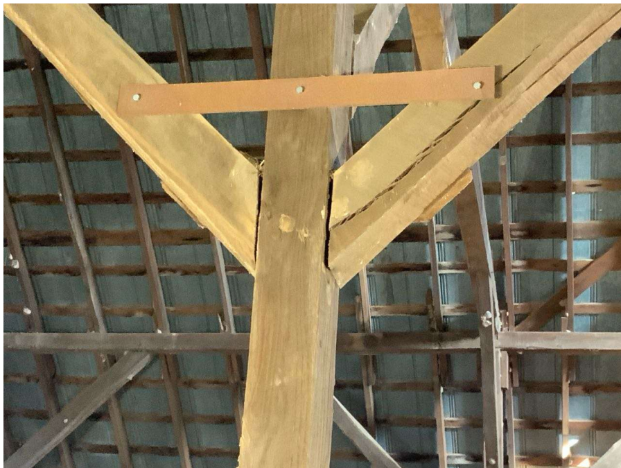
Photo S-46: Typical steel strap retrofit at hayloft brace to column connection. Column S/3 shown looking north.
