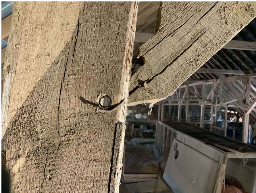
Photo S-54: South brace at Column E/2 in the hayloft is disconnected at the base connection to the column. The dowel hole is broken and only a small sliver of the brace is still within the mortise slot.
