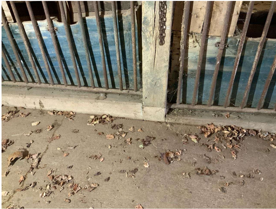
Photo G-15: General view of a grade level column supported by a concrete curb. Column J/4 shown looking east.
