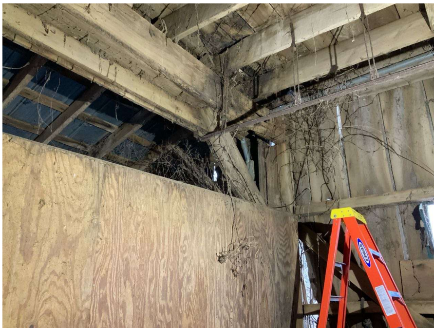
Photo S-80: Critical Finding at floor beam between Columns B/4 and C/4. The west end of the beam has approximately 90% section loss.
