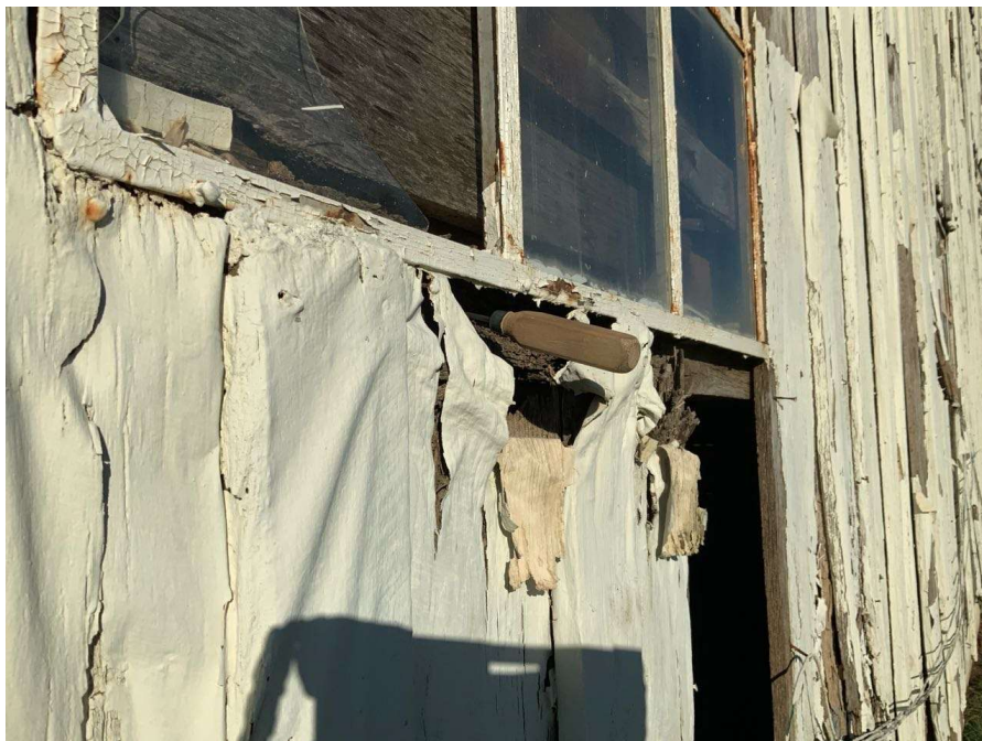
Photo S-168: Typical area of rot in the wind girt under the window opening. Girt between Columns T/3 and T/4 at grade level shown. Icepick penetration at this area is up to 3.5" deep.
