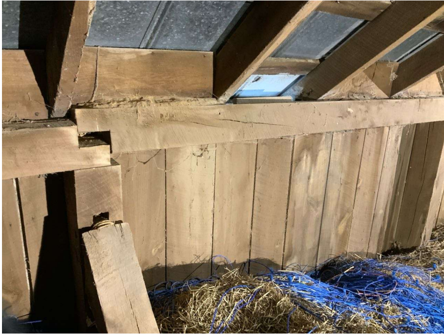
Photo S-17: Perimeter roof beam between Column N/4 and O/4 is twisting 7 degrees south at east bearing and has minimal to no bearing remaining.
