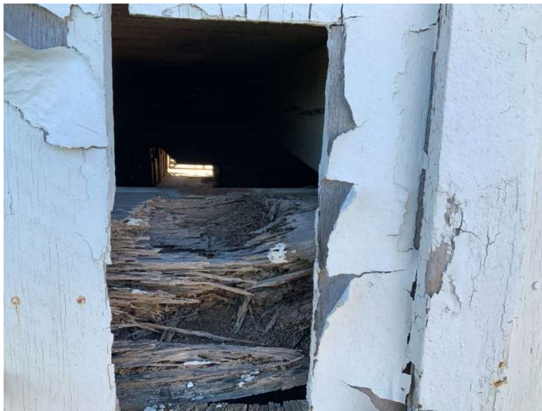
ES Photo 9 – Severe rot at floor beam – west end has significant section loss – (REF Photo S82 – Appendix B2)
