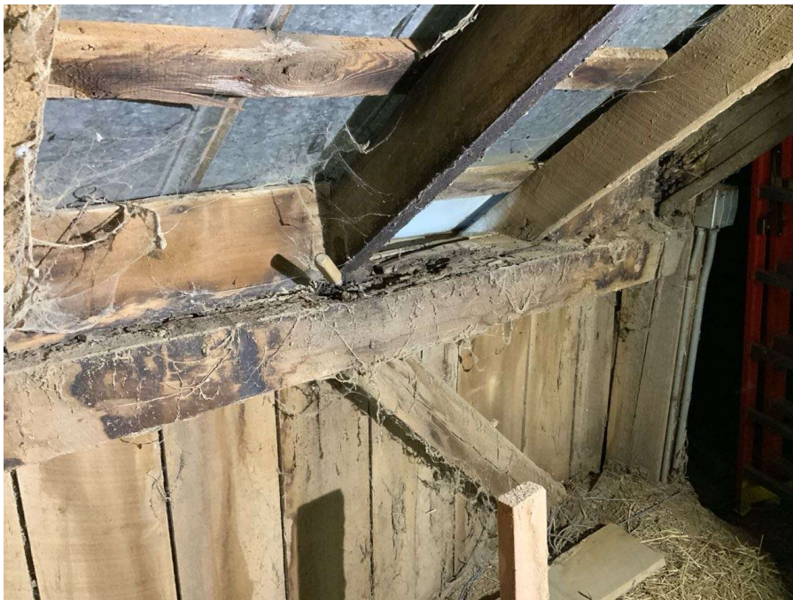
Photo S-24: Roof beam between Columns N/4 and O/4 exhibits rot with up to full icepick penetration in top face at west bearing over a 6ft length.
