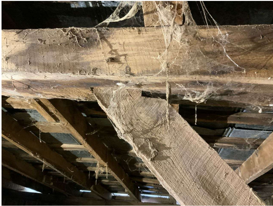
Photo S-49: East brace at Column H/6 in hayloft is slipping out of the mortise slot at the top connection to the roof beam (looking south).
