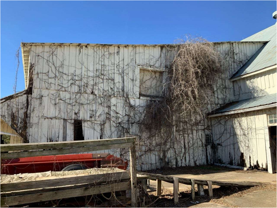
Photo S-172: Heavy vegetation growth on east elevation of lean-on structure.
