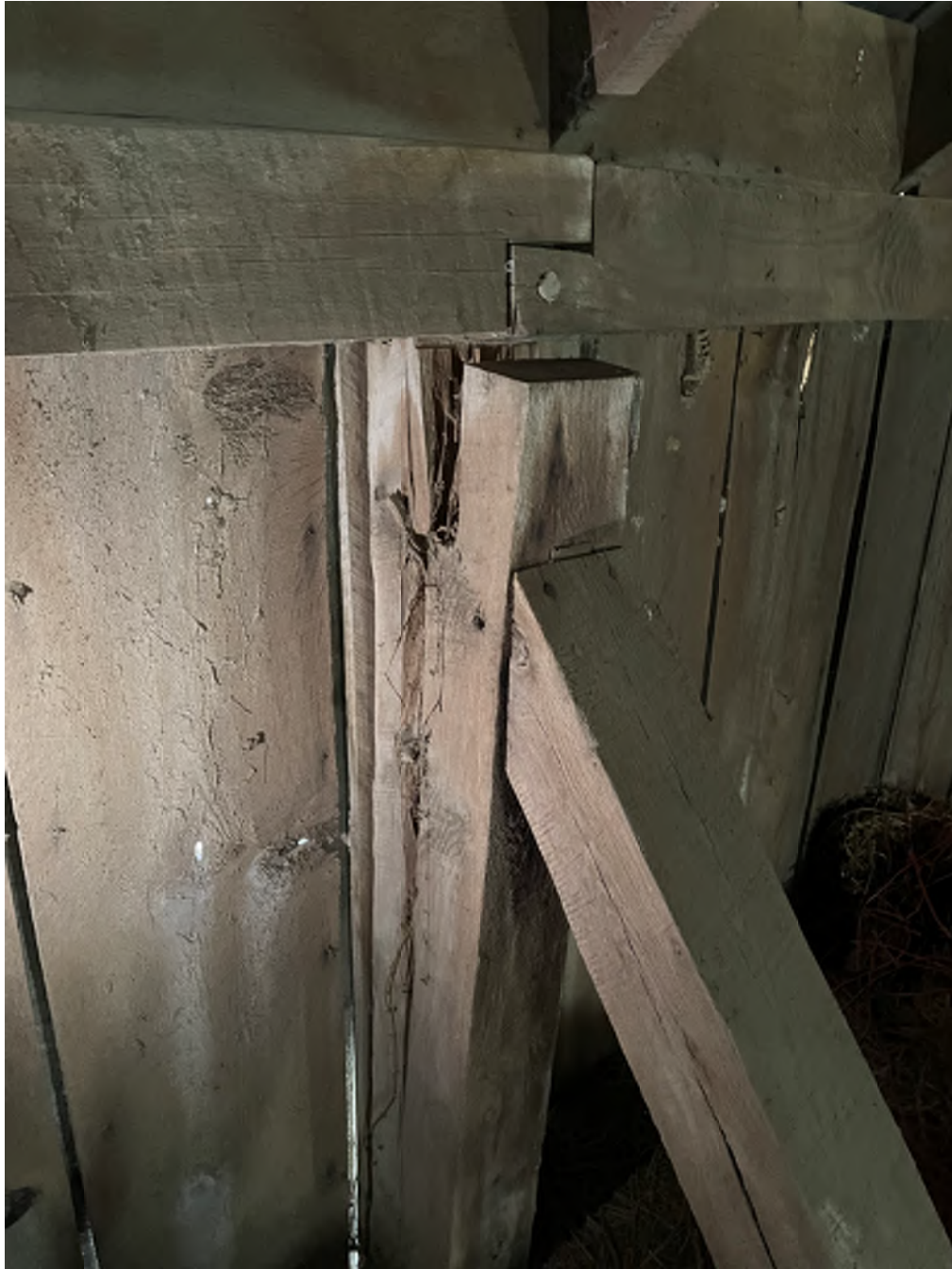
Damaged post in loft
