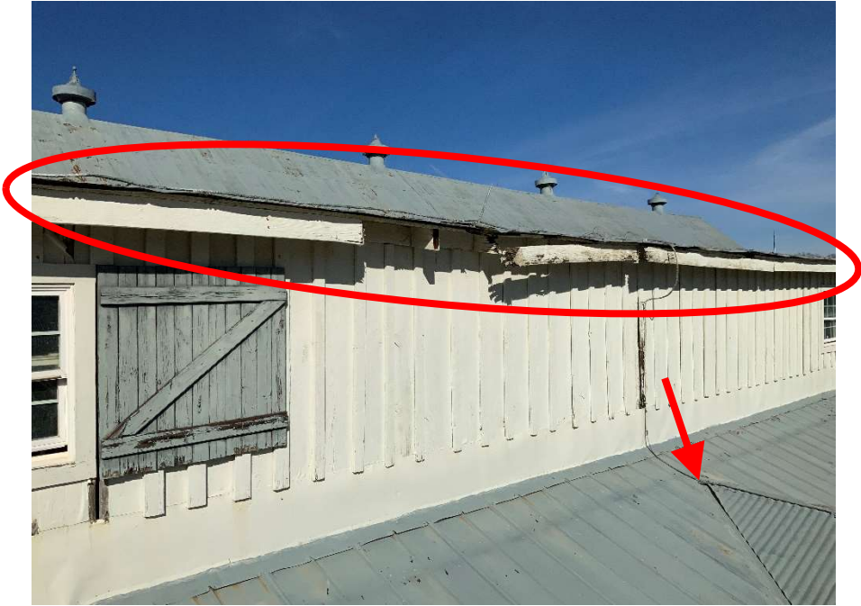
Photo A-4: Deteriorating roof edge and inadequate waterproofing at corrugated roof.
