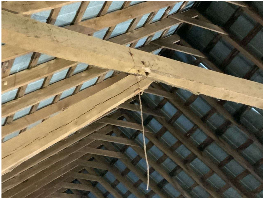
Photo S-55: South brace at Column F/2 in the hayloft is disconnected at the top connection to the horizontal frame member. The brace is no longer within the slot and held up by a single steel strap (looking east).
