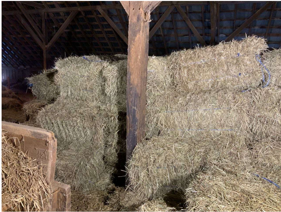
Photo S-35: Column M/3 in hayloft exhibits water staining and soft rot with minimal ice pick penetration (looking northwest).
