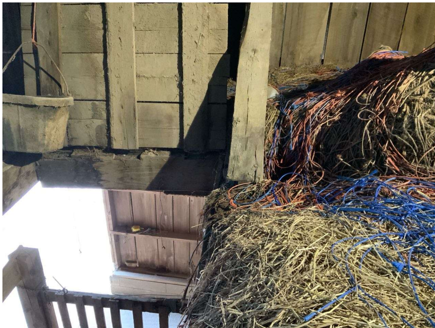
Photo S-60: North brace at Column R/4 in hayloft is disconnected at the base connection to the floor beam.
