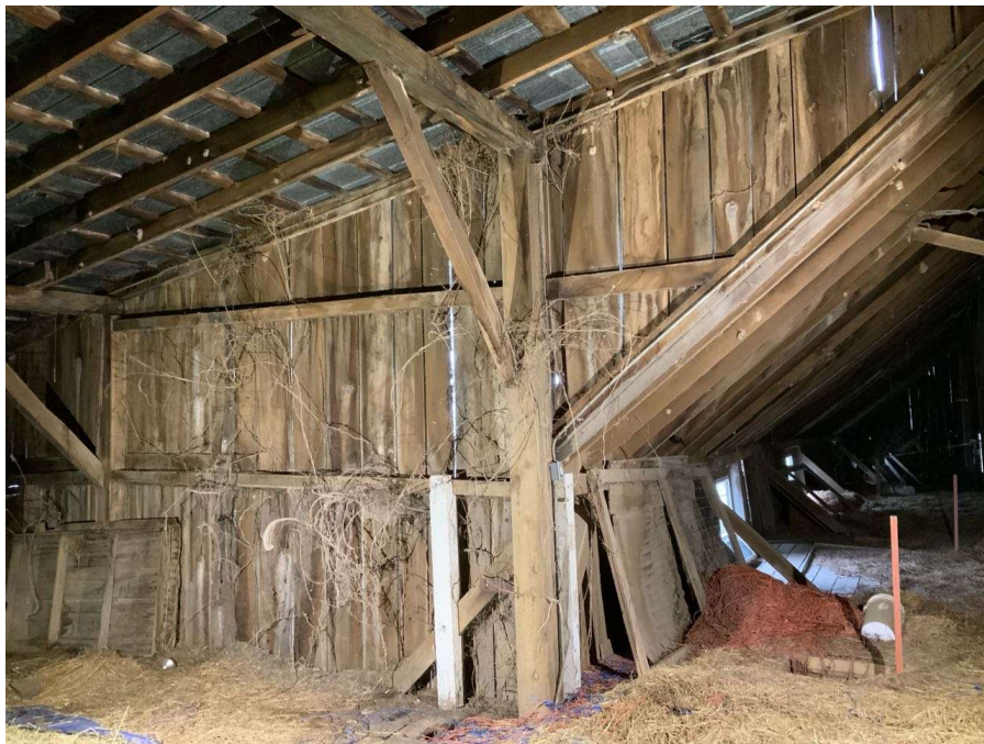
Photo S-40: New column and posts supporting wind girt and roof beam at Column H/4 in hayloft (looking southwest). Note the south brace is connected with an ineffective strap to the new column.
