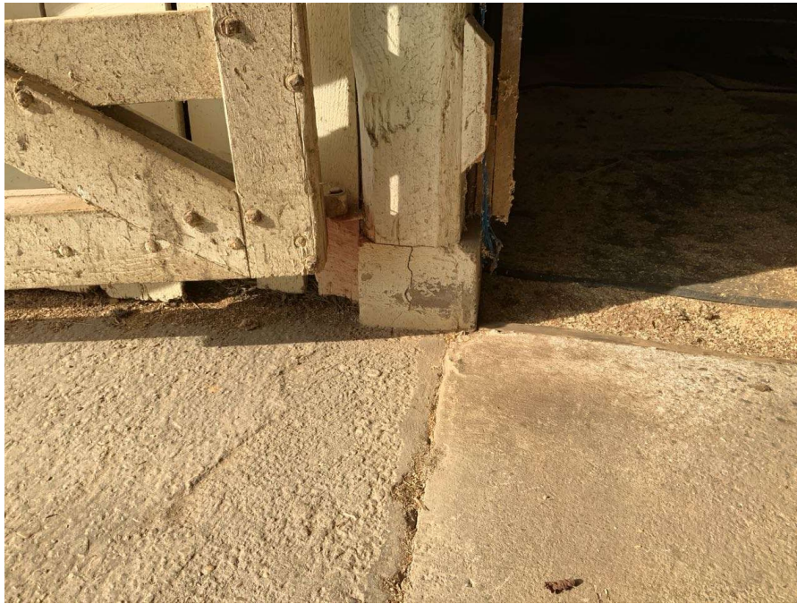
Photo S-157: Vertical crack in east face of the concrete curb supporting Column L/7 at grade level. Note that the column does not appear to be positively attached to the concrete curb.
