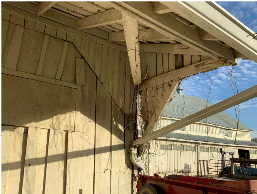
Photo S-140: The overhang support diagonal is disconnected at the base connection to Column N/7.
