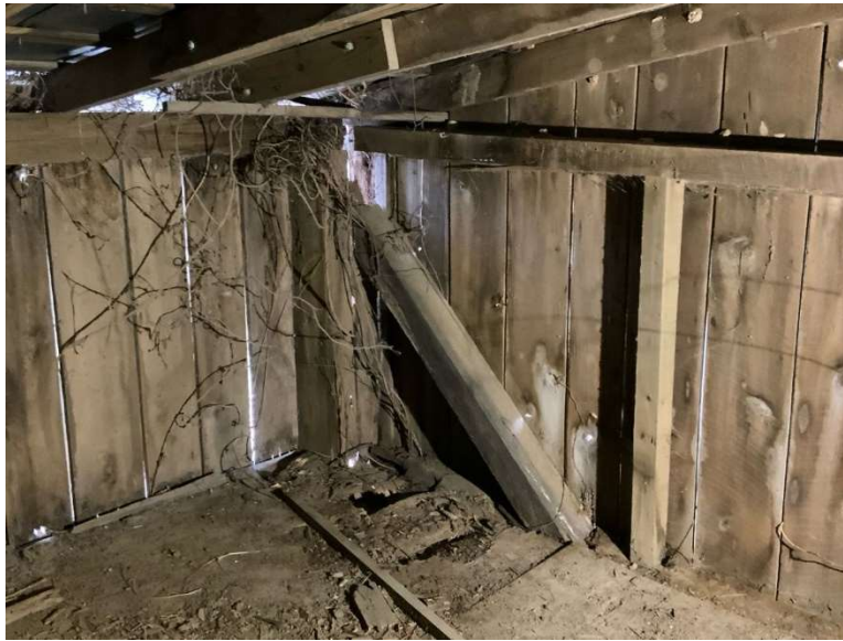
ES Photo 6 – Hayloft looking southwest – post has been added to east existing column., north brace and wind girt are not connected to the post and the east brace is missing. The floorboards adjacent to the column are rotting. (REF Photo S42- Appendix B2)
