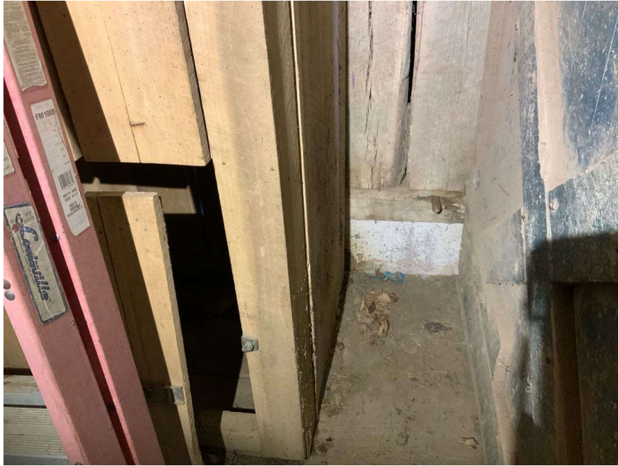
Photo S-145: Rot with full icepick penetration in the sill plate below Column H/1 at grade level.
