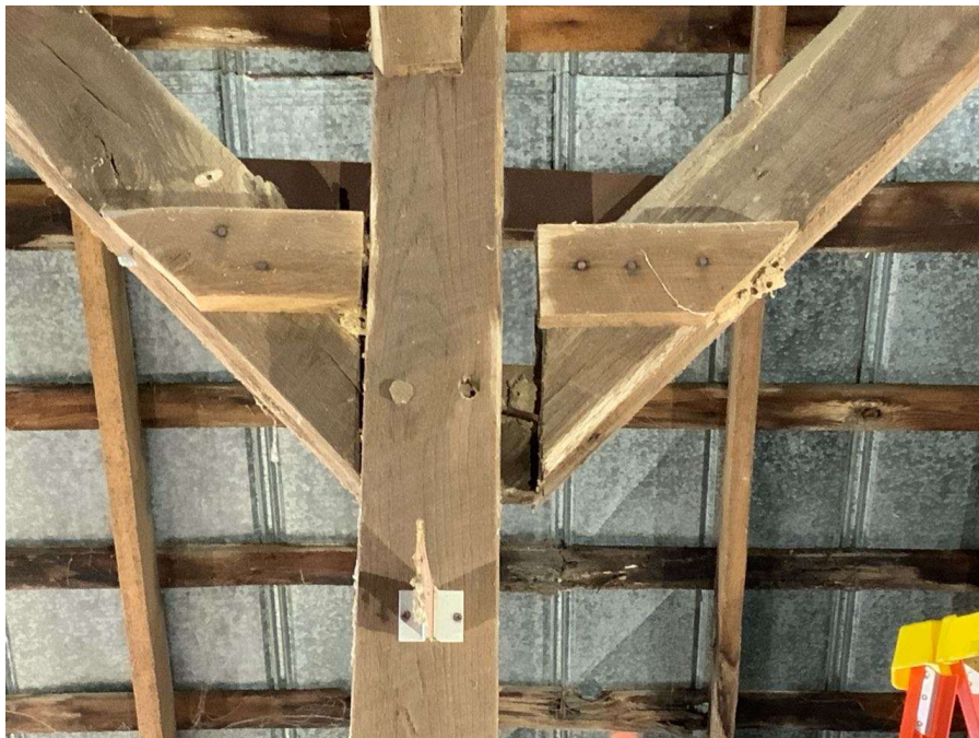
Photo S-50: The west brace at Column R/3 in hayloft is disconnected at the base connection to the column. The dowel at this connection is missing.
