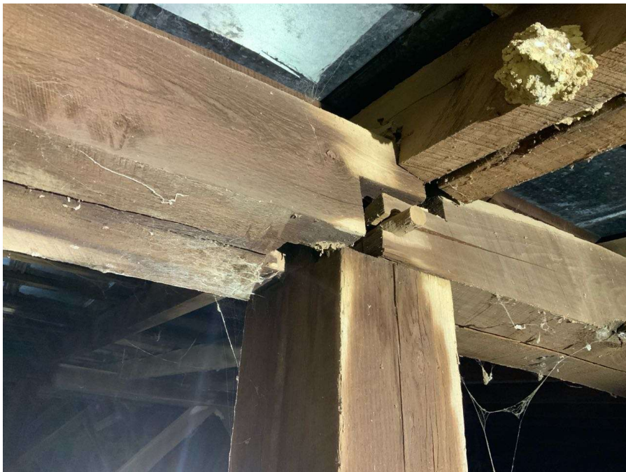
Photo S-28: Gap between roof beams at Column 1/6 bearing location (looking northeast). Note the west beam is twisting towards the north.
