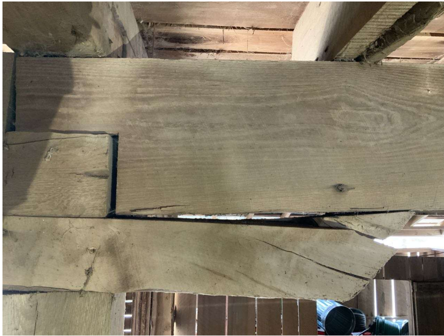
Photo S-77: Uneven floor beam at Column F/3 (looking south). West beam is not bearing on the cap and is only bearing on the east beam at notch. The column cap is split.
