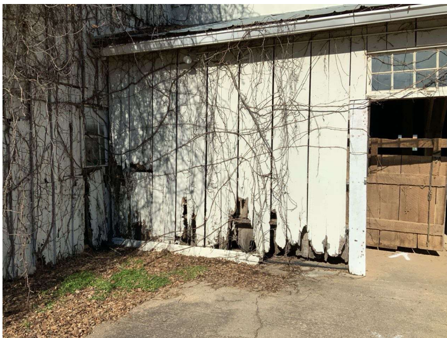
Photo S-162: The curtain wall between Gridline N and O has rotting siding and sill plate near the base. The wall moves when pushed.
