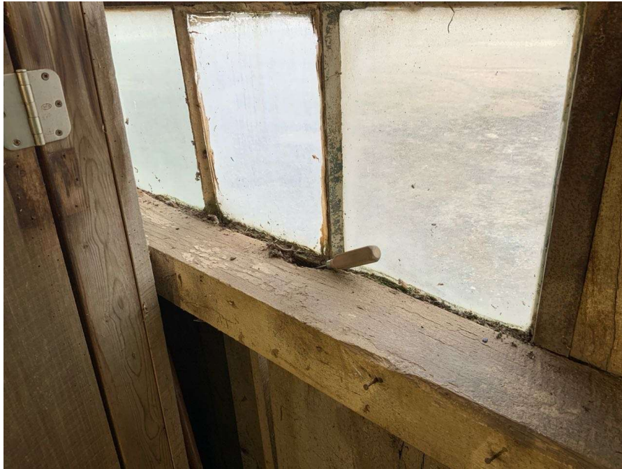
Photo S-167: Typical area of rot in the wind girt under the window opening. Wind girt between Columns M/1 and N/1 at grade level shown.
