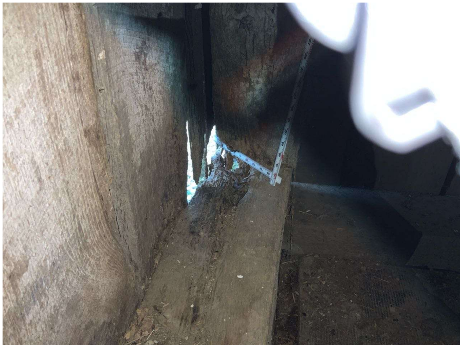
Photo S-112: Bearing loss at Column T/1 at grade level. The column has 50-75% section loss. The sill plate is deteriorated and rotting under the column.
