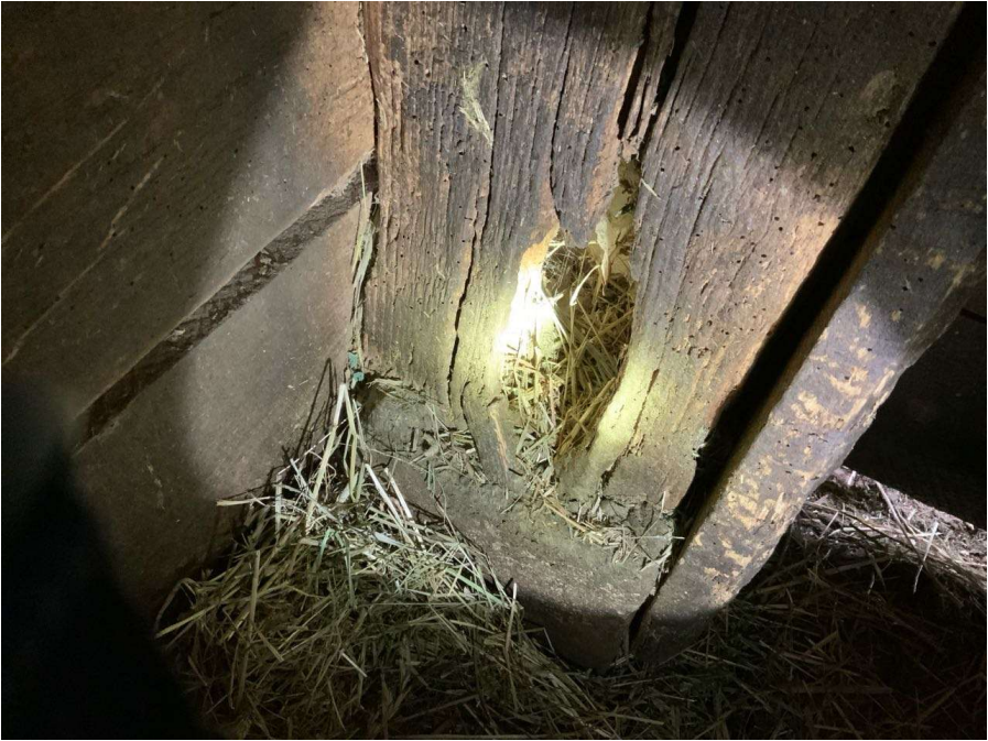
Photo S-102: Bearing loss at Column D/2 at grade level.
