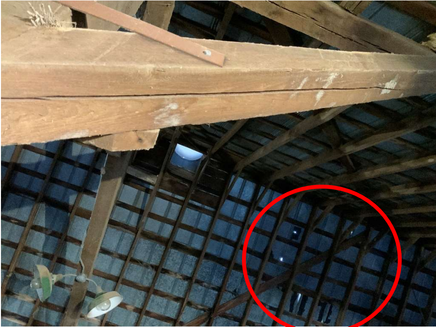
Photo A-2: Underside of metal roof panels with open cavities.
