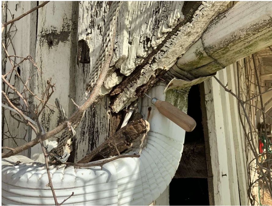
Photo S-137: The overhang support diagonal at Column H/7 exhibits rot at base connection with up to 4" deep icepick penetration. The diagonal is not fully connected to the column.
