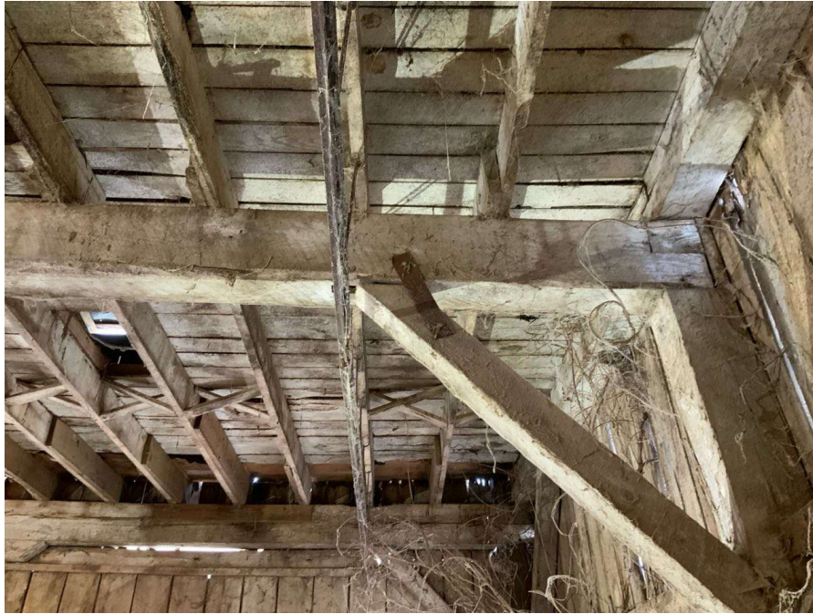
Photo S-125: The east brace at Column H/6 at grade level is slipping out of the mortise slot at the top connection to the floor beam (looking south). A retrofit strap has been added to keep it in place.
