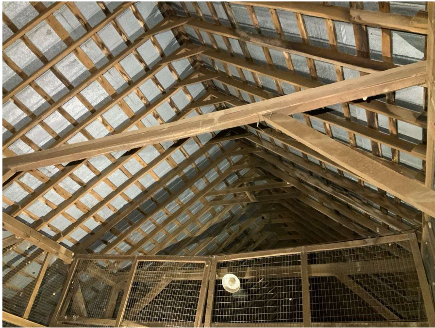
Photo S-31: Potential split at horizontal frame member between Columns G/2 and G/3 in the hayloft (looking east). The member appears to have excessive deflection compared to other similar members.
