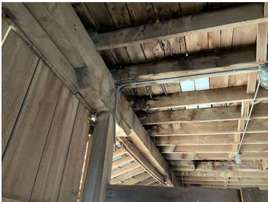
Photo S-92: Area of water damage and rot near south end of floor beam. Beam between Columns S/3 and S/4 shown looking west.
