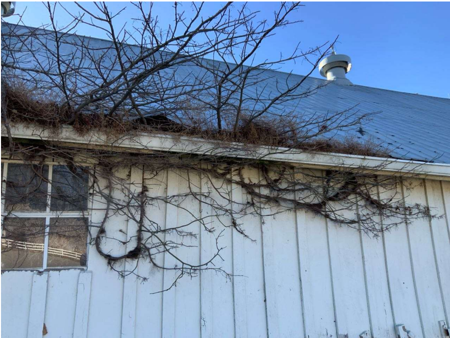
Photo S-6: Close up of heavy vegetation pushing up roof deck along north elevation (looking south).
