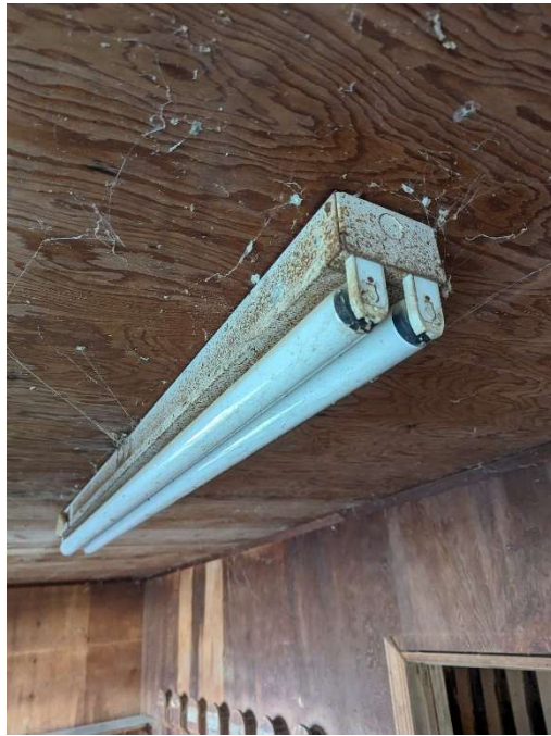
Photo E-13: Fluorescent light fixture in barn interior room along northern building wall. Ballast identified as potentially containing PCBs. Fixture was not opened for inspection due to its condition.
