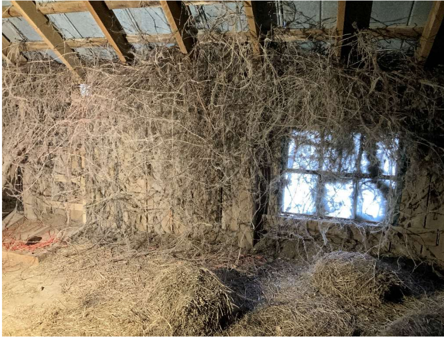
Photo A-17: Interior photo of vegetation overgrowth compromising the building envelope.
