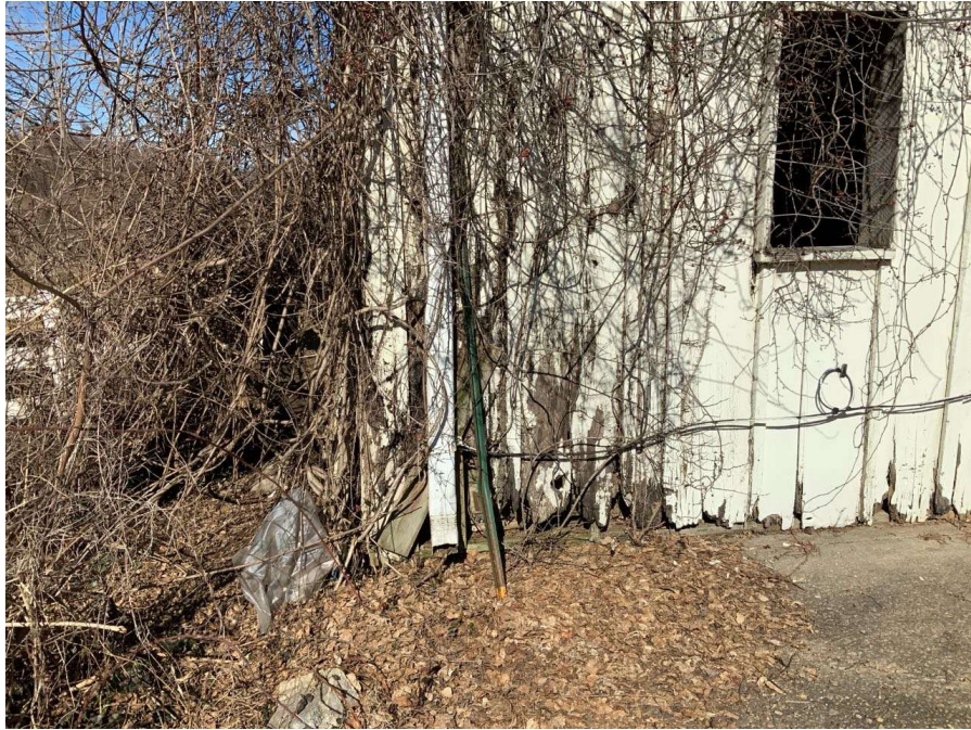
Photo S-159: Rotting siding along the bottom of the curtain wall bump out between Gridlines B and C.
