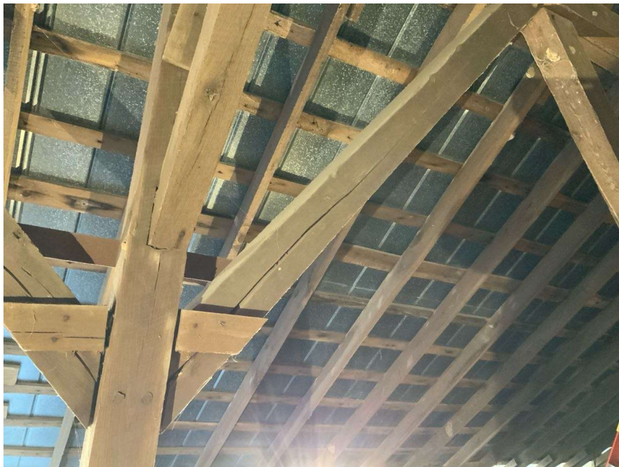
Photo S-44: Typical split starting at brace connection in the east/west braces in hayloft. East brace at Column I/2 shown looking north.
