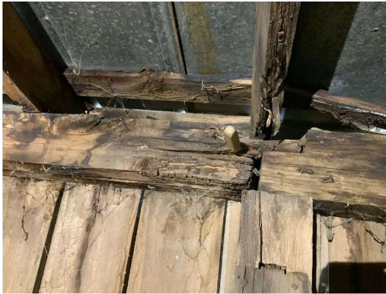
ES Photo 4 – Perimeter Roof Rot (REF Photo S21 – Appendix B2)
