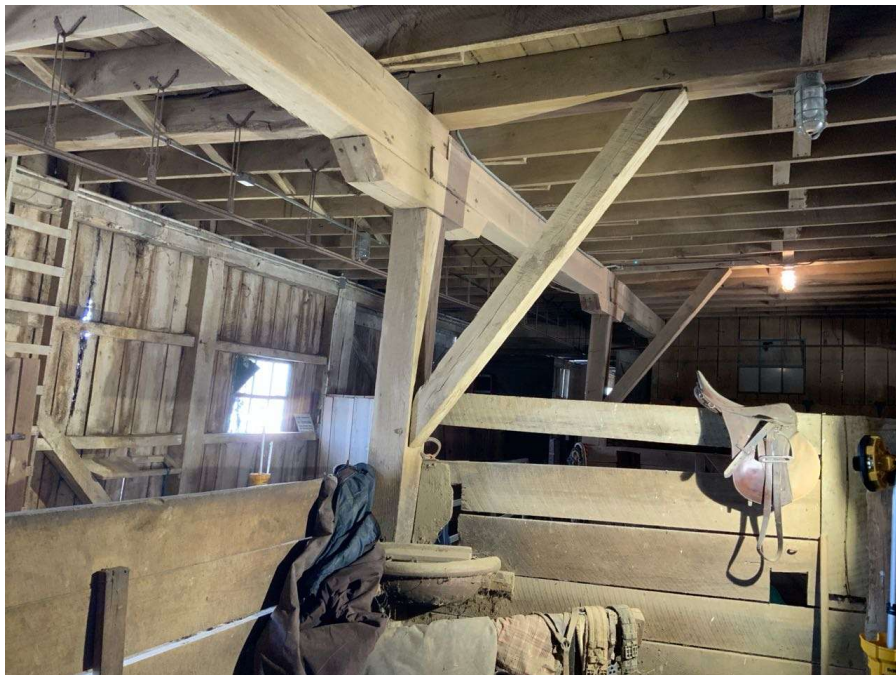
Photo G-12: General view of a knee braced column at the grade level. Column F/2 shown looking northeast.
