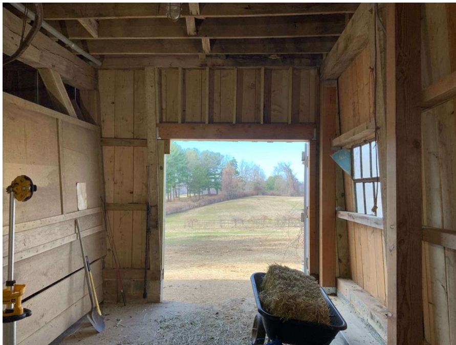
Photo S-100: View looking west down Gridline 1 in the west wing at the newly repaired northwest corner of structure. The new columns are plumb. The original columns are leaning up to 5 degrees to the south.
