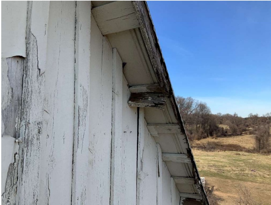
Photo A-5: Close-up view of deteriorated/missing fascia board and lack of edge flashing.
