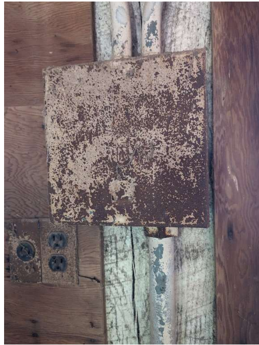
Photo E-11: Cracking/flaking white paint on conduit and junction box located on north barn interior wall. Identified as potential lead-based paint.
