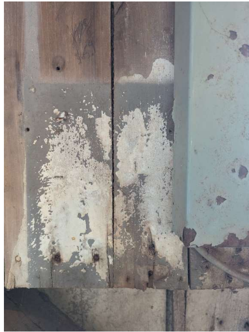
Photo E-9: Cracking gray paint behind apparent former interior electrical panel area on north barn interior wall. Identified as potential lead-based paint.
