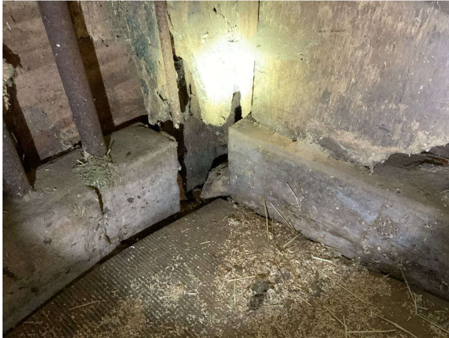
Photo S-107: Bearing loss at Column M/2.5 at grade level (looking northwest).
