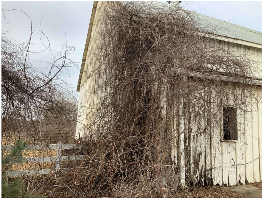
Photo S-113: Heavy vegetation on southwest corner of structure preventing access to Column B/4.
