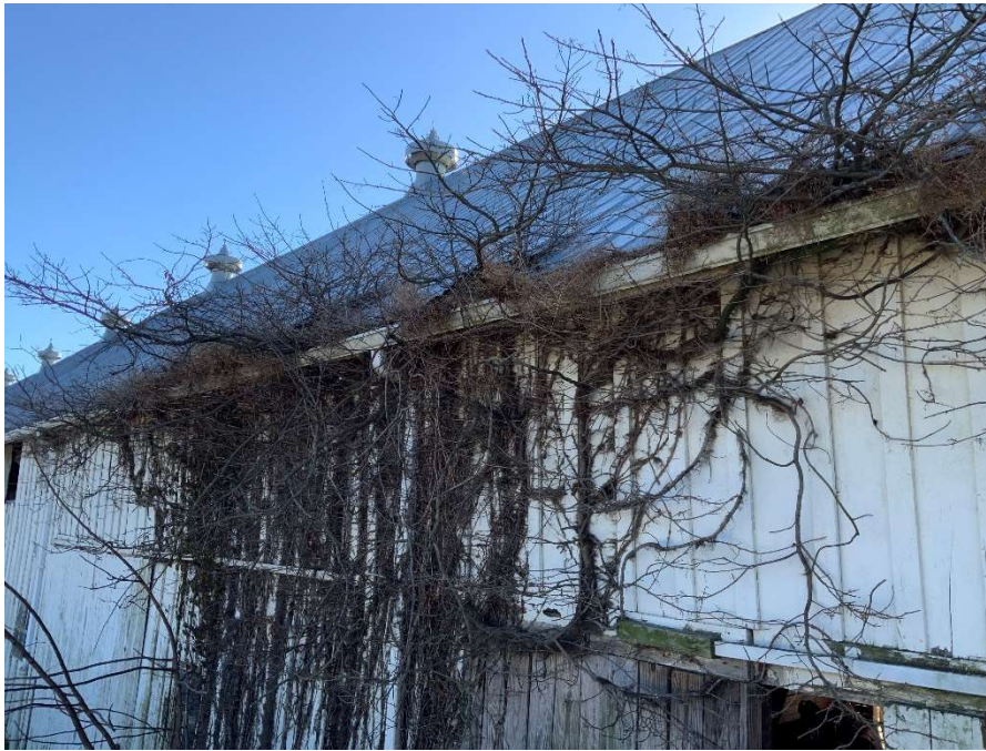
Photo A-15: General exterior photo of vegetation overgrowth and clogged gutters.
