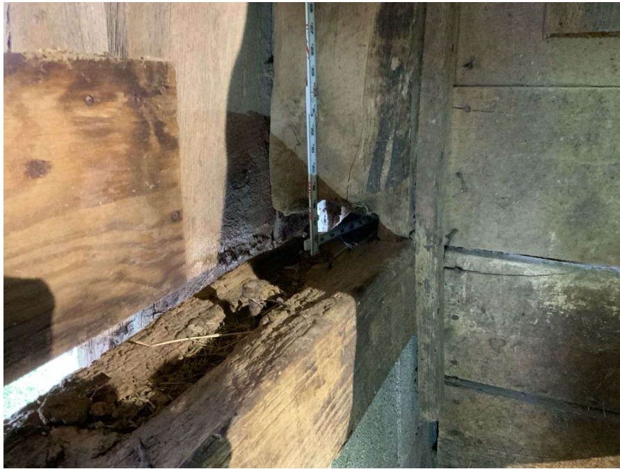
Photo S-109: Bearing loss at Column T/3 at grade level (looking southeast). Supporting sill plate is also rotting.
