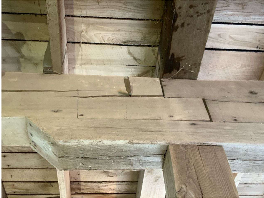
Photo S-73: Split at end of floor beam at bearing location. Floor beam between Column S/2.5 and T/2.5 shown looking south.
