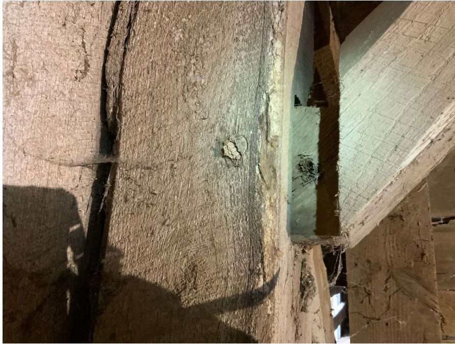
Photo S-129: The west brace at Column T/2 at grade level is not connected to the column at the base connection (looking south). Note the dowel is sheared and the brace is sticking out of the mortise slot.
