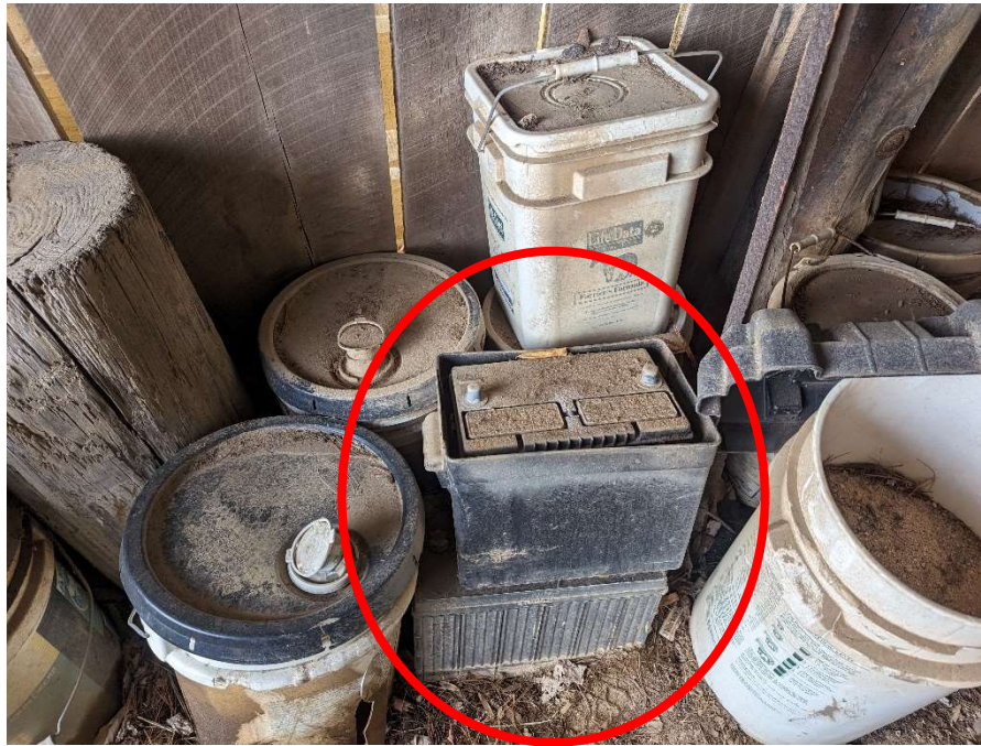
Photo E-15: Lead-acid batteries in plastic battery boxes. Located in garage/outbuilding south of the barn. No leaks were evident.
