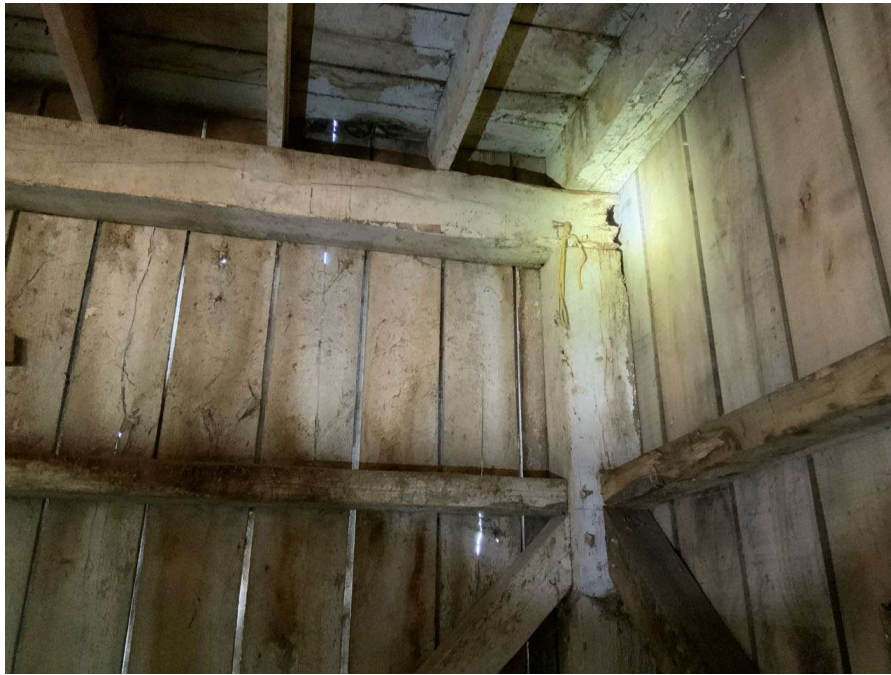
Photo S-89: Rot at east end of floor beam between Columns S/1 and T/1 (looking northeast).
