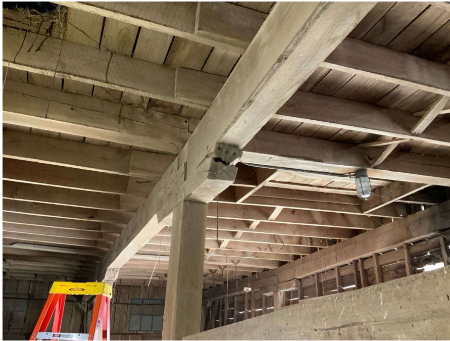
Photo S-95: Split west end of at-grade column cap at Column F/3 (looking east)
