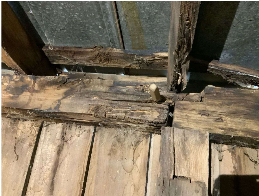
Photo S-21: Roof beam between Columns I/7 and J/7 exhibits rot with full ice pick penetration at west bearing.
