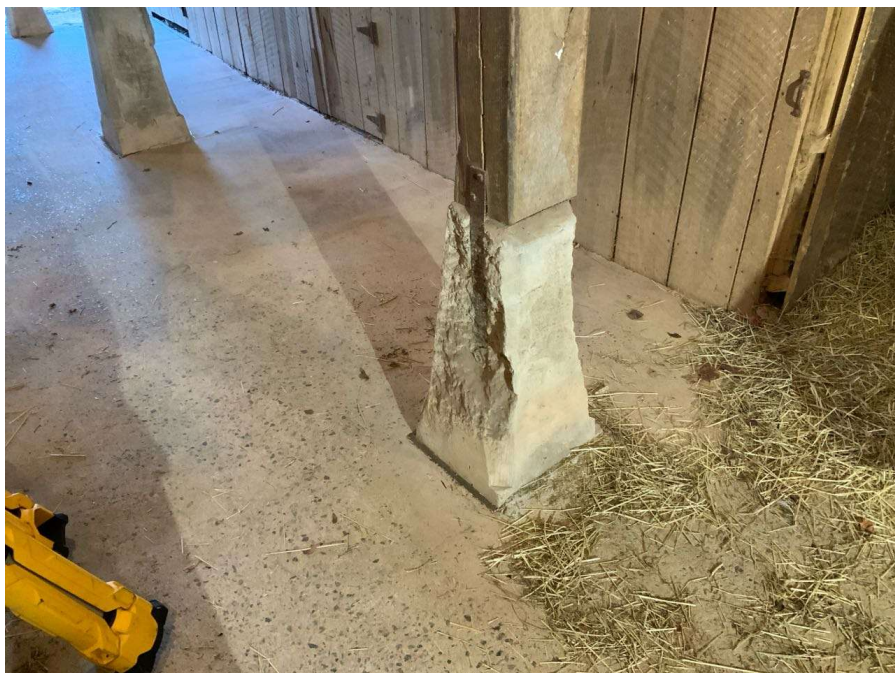
Photo S-156: Typical pedestal with spalled faces exposing the embedded steel straps. Column O/2.5 shown.
