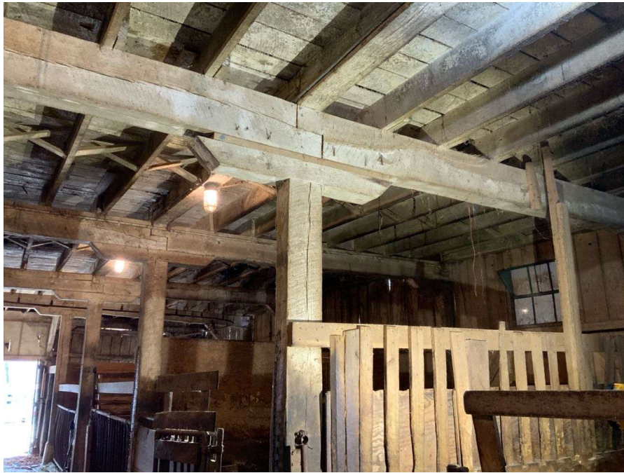
Photo S-79: Shim installed at Column I/3 between the top of the at-grade column cap and bottom of the floor beams (looking south).
