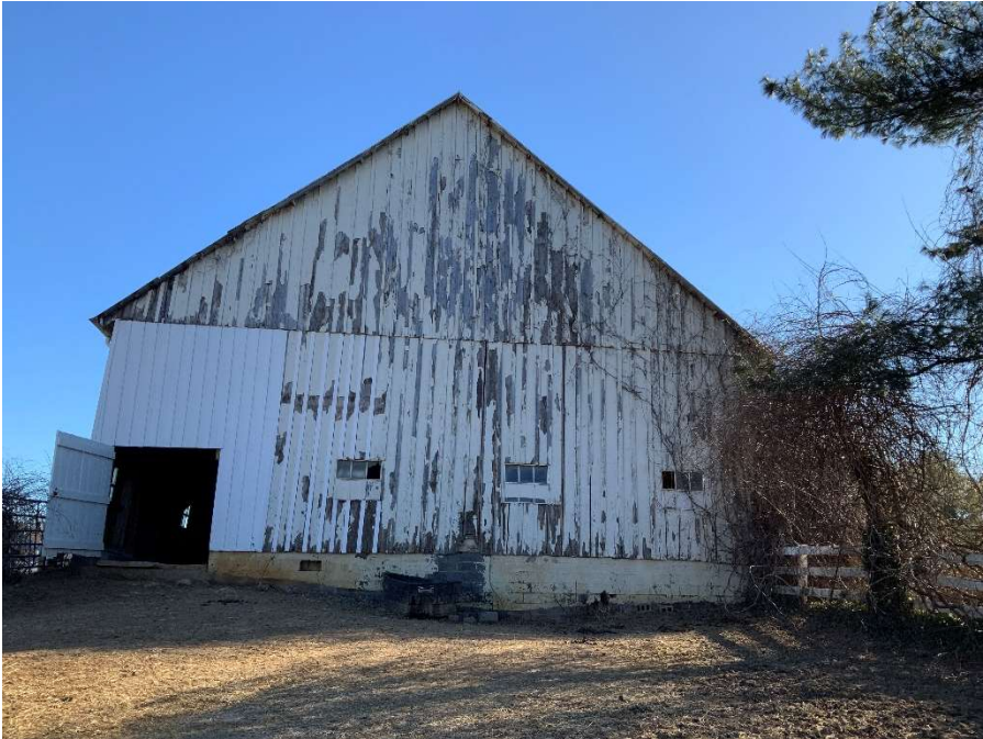
Photo A-9: General exterior photo of paint peeling and deteriorated siding.
