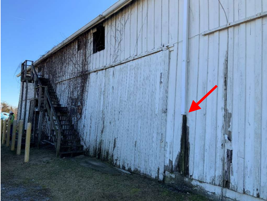
Photo A-14: Deteriorated boards and a discontinuous rain leader.
