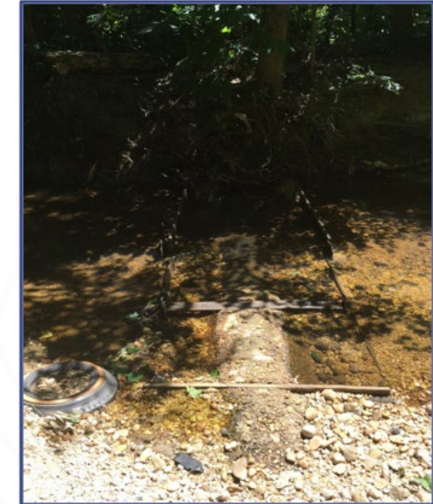
Exposed sewer pipes
