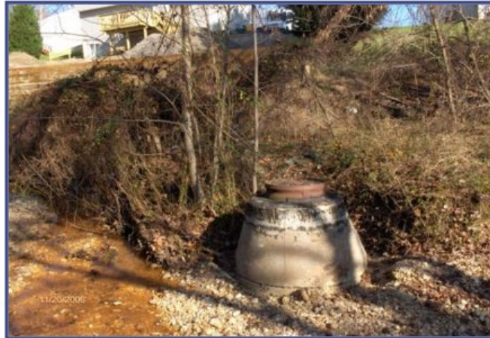
Above grade manhole
