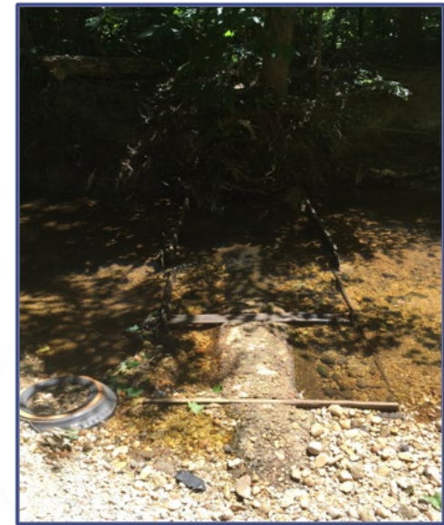
Exposed sewer pipes
